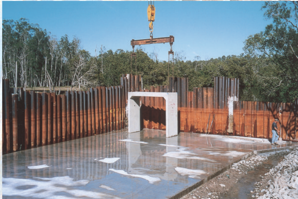
Right: Installation of a Coffer dam to facilitate construction of a roadway over a creek at Coomera.
