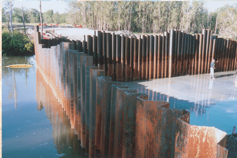
Right: Sheet piling was required to hold back up to 3 metres of water during king tides.
