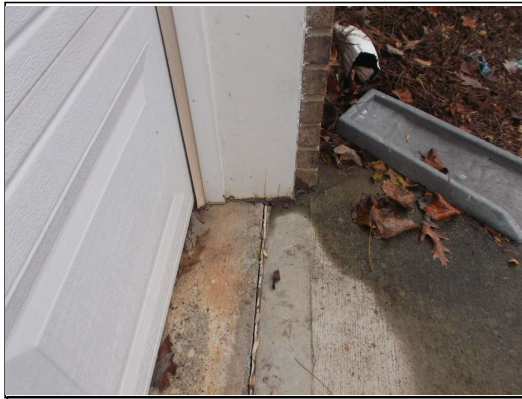
Vehicle door frames contact concrete
