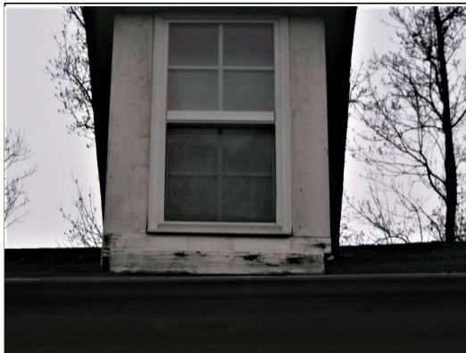
Water damage at dormer trim
