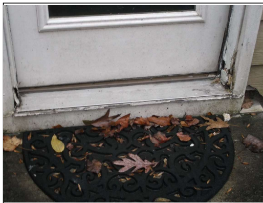
Water damage to rear door frame & threshold
