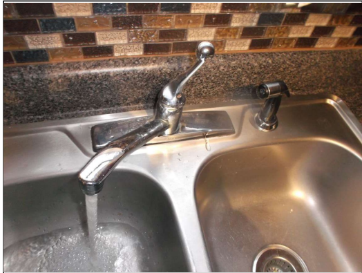
Faucet leaks at handle
