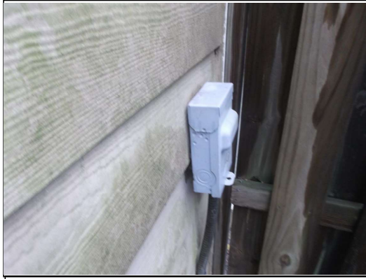
Missing caulk bead at the top of the AC box
