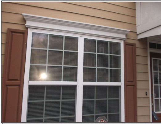
Top window sash fogged
