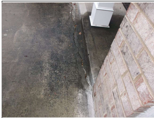
Moderate crack in driveway at front porch
