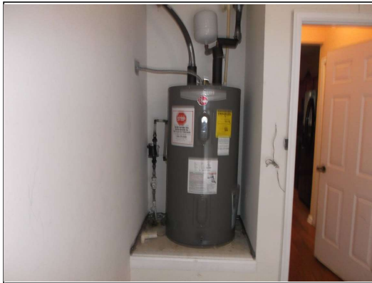
No drain pan under water heater
