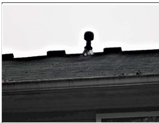
Pipe flashing installed on top shingles nailed?
