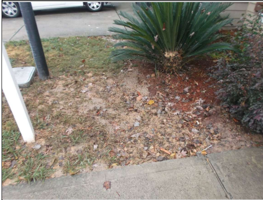
Yard dug up, sink hole, exposed soil
