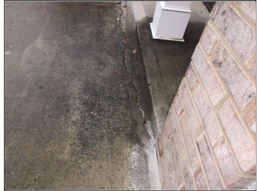
Driveway needs pressure wash
