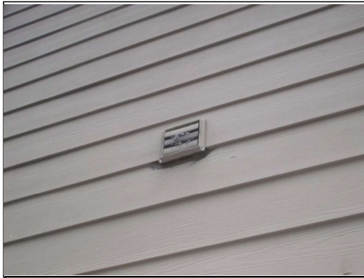
Wrong type of vent terminal for dryer
