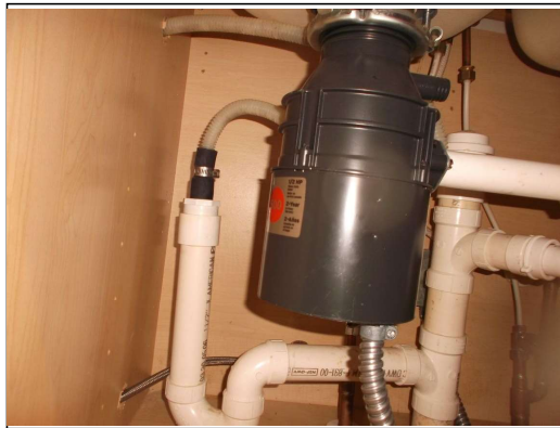
Dishwasher drain pipe not high looped
