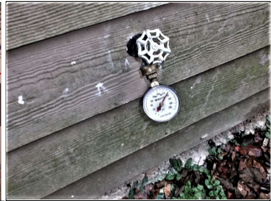
Water pressure 135 psi is very high!
