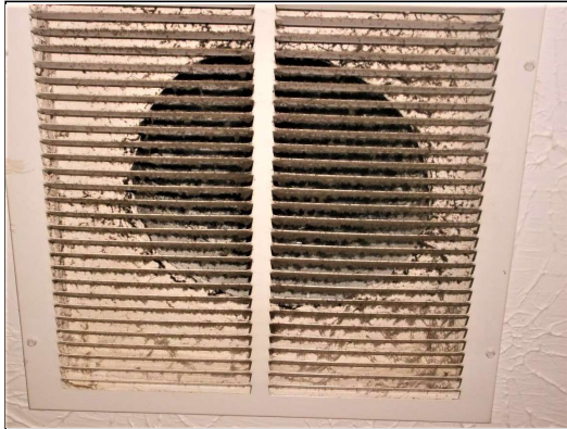
Air duct system dirty and dusty
