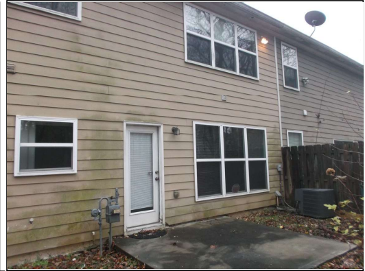
Rear siding and patio needs pressure wash
