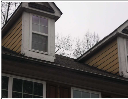
Siding touch roof ans some water intrusion
