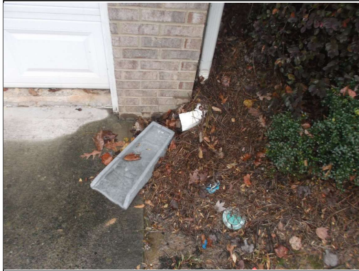
Route downspout away from garage
