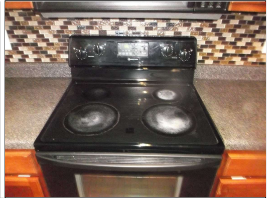
Stove top glass corroded & no anti tilt device
