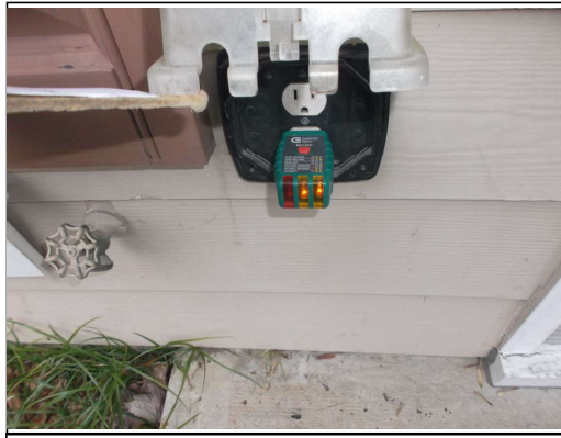
Front and rear outlets not GFCI protected
