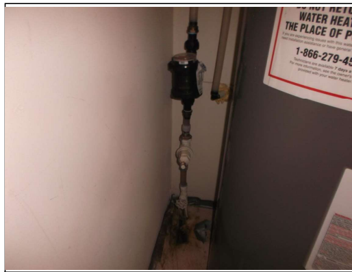
Pressure gauge wet under the bottom (leak?)
