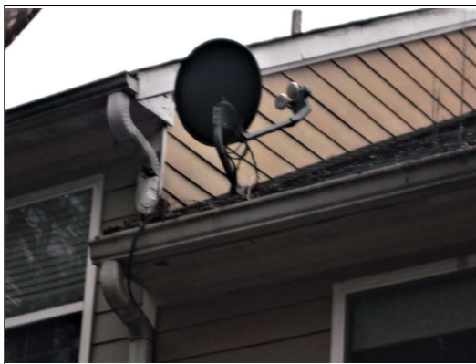
Dish bolted to the roof
