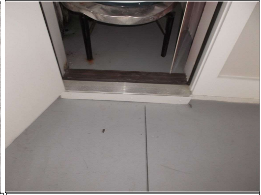
Door threshold not fully supported
