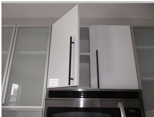
Loose door hinges at wall cabinet
