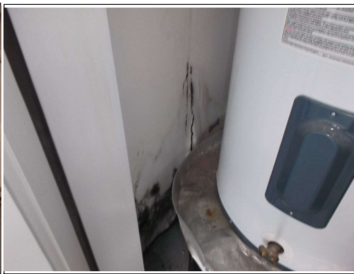
Water in and coming down wall
