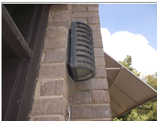
Front light did not illuminate
