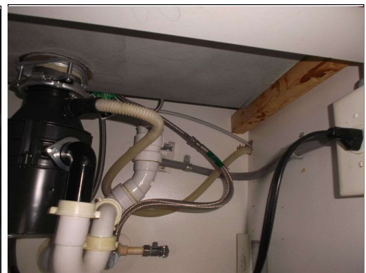
Dishwasher drain pipw not high looped up
