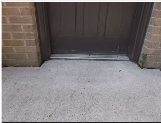
Front door threshold defective
