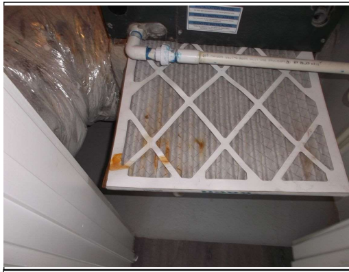
Rust stains on main floor furnace filter
