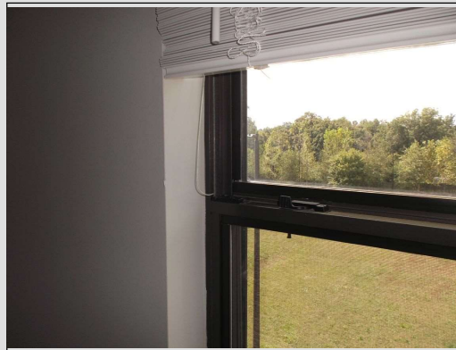
Defective sash cord at rear bed window
