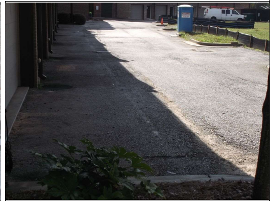
Poor slope and drainage at driveway
