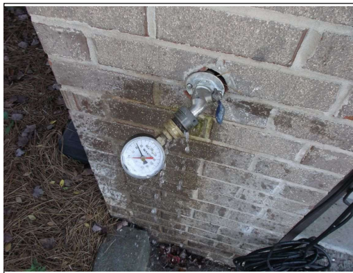
Anti siphon device leaks/hole not sealed
