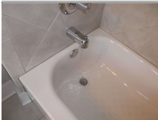
Low water flow at tub spout
