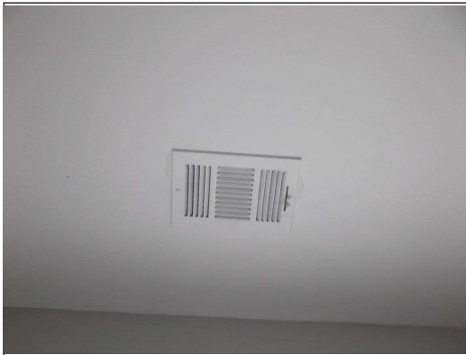
Ceiling stains at rear bed air vent
