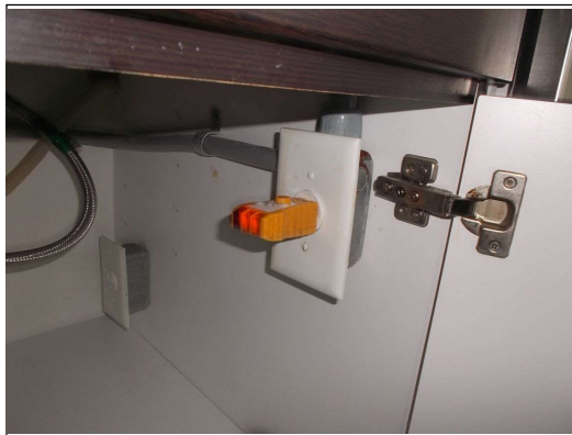
Outlet did not trip when tested
