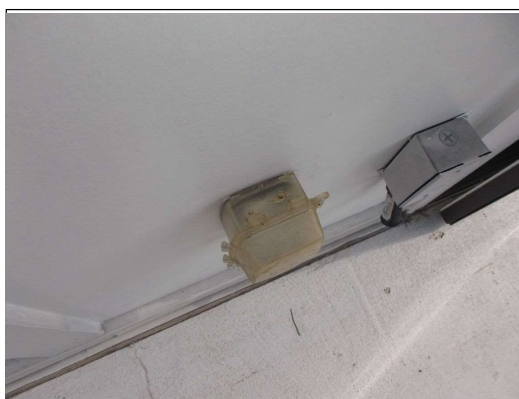
Missing caulk at electrical boxes/box loose
