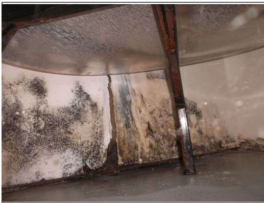
Major water intrusion and damage at wall
