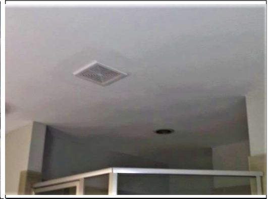
Stains painted over@ master bath ceiling area
