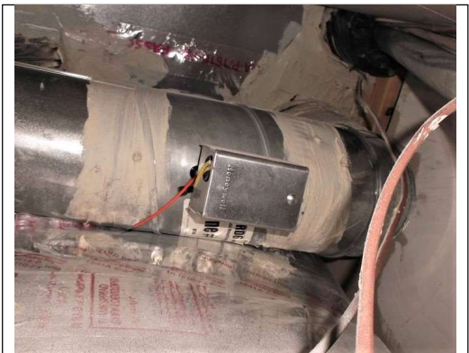
Damper wires not connected to source
