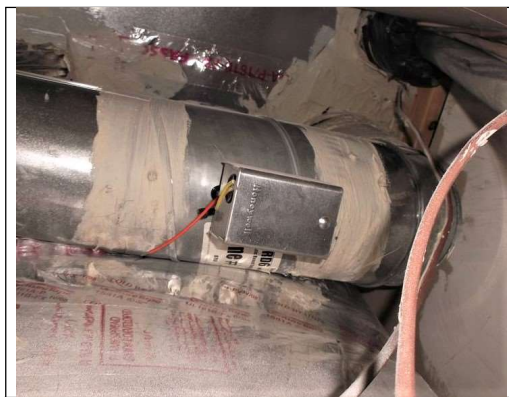
Damper not wired to electrical source
