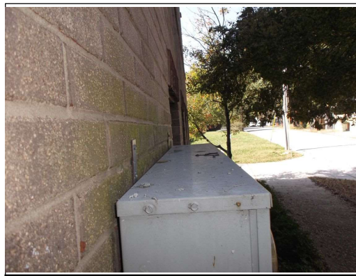
Missing caulk across top of electrical boxes
