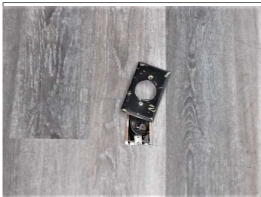
Floor outlet unsafe and defective
