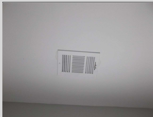
Dry stains at ceiling at vent
