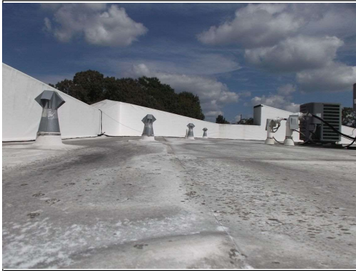
Roof show staining/check laps and seals
