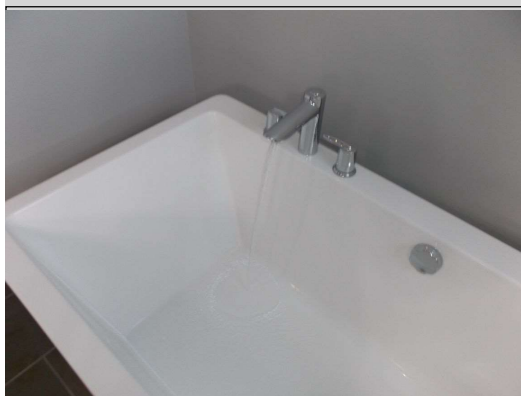
Low water flow at the tub spout
