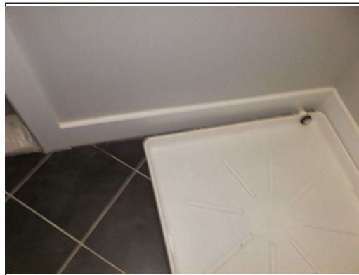
Missing shoe molding at baseboard
