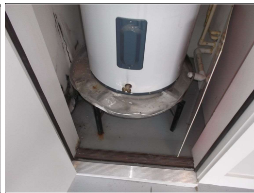
Drain pan bent and crushed
