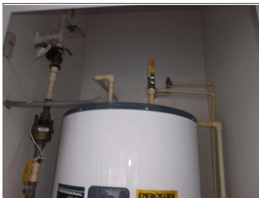
No expansion tank above water heater
