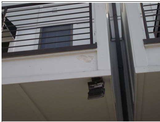
Defective paint at patio floor rim
