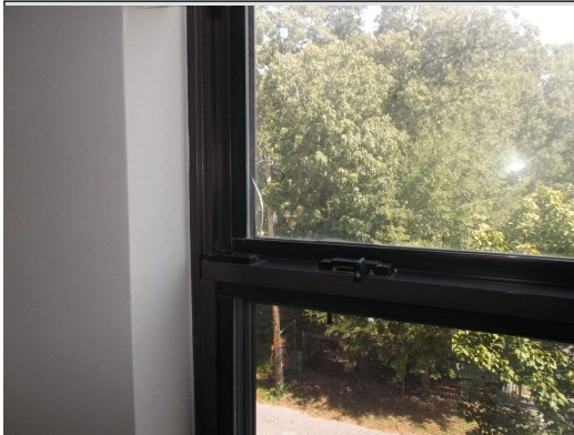
Crack in front bed glass
