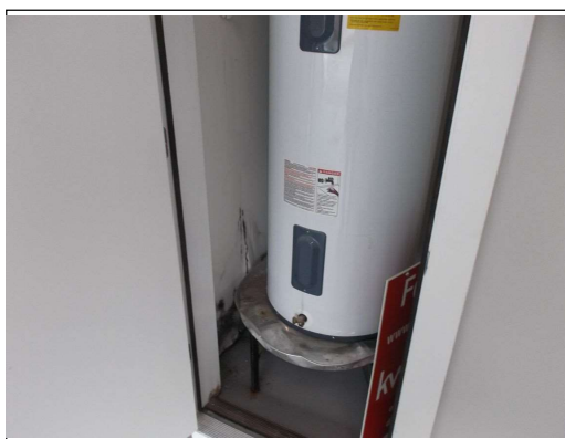
Water leak in wall left of water heater
