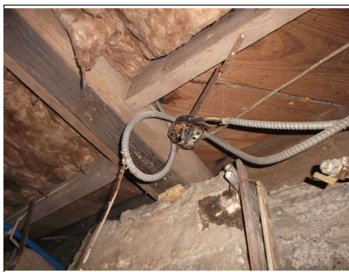
Open junction boxes in the basement
