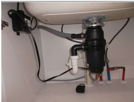
Dishwasher drain pipe not high looped
