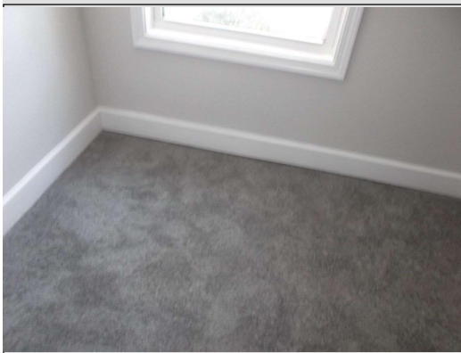
Gap at carpet and floor
