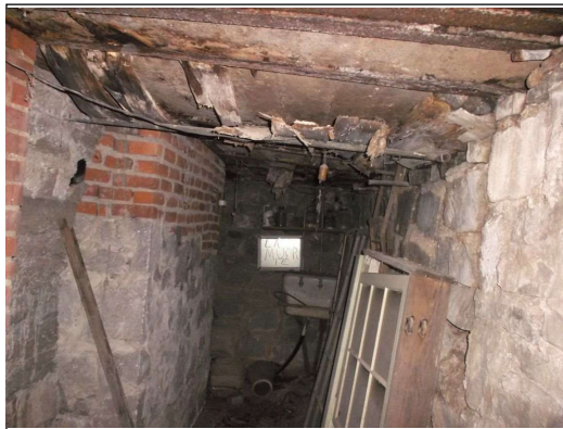
Rotted wood and debris
