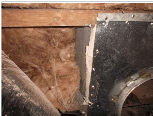
Asbestos tape damaged in basement ceiling
