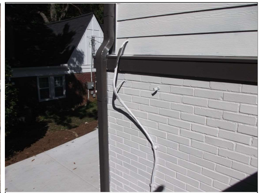
Feeder cable not clamped to brick
