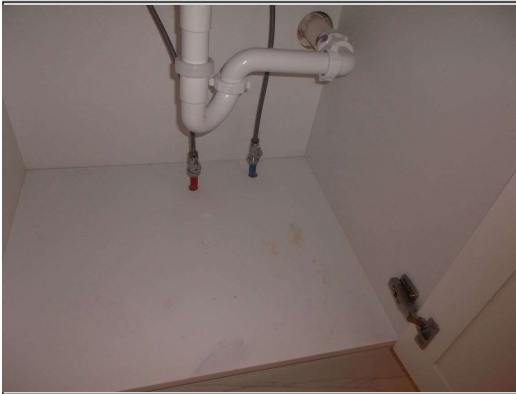
Missing cover plates at pipes in cabinet floor
