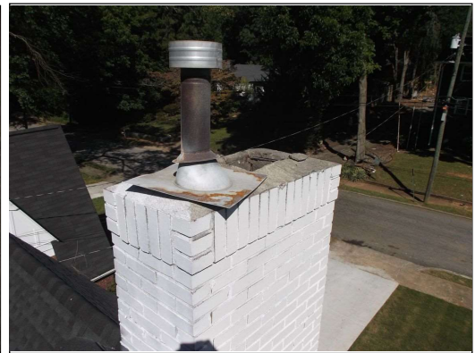
Defective furnace vent pipe atop chimney
