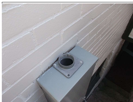
Hole in top of panel box
