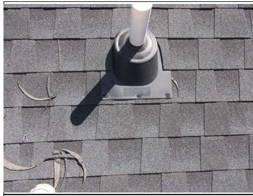
Flashing on top shingles face nailed
