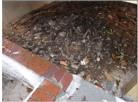
Debris placed under the deck
