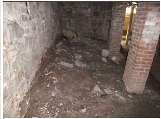
debris and missing moisture barrier
