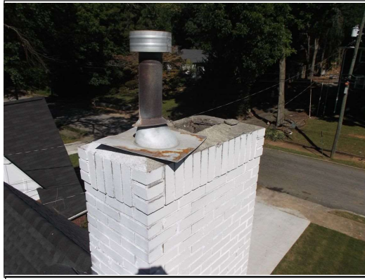
Defective cap, missing screen, defective vent
