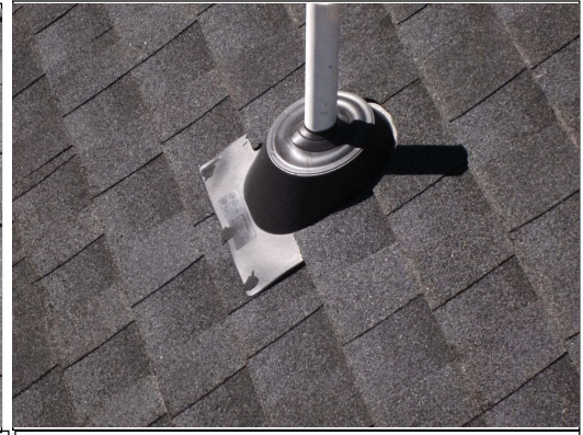
Flashing on top shingles face nailed can leak
