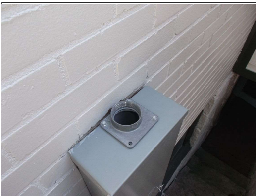
Hole in top of electrical disconnect box
