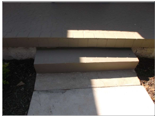
Front steps trip hazard
