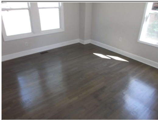
Front bed floor slopes to exterior corner
