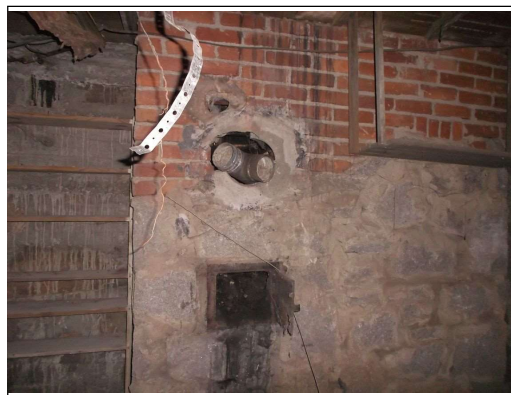
Defective furnace flue pipe assembly
