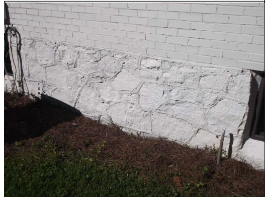
Defective mortar joints in foundation
