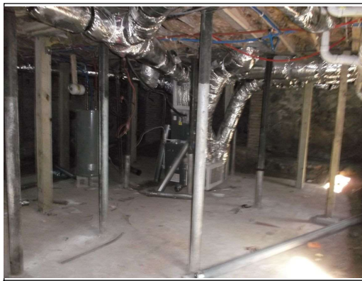
Defective lighting in basement ceiling
