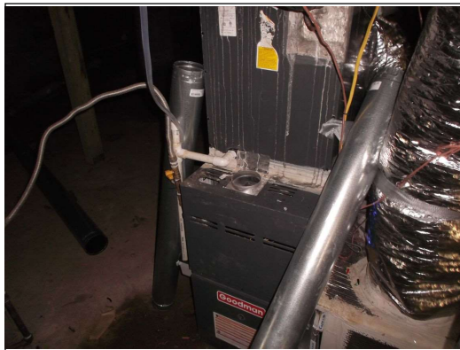
Furnace defective, missing flue, stains
