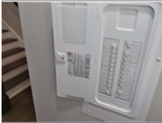
No breaker list inside panel door
