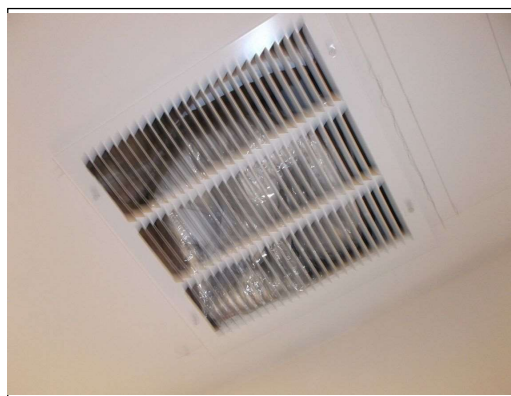
Air duct inside return air register
