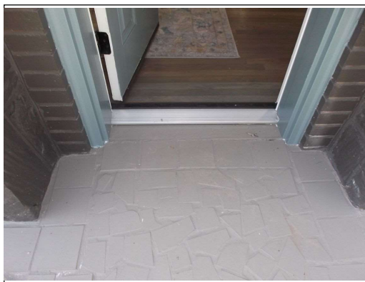
Threshold not supported
