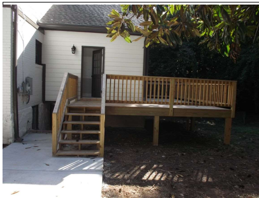
Deck needs corrections several areas
