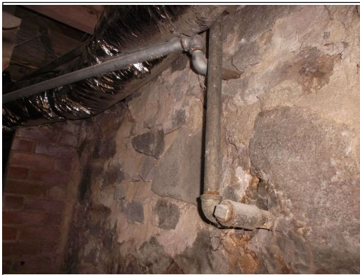
Water pipe for gas
