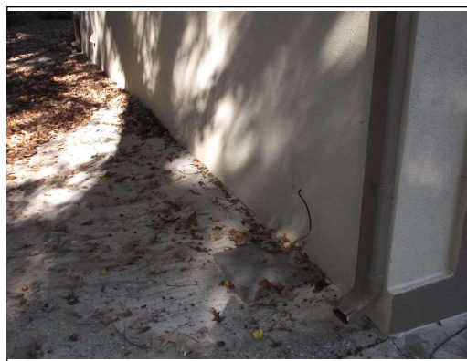
Stucco below concrete can allow termites
