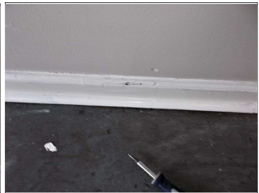
Termite intrusion at baseboard exterior wall
