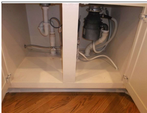
S-Trap and no trap at kitchen sink pipes
