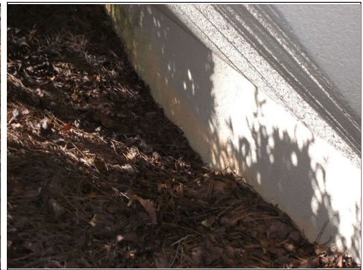
Stucco below soil below front bay window
