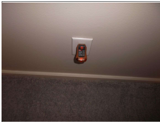
Outlets not energized at master bedroom
