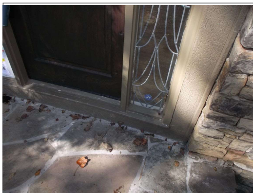
Front door threshold settles on the right
