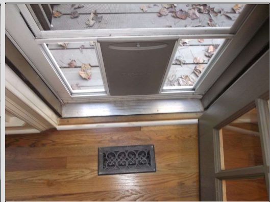
Door frame split at the bottom
