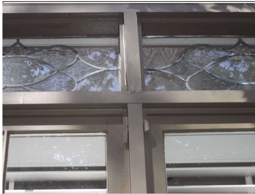
Water damage to living room window frame
