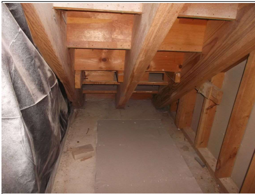
Stairs rest on concrete?
