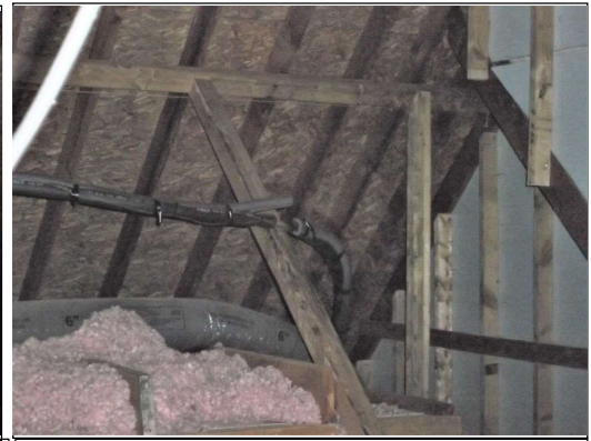
Missing refrigerant line insulation in attic
