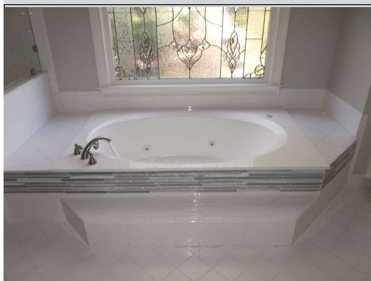
Tiles defective, jets not operating, stopper
