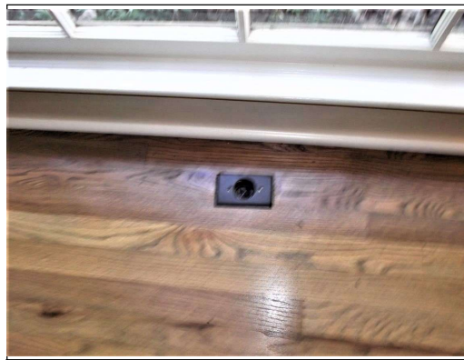
Missing floor outlet covers safety hazard
