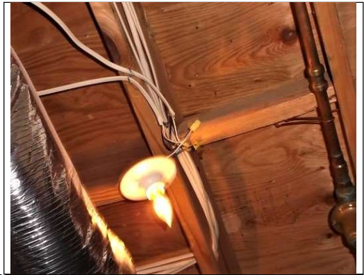
Exposed wire connections at the utility room
