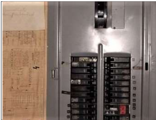
Opening in breaker cover @ panel in basemer
