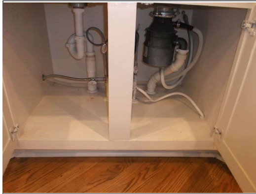
Drain pipes improper and unsafe
