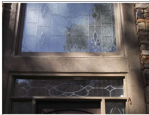
Water damage to foyer window frame
