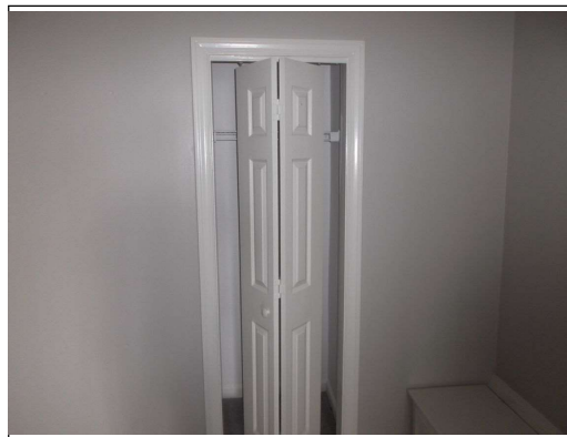
Closet doors defective
