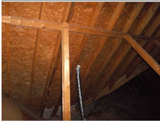
Bath exhaust into attic
