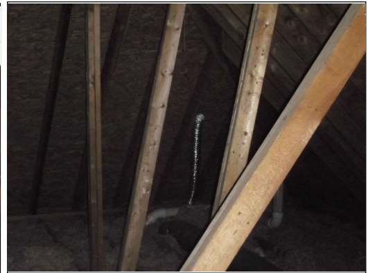
Bath exhaust into attic
