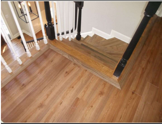
Trip hazard at flooring and top of steps
