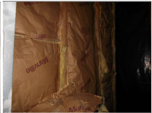
Insulation installed in walls backwards
