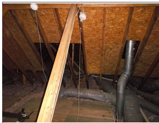
Attic light not illuminating
