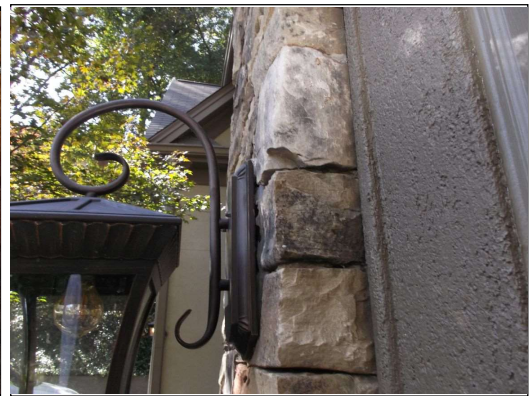
Missing caulk where light attach to walls
