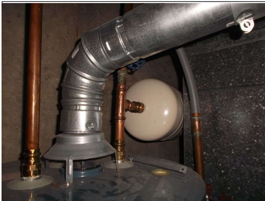
Expansion tank rest on pipe/plastic pipe
