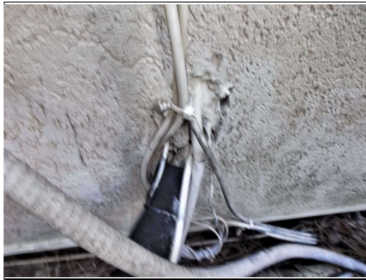
Missing refrigerant line insulation in wall
