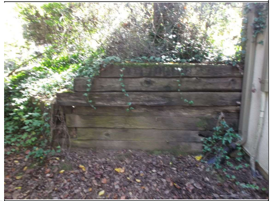
Retaining walls deteriorating
