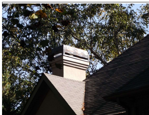
Metal chimney cap needs paint
