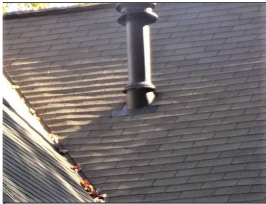
Flashing on top shingles face nailed can leak
