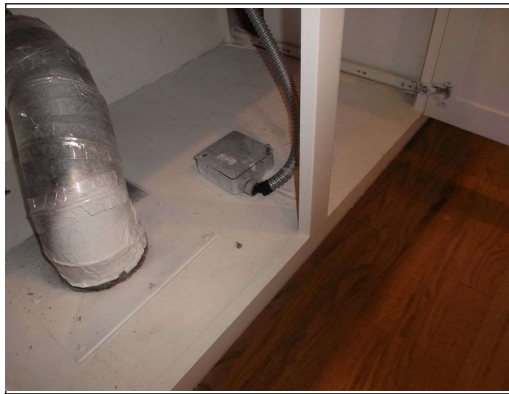
Detached conduit at junction box
