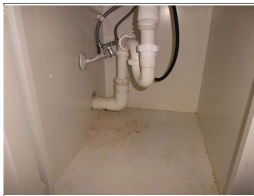
S-Trap in bar sink drain pipe
