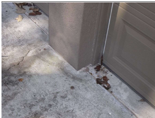
Stucco below concrete can absorb water
