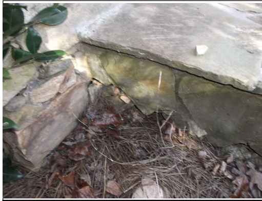
Soil erosion under front porch floor
