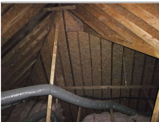
Missing spacer clips between deck panels
