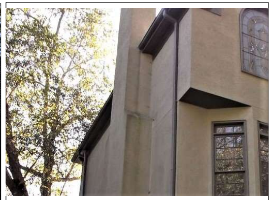
Water stains on stucco from roof or flashing
