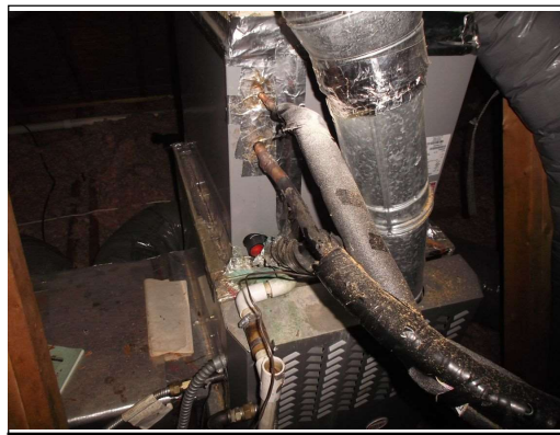
Missing refrigerant line insulation attic furnace
