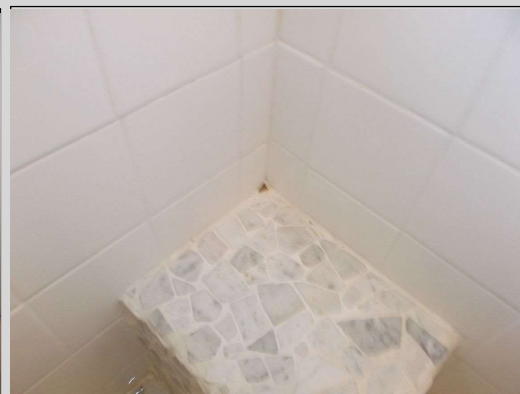
Debris in shower grout
