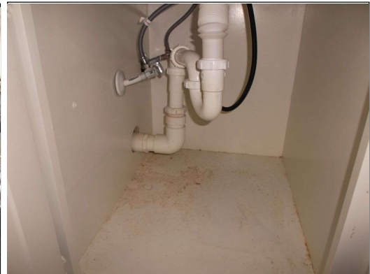
S-Trap at basement bar sink pipes
