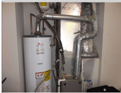
gas vent pipe slopes downward
