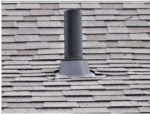
Pipe flashing on top of shingles face nailed
