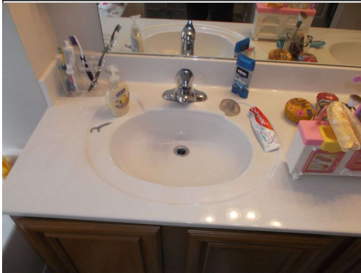
Sink stopper missing
