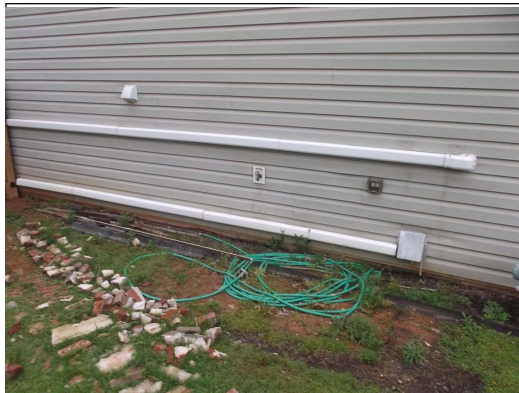
AC units moved from here to back of house
