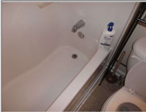
Tub stopper missing
