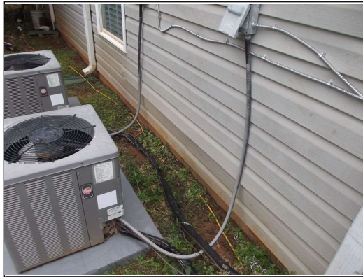
AC electrical conduit not secured to wall
