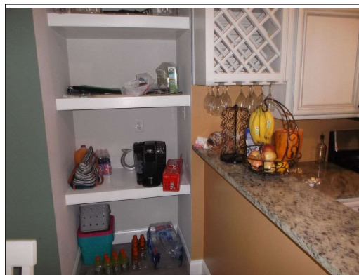
Light switch located in wrong place
