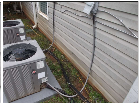
AC conduit not clamped to wall
