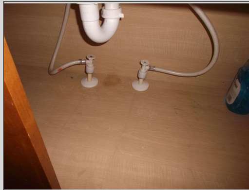
Dry stain on sink cabinet floor
