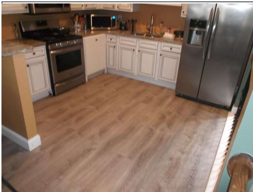
Floor slopes to the sink
