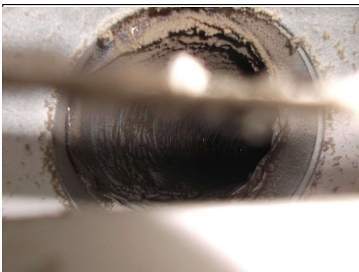
Air ducts are dirty
