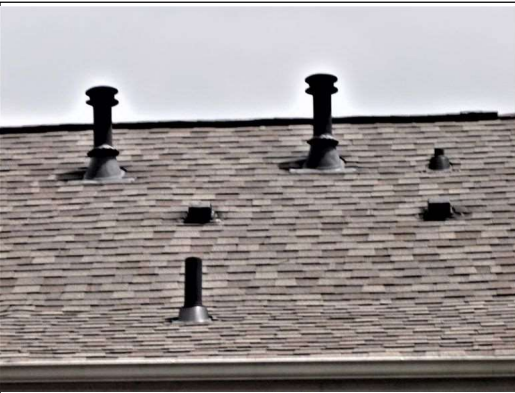
Pipe & vent flashing face nailed
