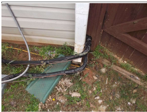
Downspout pours at the rear foundation
