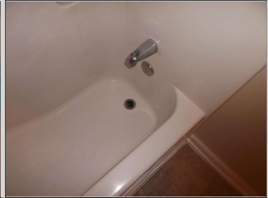
Missing tub stopper
