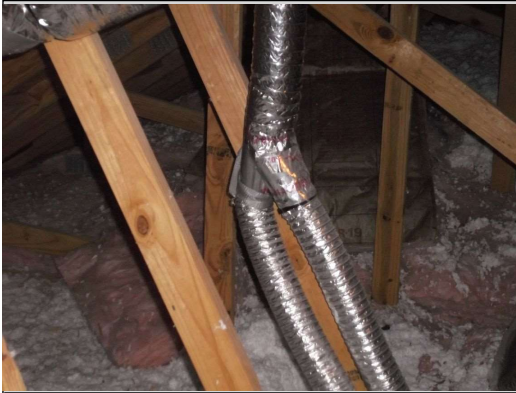
Two bath fan ducts join to one is improper
