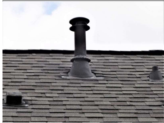
Vent flashing on top shingles face nailed
