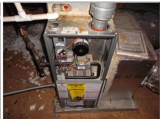
Rust on top of the attic furnace
