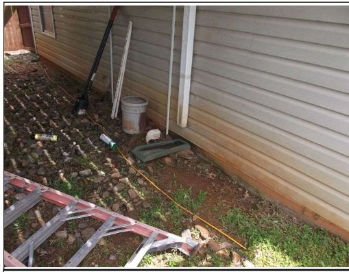
Soil very wet under deck/poor soil slope away
