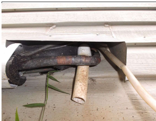
Missing refrigerant line insulation
