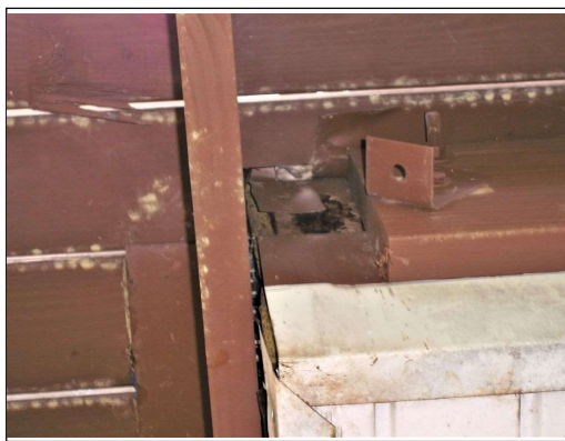
Defective deck floor-to-wall flashing
