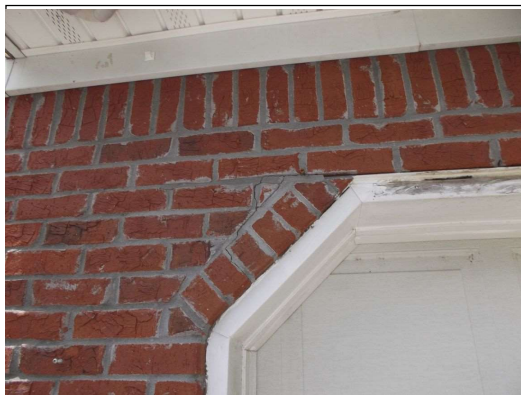
Cracks in brick mortar above vehicle door
