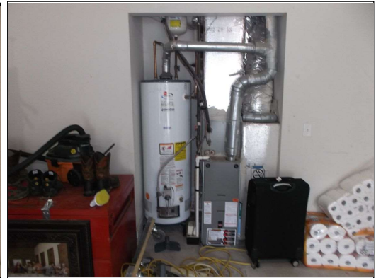
Water heater not 18 in. above garage floor
