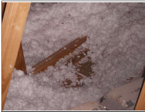
Missing insulation over front bedroom
