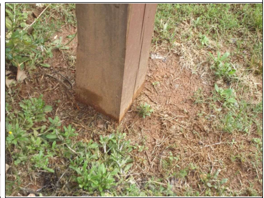
Deck posts contact soil
