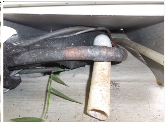
Condensate pipe pouring at siding into soil
