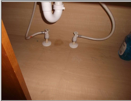
Stain on cabinet floor
