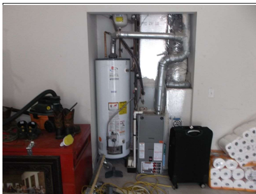
Water heater not raised 18 inches off floor
