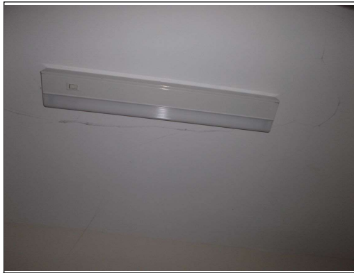
Laundry light not operational
