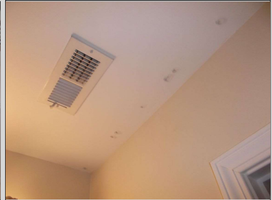
Holes in ceiling over door
