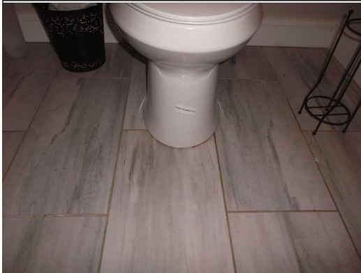
Missing caulk where toilet rest on the floor
