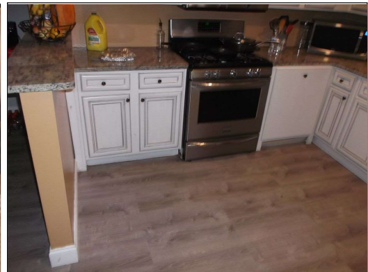
Floor settles at the stove and cabinet
