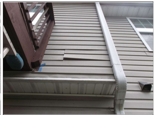
Detaching siding some areas and at deck
