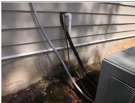
Electrical conduit not fastened to wall
