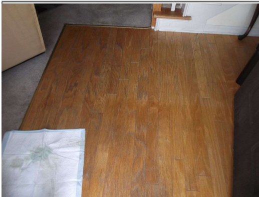
Wood flooring finish worn at front door
