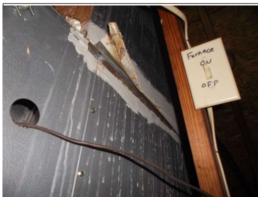
Duct tape & sealant detaching at air handler
