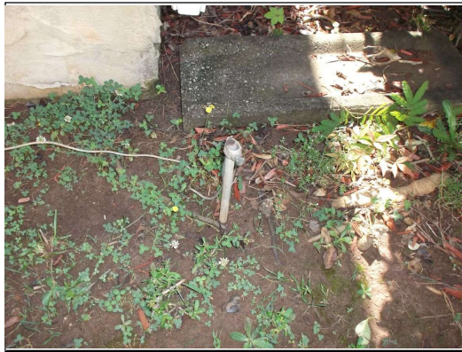
Ground rod not driven all the way in ground
