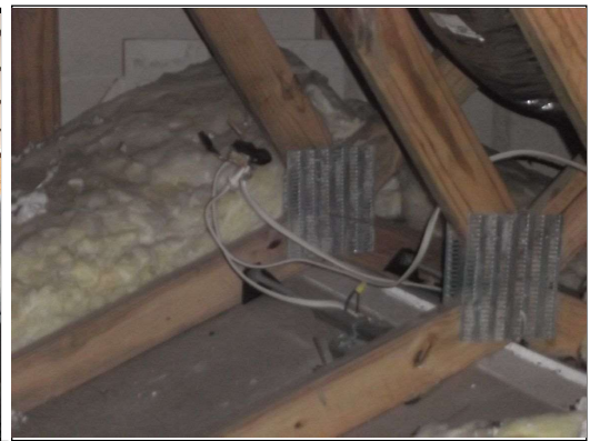
Exposed wire connections in attic
