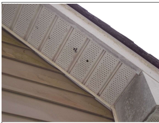
Holes in vinyl soffit left side
