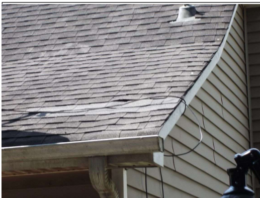
Shingle repair/waves in roof decking
