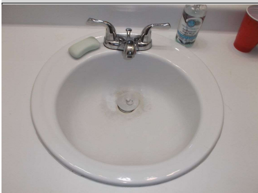
Stains in sink and stopper missing
