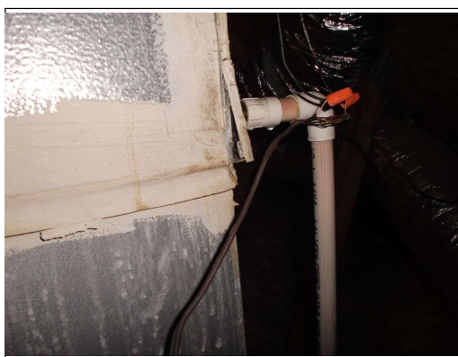
Duct tape detaching at air handler
