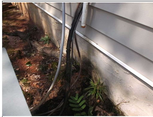
Condensate dripping at the foundation
