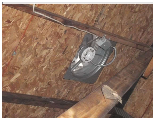
Exhaust fan not operating
