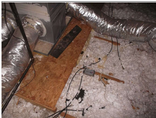
Missing floor at entry and to furnace
