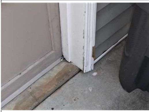
Door frame contact the concrete floor
