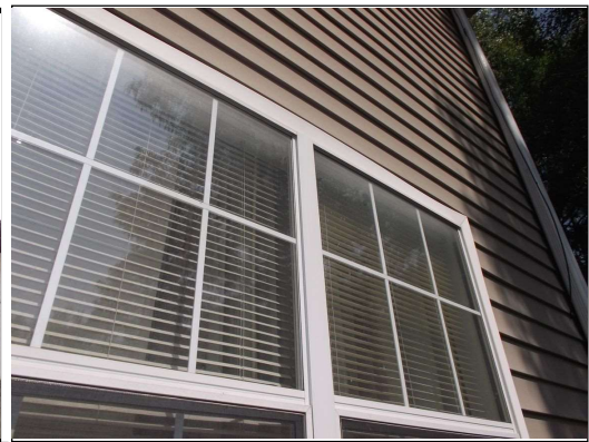
Window glass fogged at front of the house
