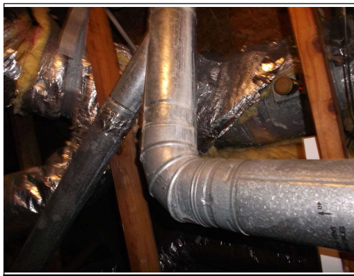
Corrosion on gas vent pipe
