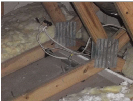
Exposed wire connections in attic
