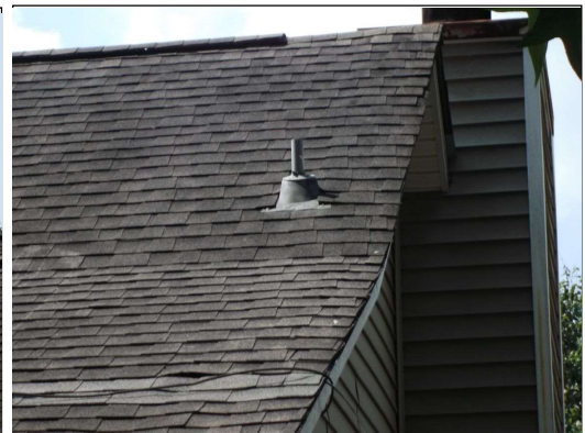
Flashing on top shingles face nail at bottom
