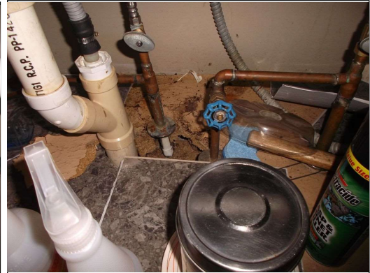
Sink cabinet floor rotted
