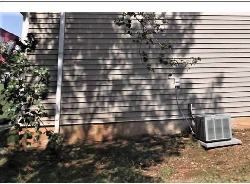
Soil erosion at the right side of the house
