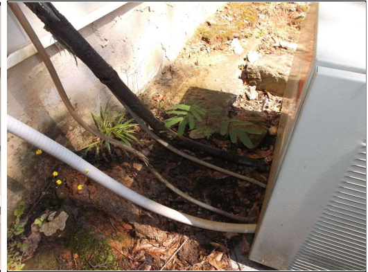
Refrigerant line insulation deteriorated
