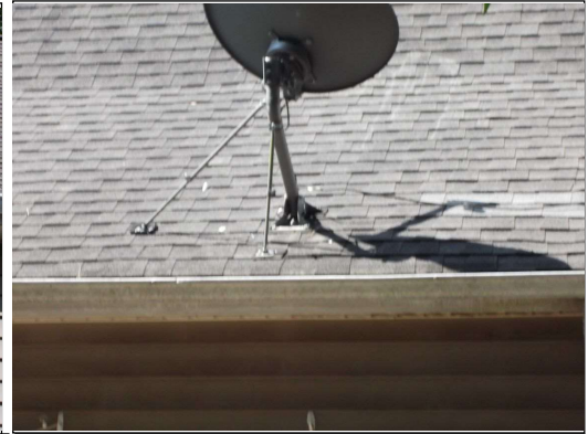
TV dish bolted to the roof can cause leaks
