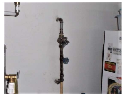
Verify pressure regulator valve not defective
