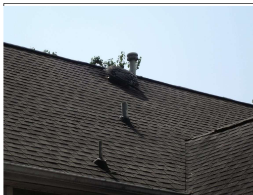
Pipe flashing on top shingles face nailed
