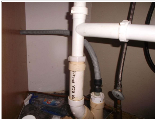
Dishwasher pipe not hi looped up to counter
