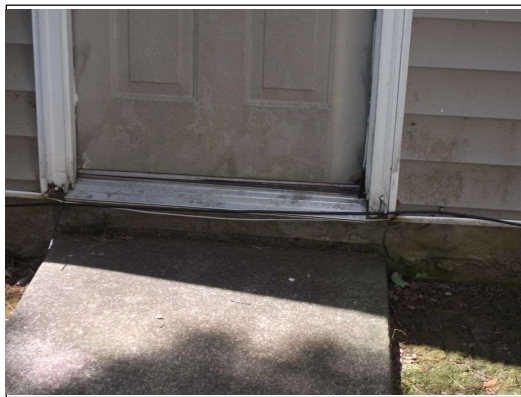
Rear doors rot and water damage
