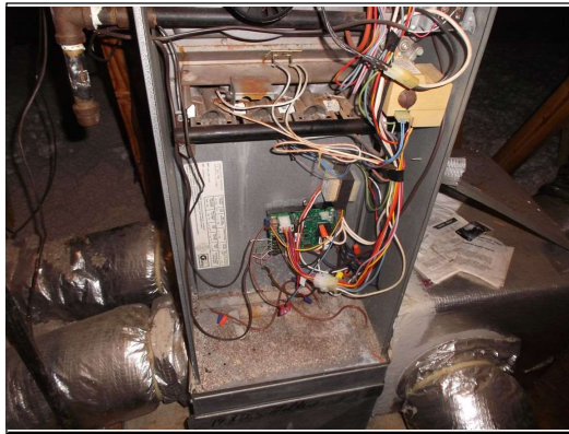
Slight rust and debris in furnace
