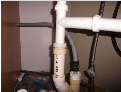
No trap nor vent in sink drain pipe
