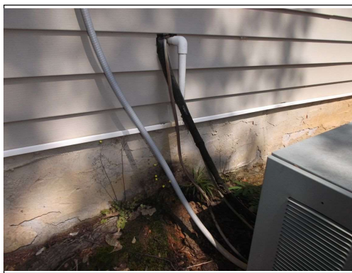
AC electrical conduit not strapped to wall
