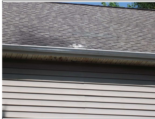
Shingle appears patched at the right side
