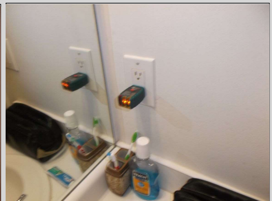
Outlet did not trip when tested
