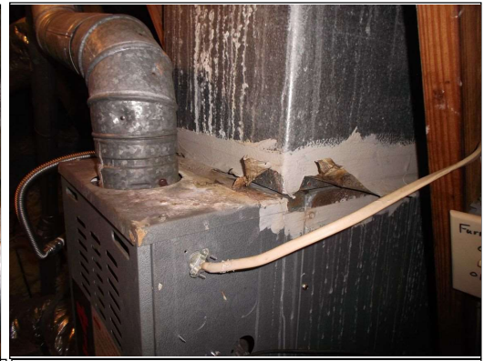
Sealant and duct tape detaching
