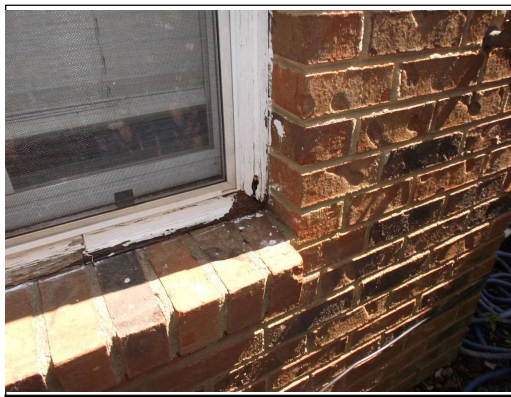
Rot at front window frame
