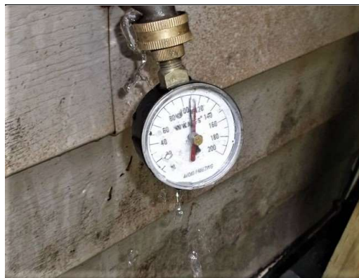
Water pressure 109 psi is too high
