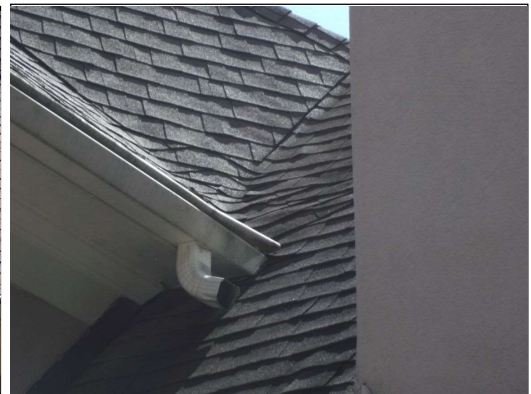
Defective or loose shingles at rear valley
