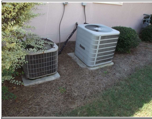
AC units appear original to house
