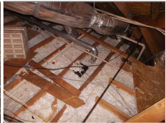
Pipe detached from exhaust fan
