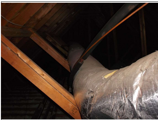
Missing refrigerant line insulation
