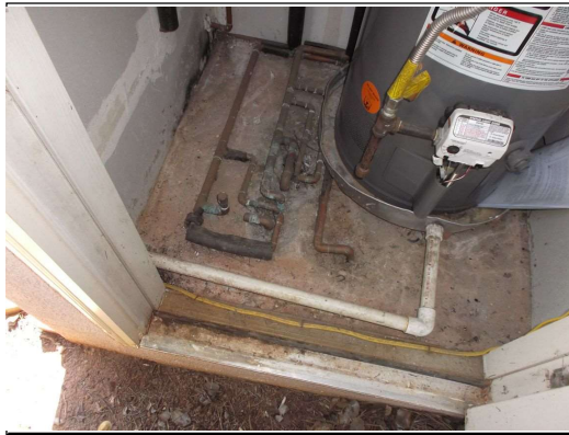
Pipes not wrapped in insulation
