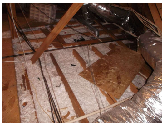
Poor insulation thickness
