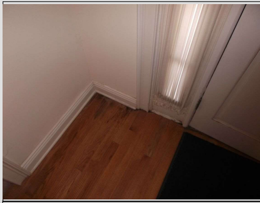
Water damage at foyer floor and wall
