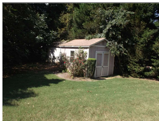
Water damage at storage buildings
