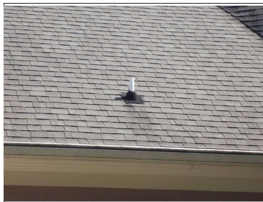
Flashing on top shingles face nailed
