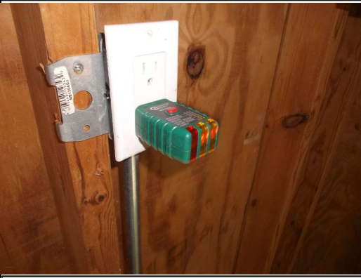
Outlets not GFCI protected at storage bldgs.
