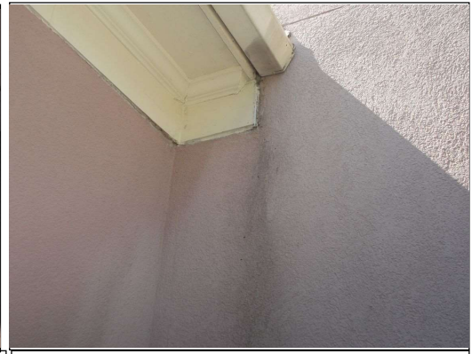
Water enter wall at back of garage
