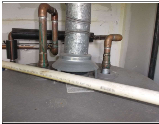
Copper and steel join w/o dielectric fittings
