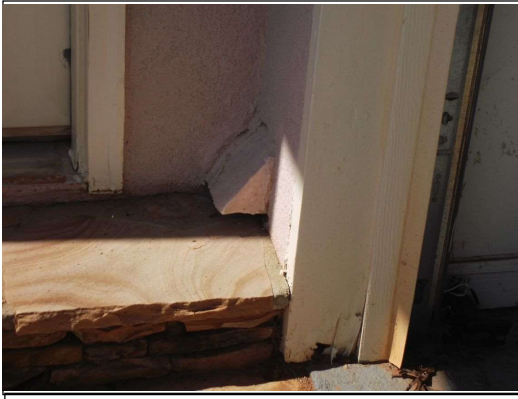
Dryer vent terminal too close to the ground
