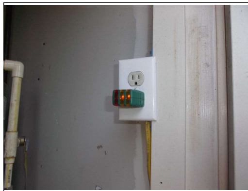
Outlet at water heater closet not GFCI
