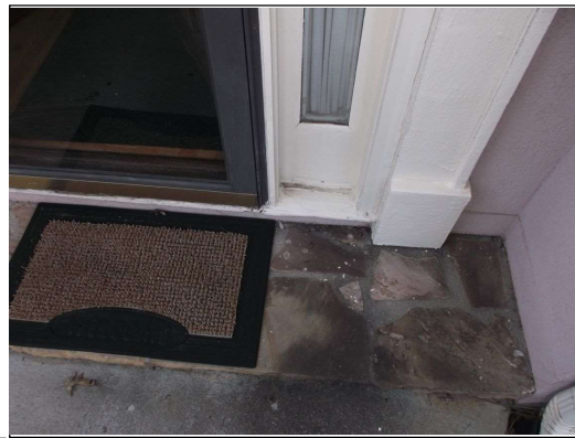
Water damage at front door and in wall
