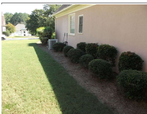
Poor soil slope away from foundation
