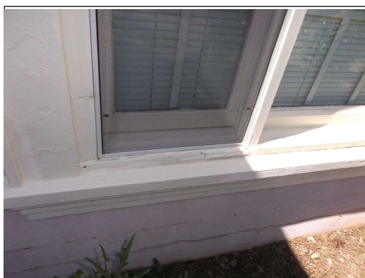
Water damage front and rear windows
