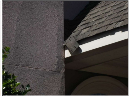
Cracks in stucco and detaching shingles
