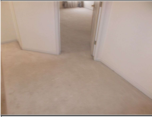
Hall floor slopes to left bed doorway
