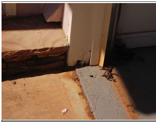
Rot at vehicle door frames at the bottoms
