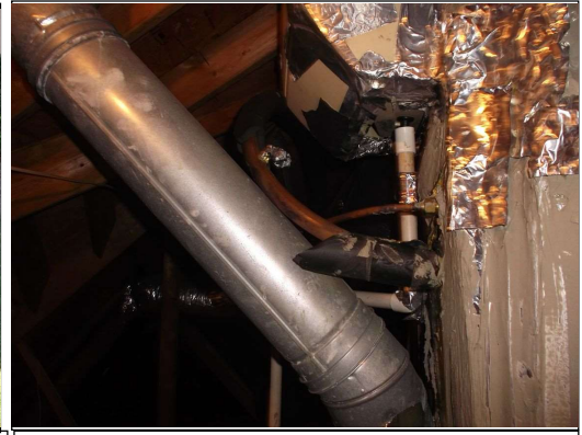
Missing refrigerant line insulation
