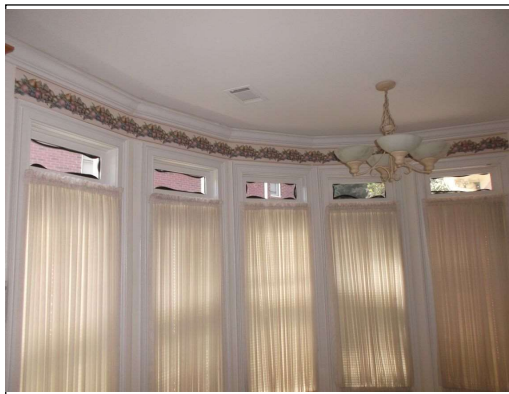
Breakfast room window glass seals broken
