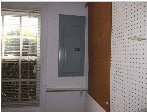
Side wall too close to panel door
