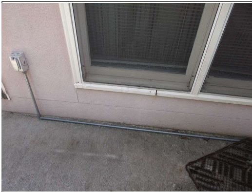
Conduit not fastened to patio or wall
