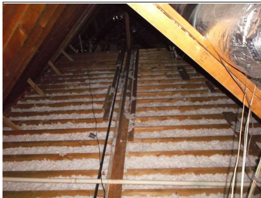
Poor insulation coverage
