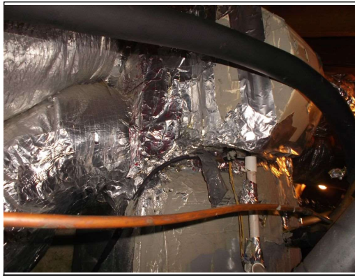
Defective attached dehumidifier
