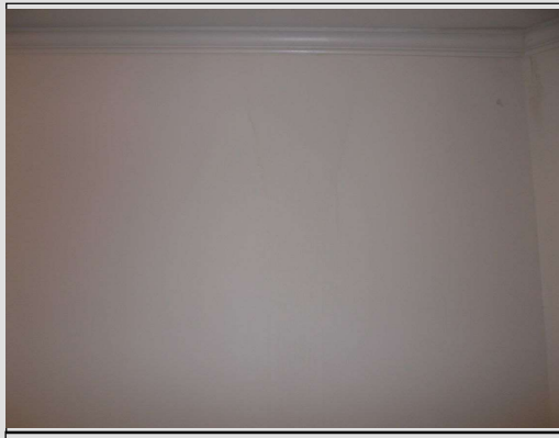
Dry stains on master bed wall
