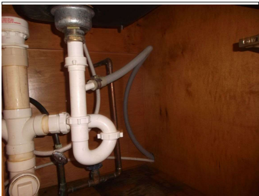
Dishwasher drain pipe not high looped
