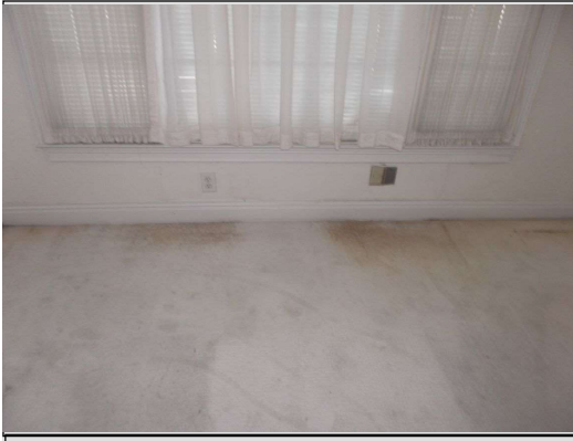
May be water intrusion at front room wall
