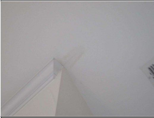
Stains on great room ceiling
