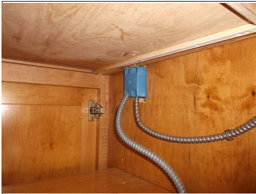
Conduit detaching from electrical box
