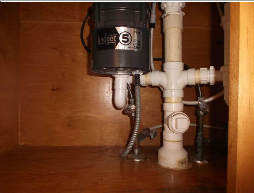
Conduit detached from disposal disposal wor
