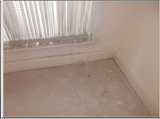
Water damage at great room wall
