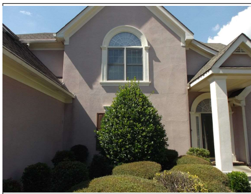
Stucco cracks, trim rot, missing gutter at porch
