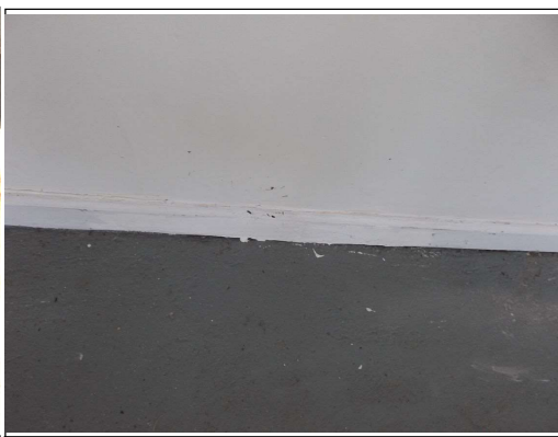
Water damage in garage back wall
