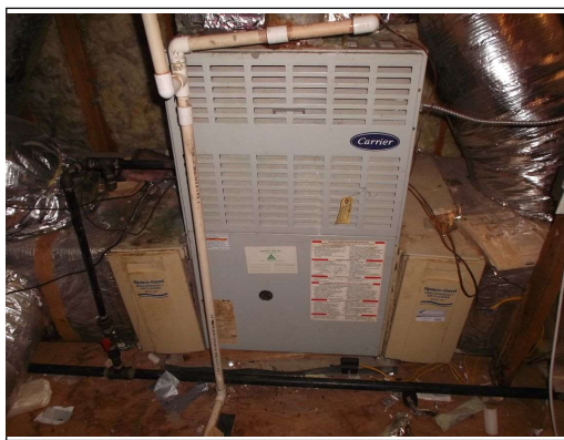
AC units appear original to house
