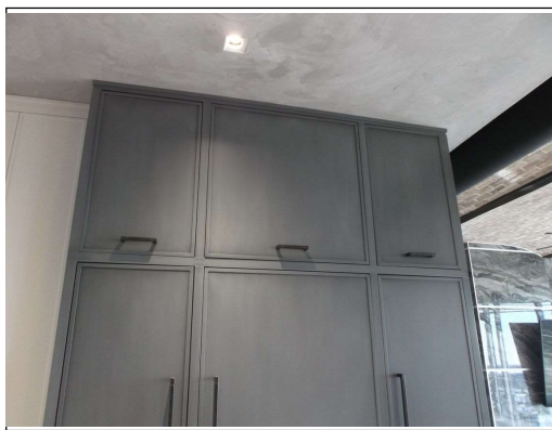
Loose hinges at right wall cabinet door
