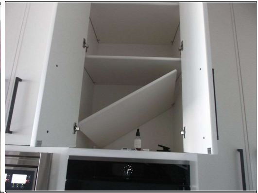
Cabinet shelf detached over coffee bay
