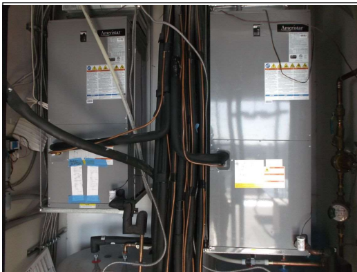
Furnaces located in the hall closet
