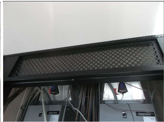
Verify return air screen has been cleaned
