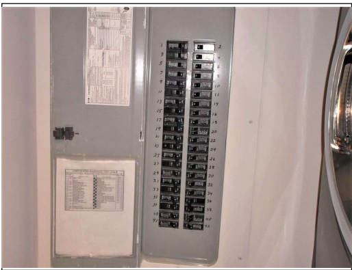
More than 6 breakers in panel no main switch
