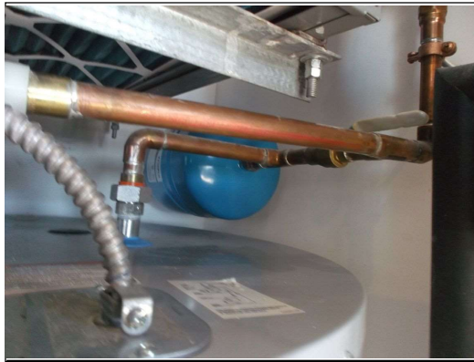
Expansion tank resting on the water pipe
