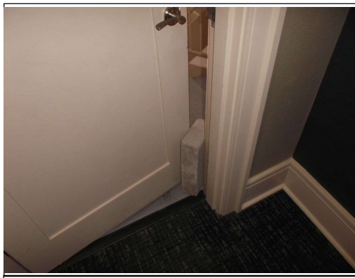
Stairwell door propped open with a block
