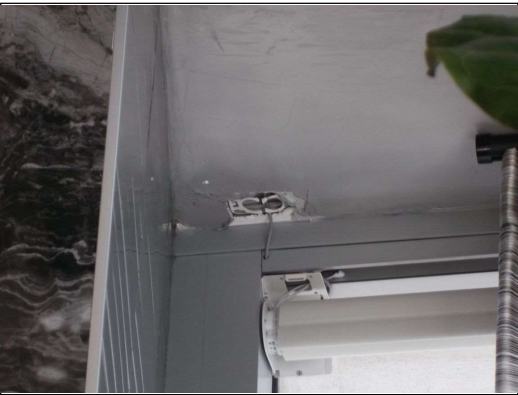
Open outlet box in Living room ceiling
