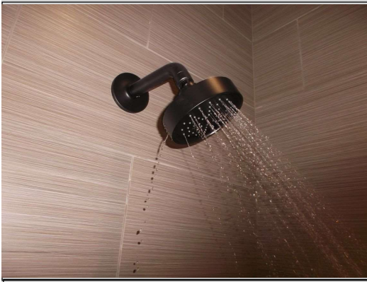
Shower head leaks at the fitting
