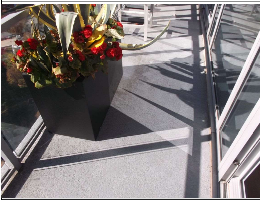
Stains in the balcony floor paint finish
