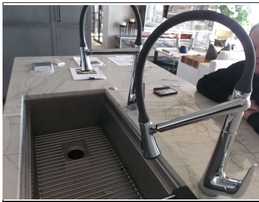
Faucets loose at the body
