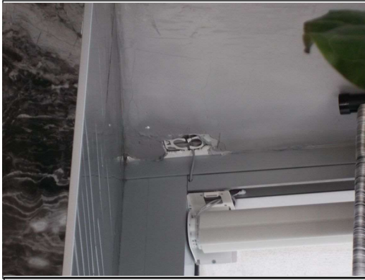
Missing fixture or cover to right of fireplace.
