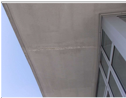
Crack in balcony ceiling
