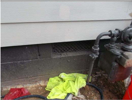
Defective foundation vents several areas
