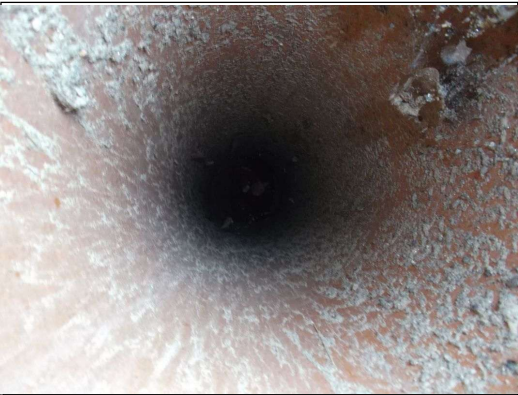
Open waste pipe riser front yard
