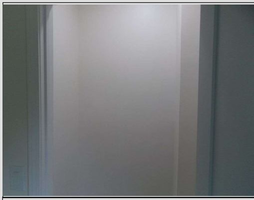
Missing closet shelves
