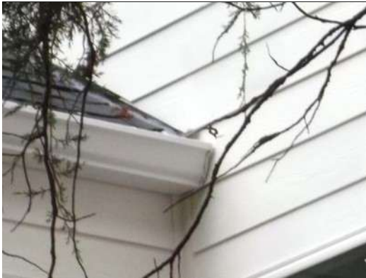
Flashing improperly kicked out
