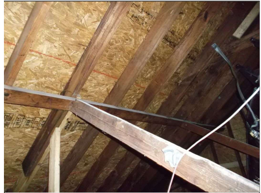
Missing spacer clips between roof panels
