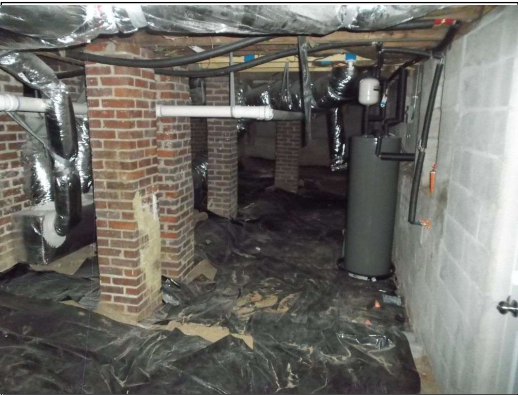
Cannot inspect water heater, door locked
