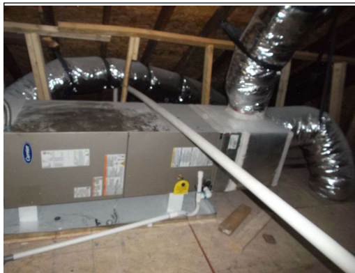
Single stud purlins should be double studs
