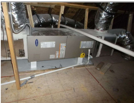
No drain pipe connected to drain pan
