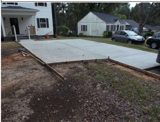
Driveway on ground, not angled, not finished
