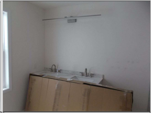
Mirror and hardware not installed
