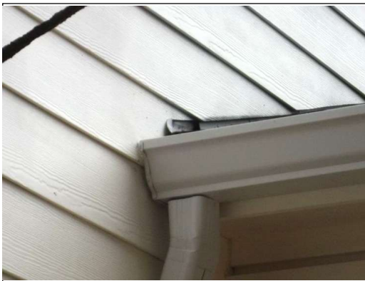
Flashing not extended, kicked out far enough
