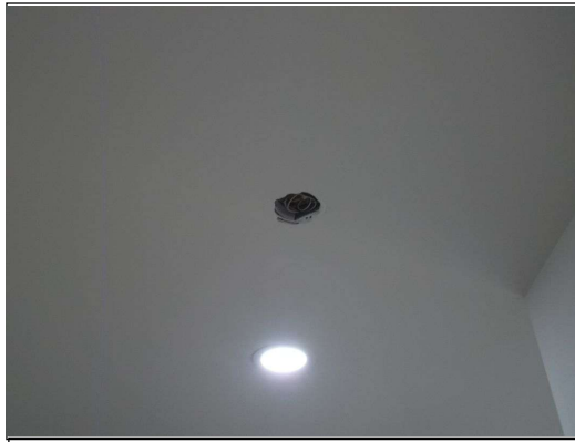
Missing fixture at hall ceiling
