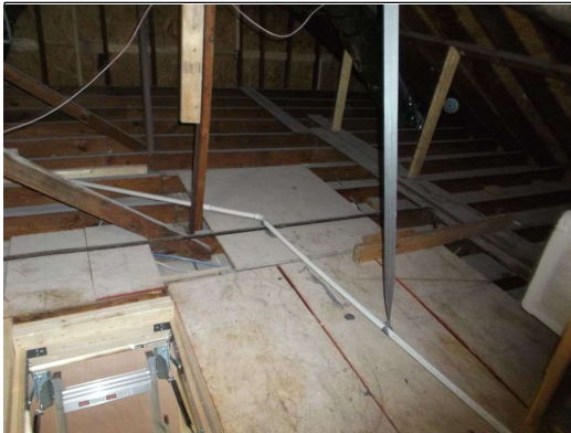
Single stud purlins, missing insulation
