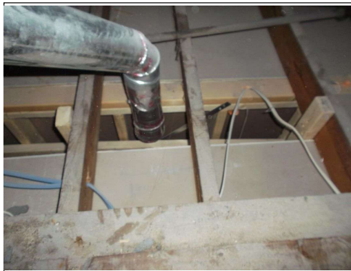
Open chase, vent pipe touch wood
