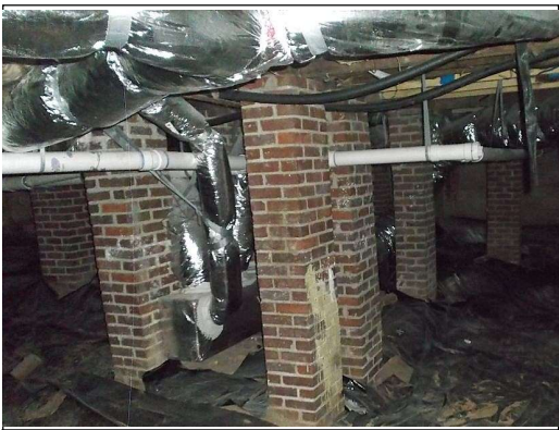
Waste pipes supported with metal straps
