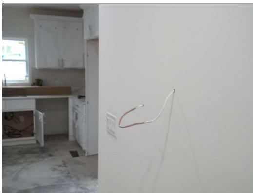
Thermostats not installed
