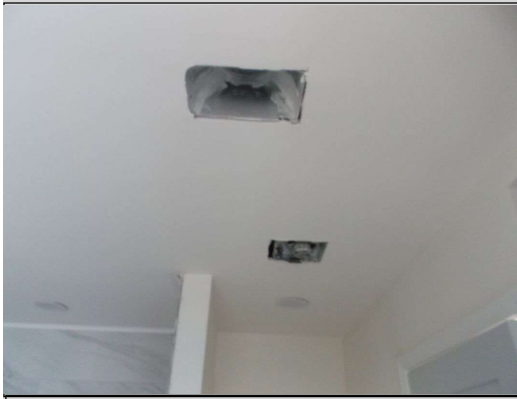
Vent covers not installed
