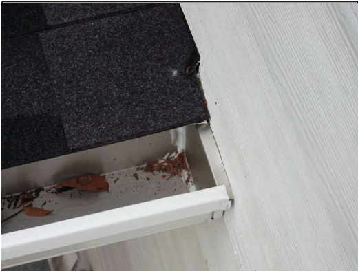
Flashing not kicked out properly
