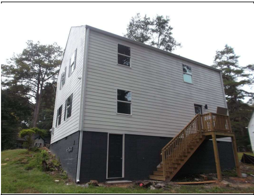
Defective paint, spouts pour at foundation
