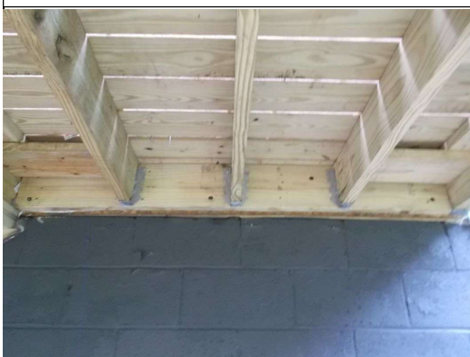
Missing bolts, missing flashing
