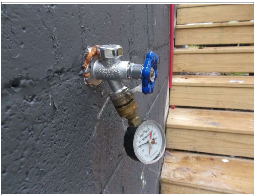
Defective valve rear hose faucet, leaks
