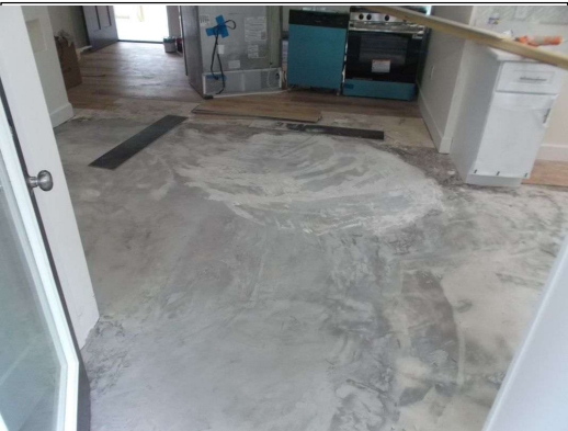
Kitchen floor and trim not finished
