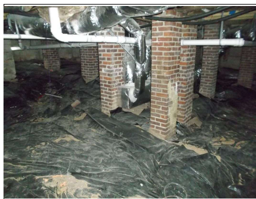
Cannot fully access furnace in basement
