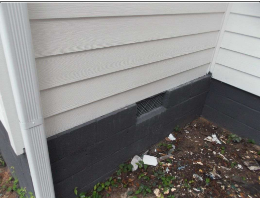
Siding set back from foundation, debris
