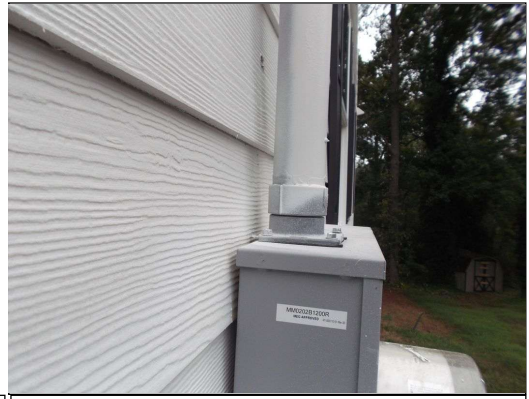
Missing bead of caulk over meter at siding
