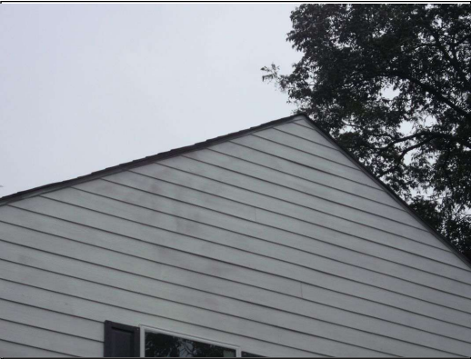
Defective paint many areas around the house
