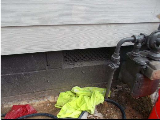
Defective foundation vents at areas
