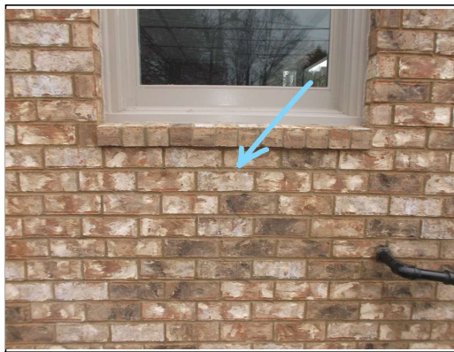
Cannot see plastic flashing in mortar
