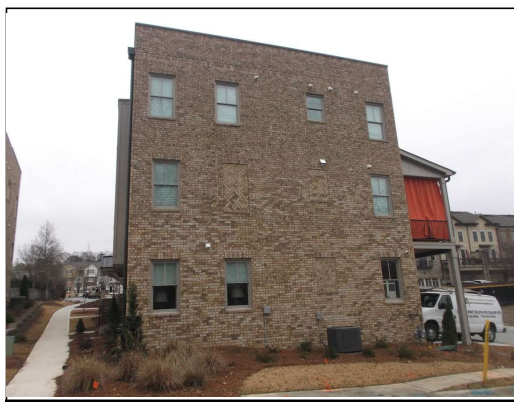
Cannot verify control joints in veneer @ side
