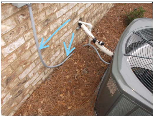
AC conduit not clamped to brick
