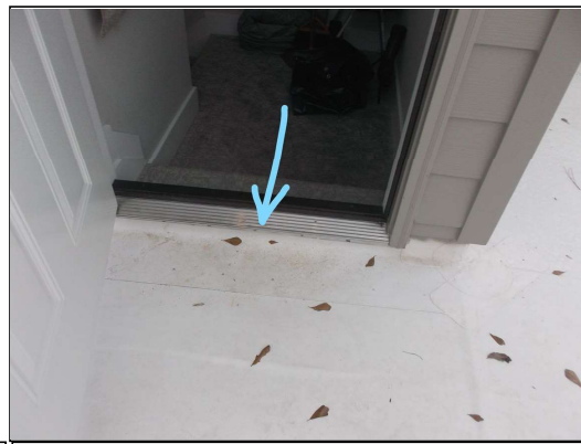
Roof door threshold not fully supported
