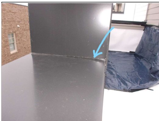
Poor caulk at parapet joints
