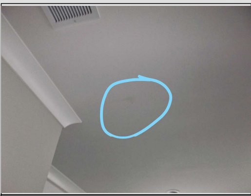
Dry water stain in master ceiling
