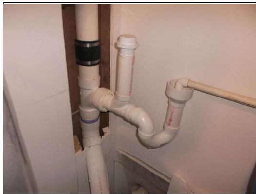
Hole water heater wall too wide @ waste pipe
