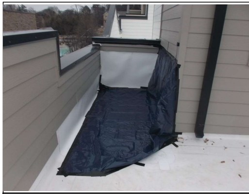
Water leak somewhere at west side of roof
