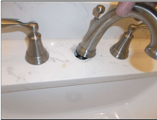
1st floor bath sink faucet detaching at base
