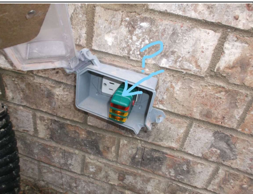
Front exterior outlet did not trip
