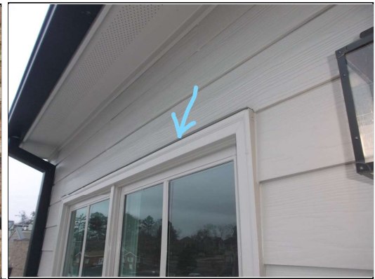
Gap at drip flashing over window, poor slope
