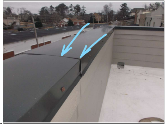
Poor sealing at parapet cap flashing
