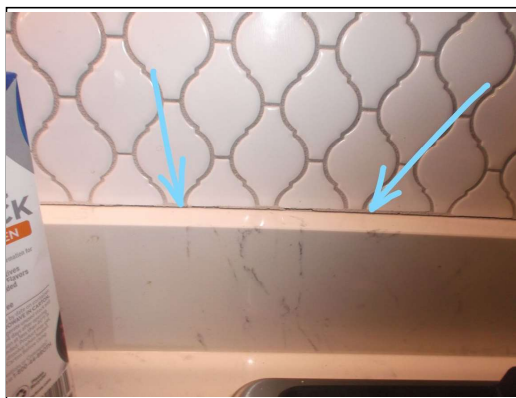
Cracks at grout at back splash and wall tiles
