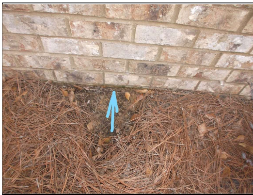
Soil contact brick and mortar at several areas
