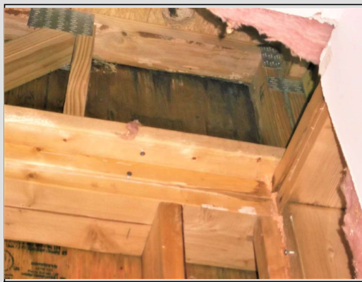
water intrusion at coat closet upper wall
