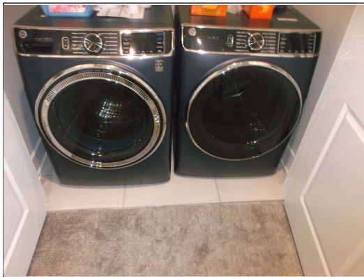
No washer drain pan in place
