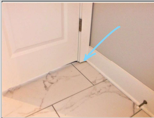
Missing caulk where door frames end at tiles
