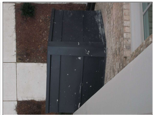
Workers debris on metal roofs
