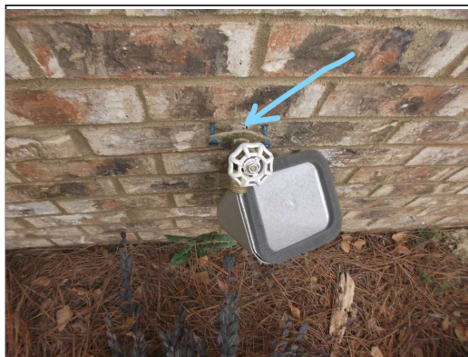
Hose faucet pipe exposed can freeze;
