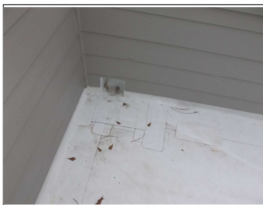
Numerous patches at scupper openings
