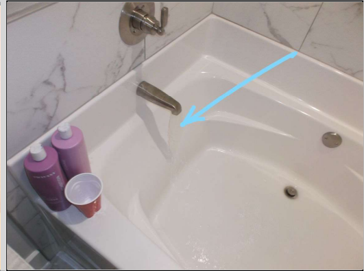
Poor water flow at master tub fspout
