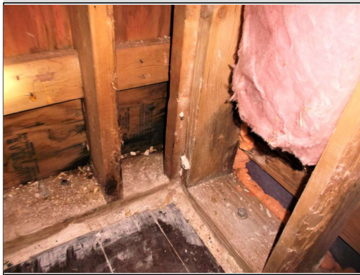
Water intrusion at lower coat closet walls
