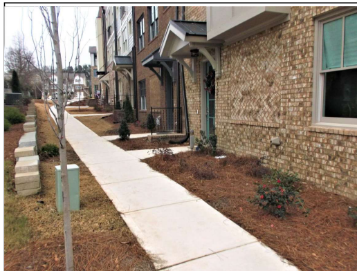
Walkway & soil grading has poor slope away
