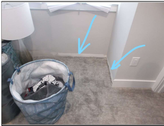
Missing baseboards in master bedroom
