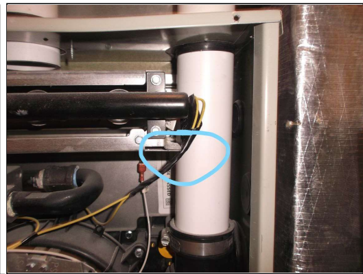
electrical wires contact burner flame shield
