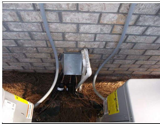
AC conduit not clamped to brick at lower area
