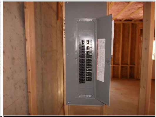
Screws too tight in distribution panel cover
