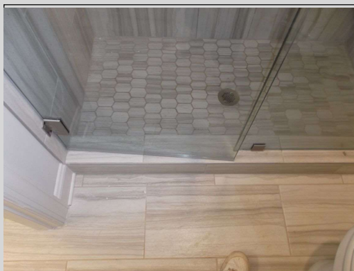
Shower door drags too much on curb
