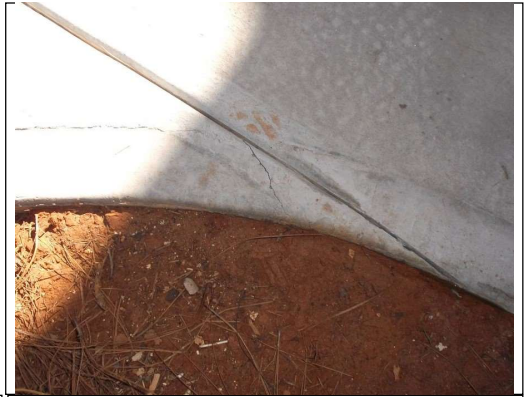
Crack in driveway corner right side of entry
