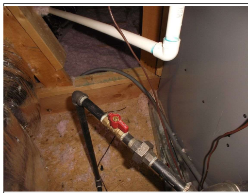
Conduit not clamped to wood in attic
