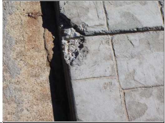
Broken section in driveway at the street
