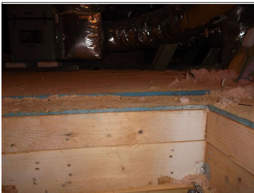
Attic floor layers are a trip hazard
