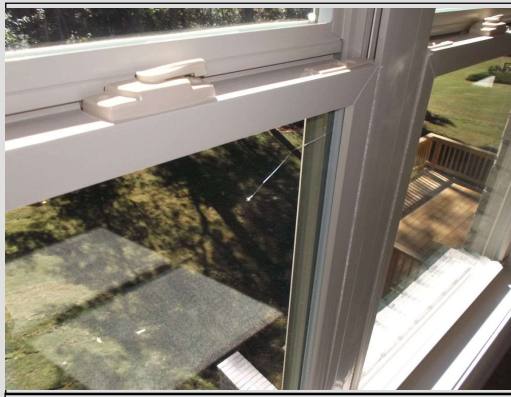
Cracked glass at master bed rear window
