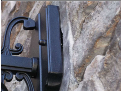
Missing caulk at light on stone wall
