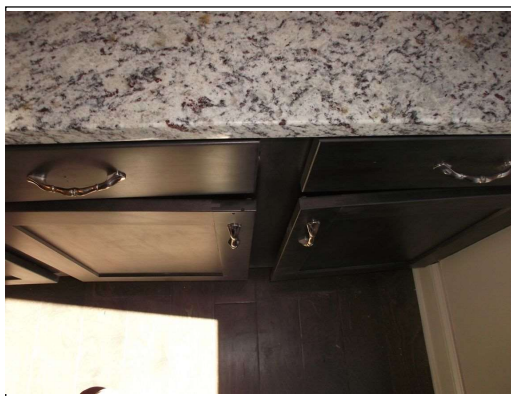
Doors not fully closing
