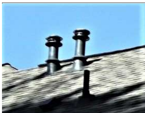
Flashing on top shingles face nailed
