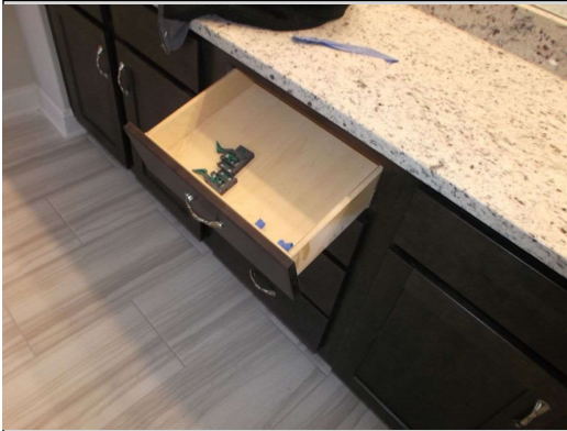
Defective drawer hardware at master
