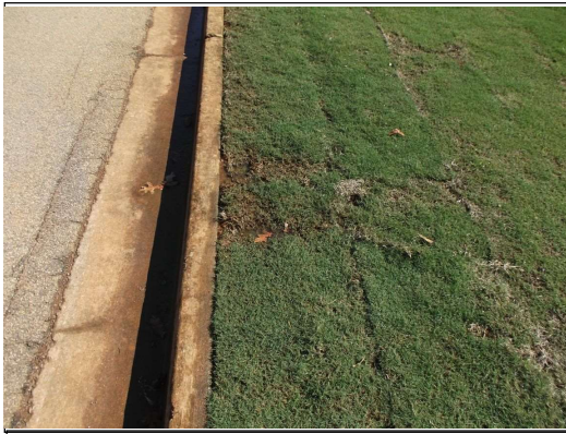
Excessive water in the ground at front yard
