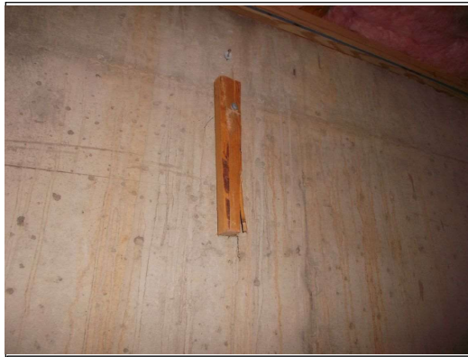
Wood nailed to foundation wall
