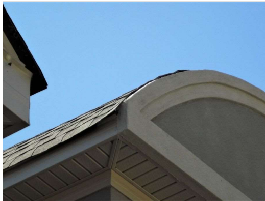
Shingles not covering top of stucco
