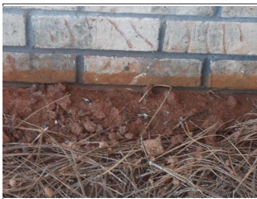
Soil contact mortar and brick
