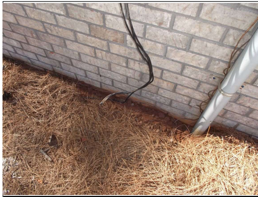
Cannot see the electrical system ground rod
