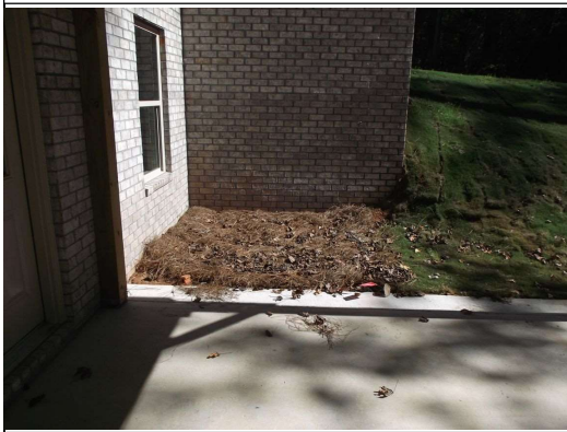
Poor soil slope out of inside corner
