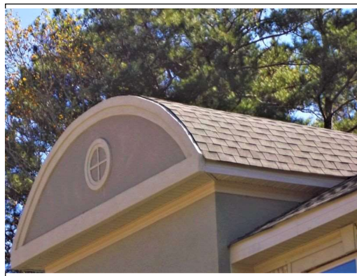
Shingles not covering stucco
