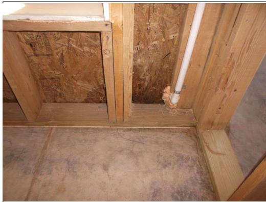
Water stains on exterior sheathing
