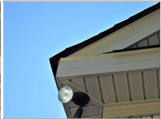
Metal fascia upper appears behind lower piece
