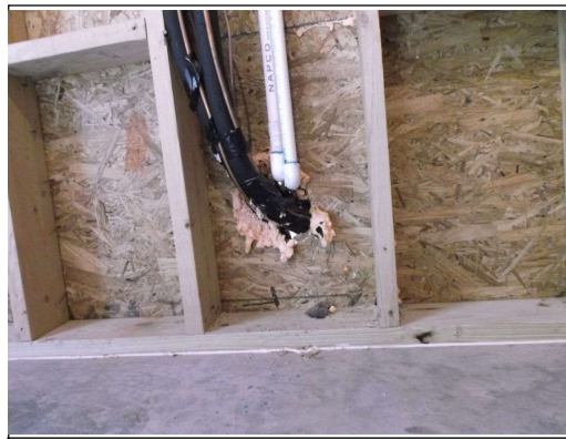
Hole in exterior wall
