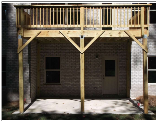
Deck and posts lean to the left
