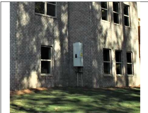
Water heater installed on the outside
