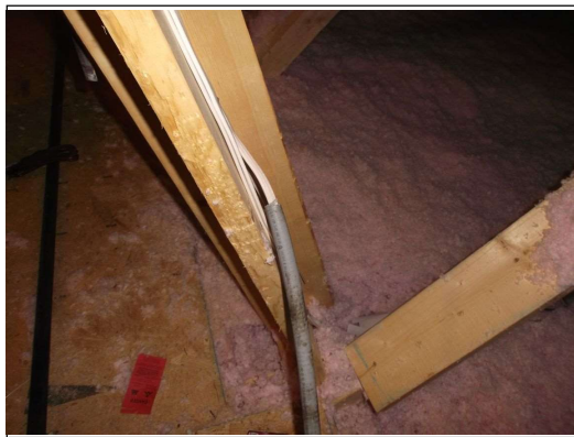
Electrical conduit not clamped to wood @ atti
