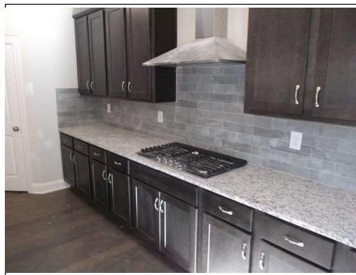
Workers residue on cabinets, appliances
