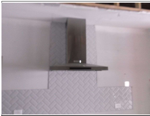
Verify no water got into exhaust fan controls
