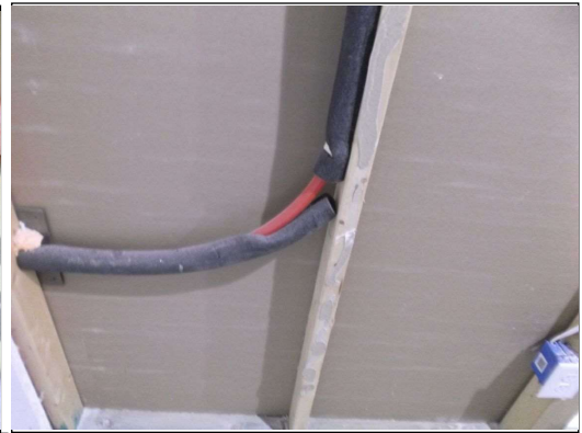
Detached pipe insulation
