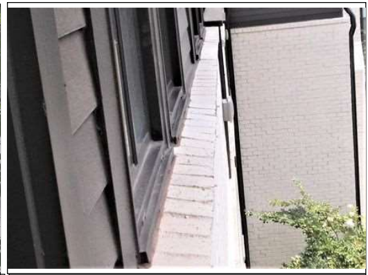
Gaps @ window seal caulk & openings @ ends
