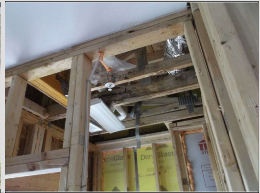
Dry water stains on ceiling framing
