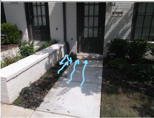
Walkway slopes to doorway/poor grading
