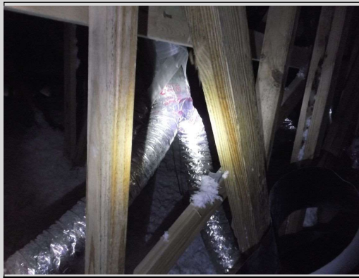
Two exhaust fan ducts join to one at attic
