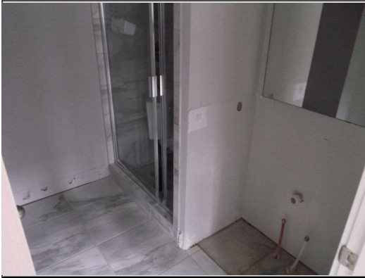
3/4 bath fixtures removed/waste pipe no cap
