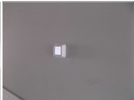
Verify thermostats have no water damage
