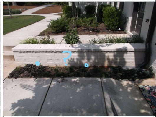
No drainage holes
