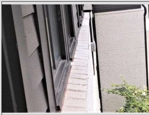
Gaps in caulk, cladding open at ends
