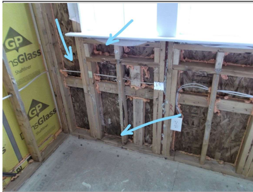
Dry water stains at exterior sheathing
