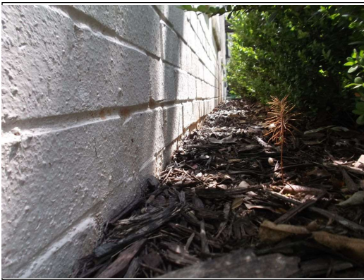
Cannot verify proper weep holes in veneer
