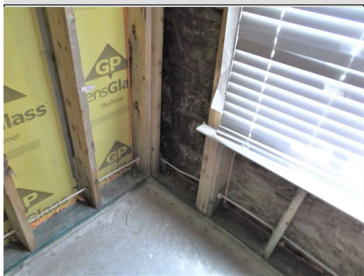
Dry water stains on sheathing
