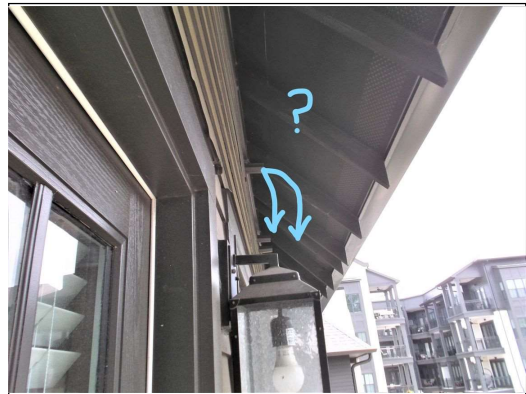
Pipes should have a elbow.
