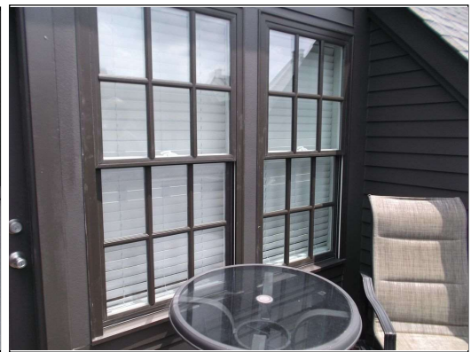
Defective paint on windows
