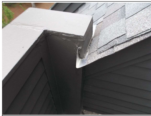
Sharp metal flashing at parapet wall and roof
