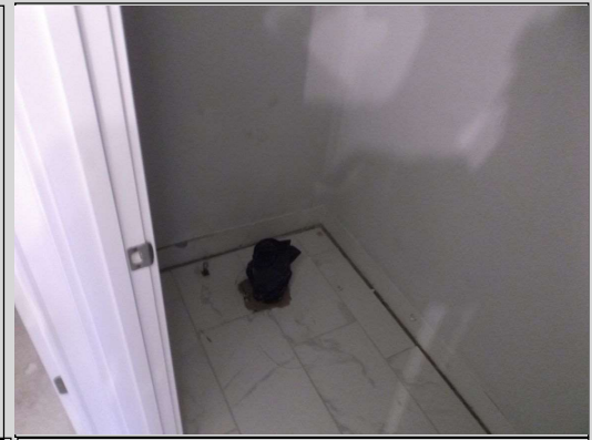
Toilet drain not properly capped
