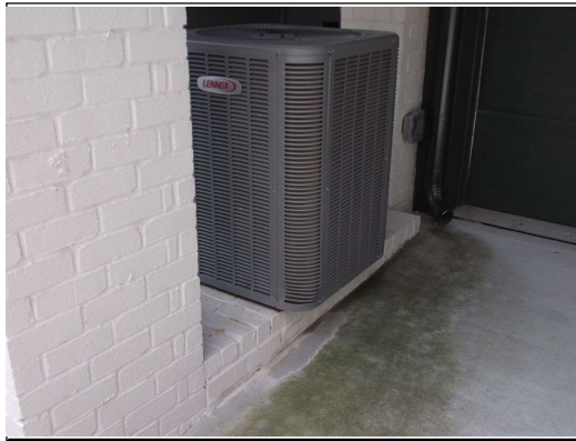
AC unit over property line/dent at bottom
