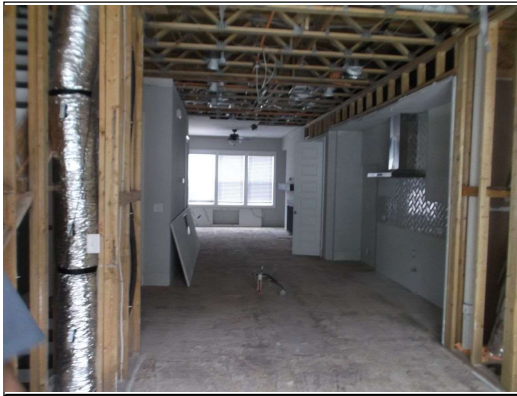
Sub floor damage
