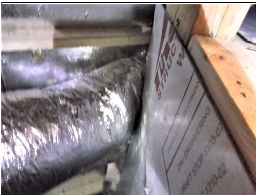
Air ducts appear crushed in attic ceiling
