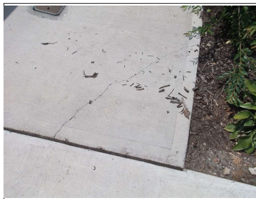
Driveway has broken corner at the street
