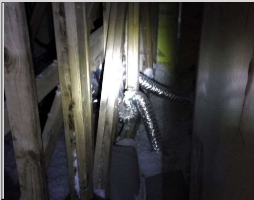
Exhaust fan duct has too many turns
