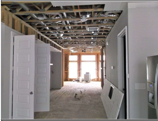
Verify no water intrusion to light fixtures
