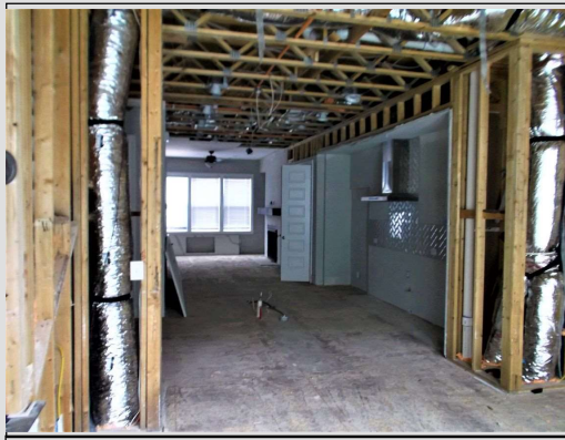
Sub floor damaged from flooring removal
