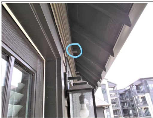
Drain pipe not turned down can drain back.
