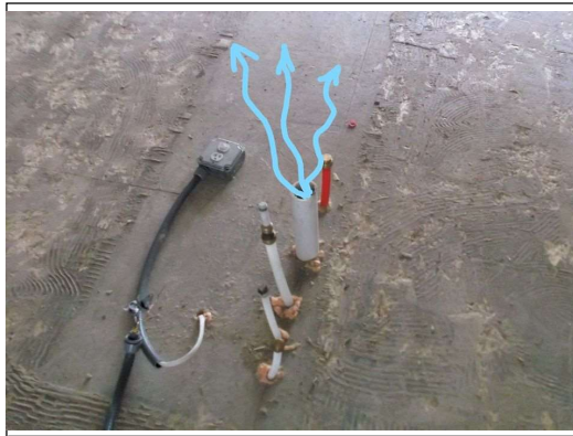
Open waste pipe in kitchen
