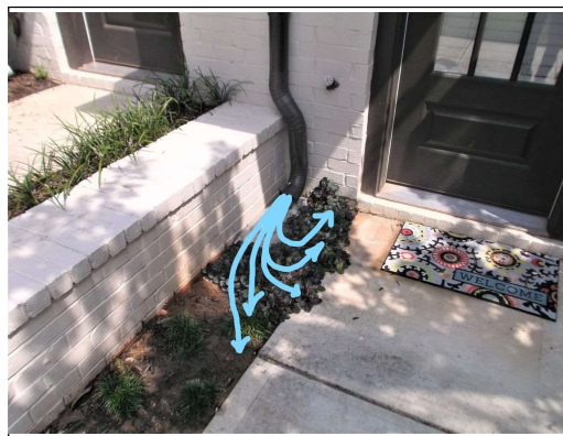
Soil has poor slope holds roof water
