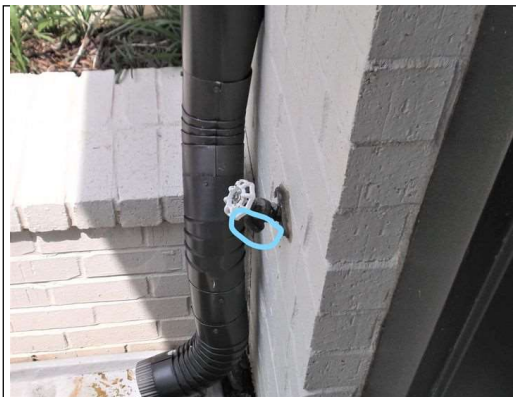
No anti siphon device on hose faucet
