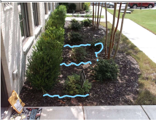
Poor soil grade and slope front plant bed
