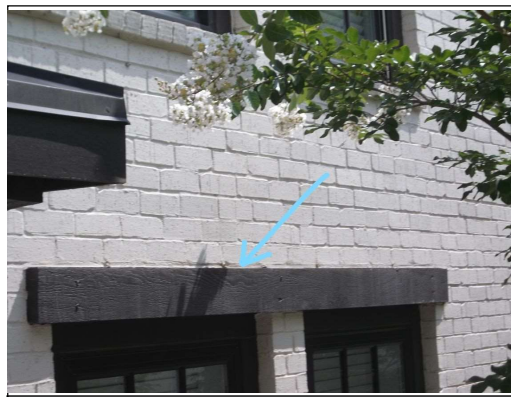
Cannot see flashing above beam
