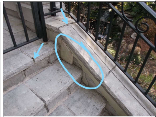
Movement cracks at basement stairs
