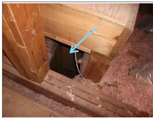
Missing insulation at keeping room wall (attic
