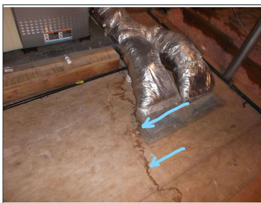
Dry water stains on attic floor at left furnace
