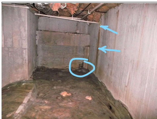
Water stains and dampness at wall
