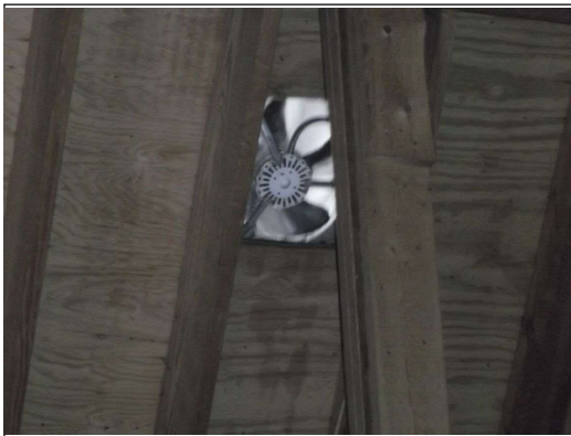
One exhaust fan in attic roof
