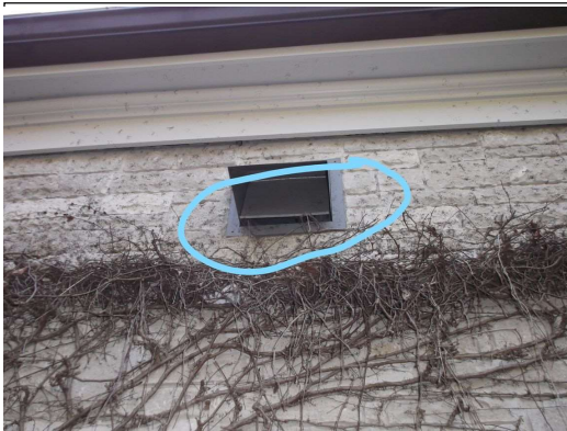
Kitchen exhaust fan terminal door open
