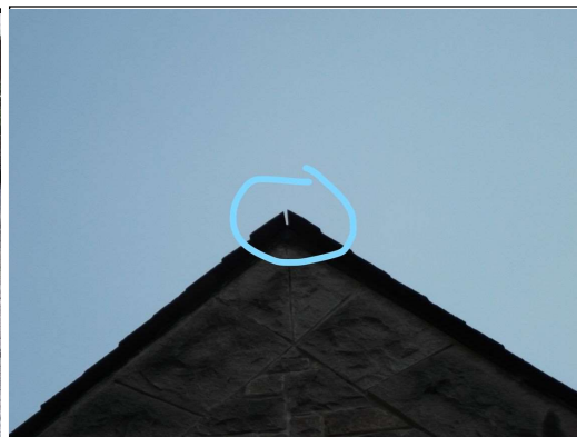
Split in slate shingle above garage gable
