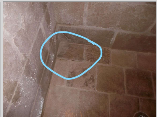
Loose tile in shower and defective grout
