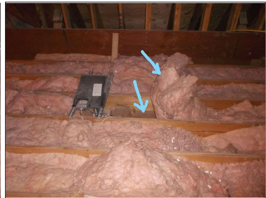
Ceiling insulation detached
