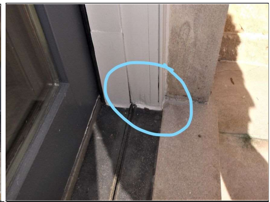
Water damage at rear door frames
