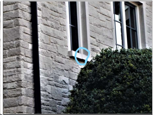
Settling crack at window masonry seal
