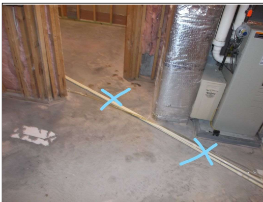
Drain pipes on floor can be damaged
