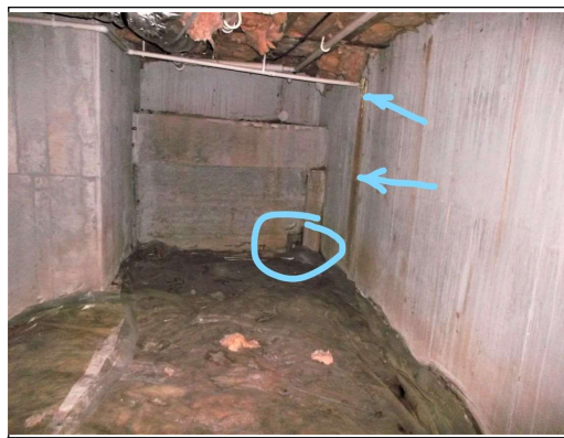
Damp foundation wall and water stains
