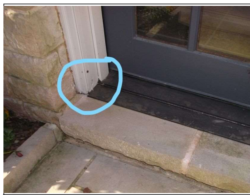
Water damage at rear door frames
