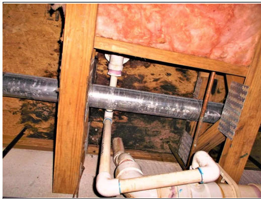
Water damage to floor seen in crawlspace
