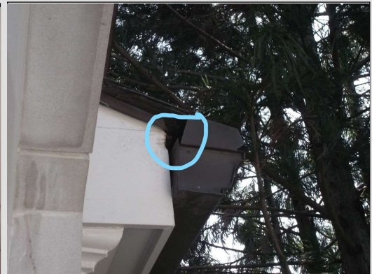
Hole in fascia seen from front bed window
