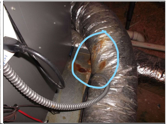
Rust stains in furnace pan at attic
