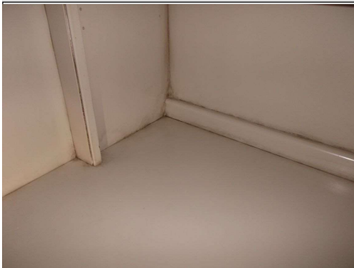
Verify stains are faux paint or not
