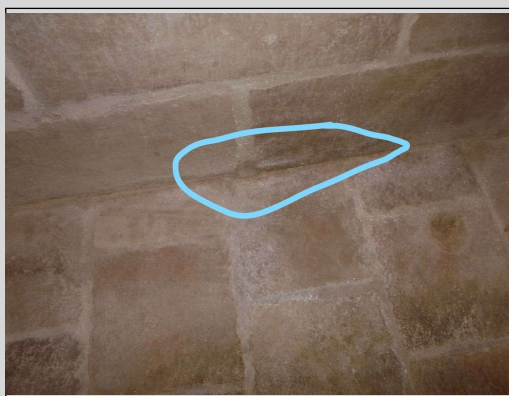
Cracks in shower tile grout
