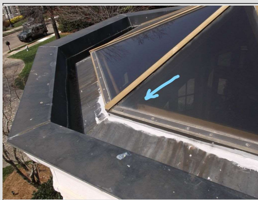
Cracked glass at skylight in sunroom
