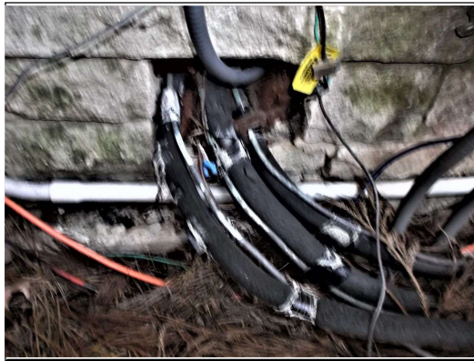
Missing, deteriorated refrigerant line insulatio
