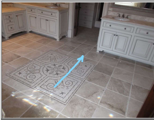
Floor slopes to sink wall
