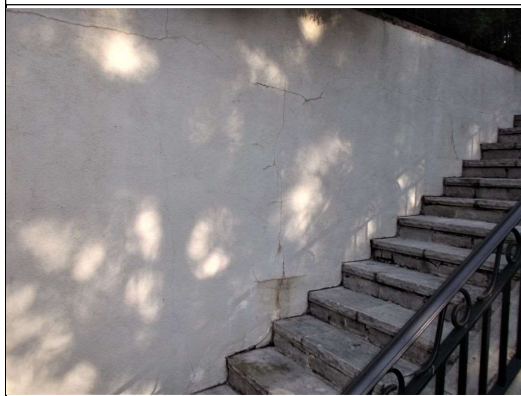
Movement crack and loose stucco
