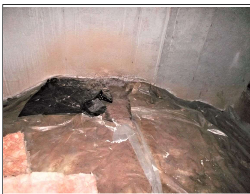
Exposed soil several areas
