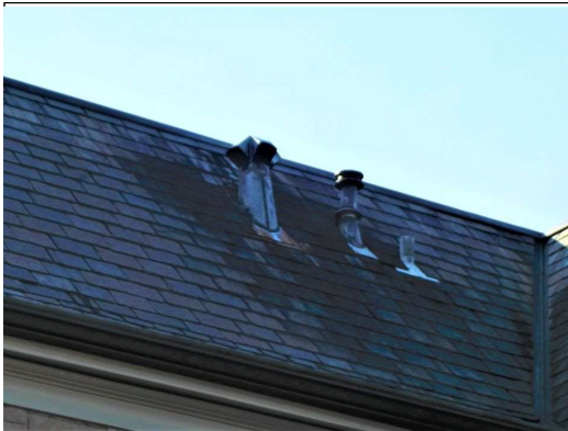
Shingles need wash, vent pipes need paint
