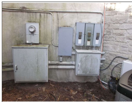
Outlet not energized below panel box
