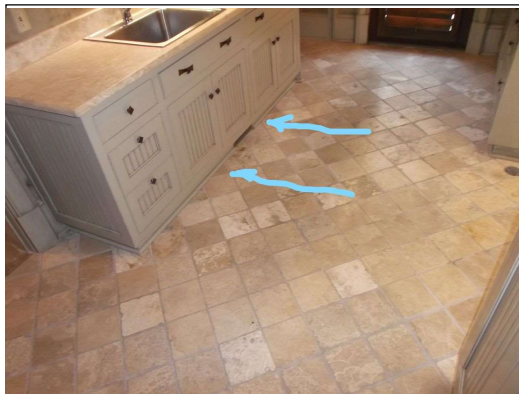
Laundry floor sinks at wash sink cabinet
