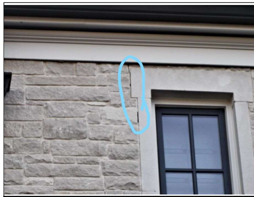
Settling crack at front left window
