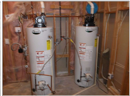
Copper & steel pipe join above water heaters
