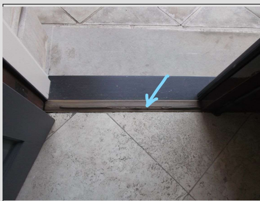
Front door weather strip damaged
