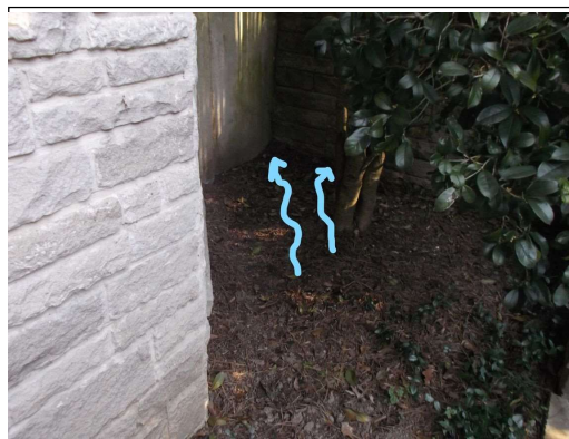
Soil slopes to foundation right side of house
