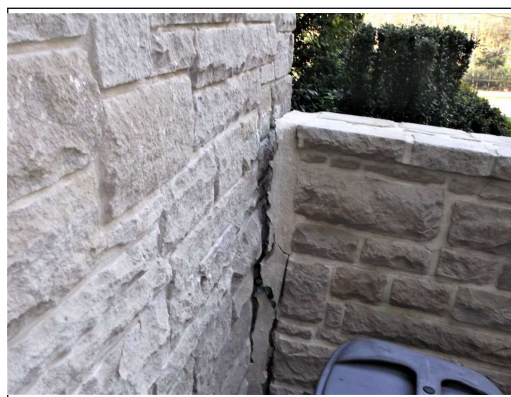
Wall detaching at side of house
