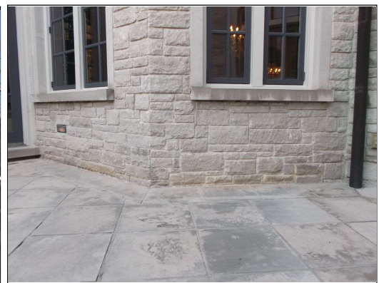
Missing weep holes in veneer several areas
