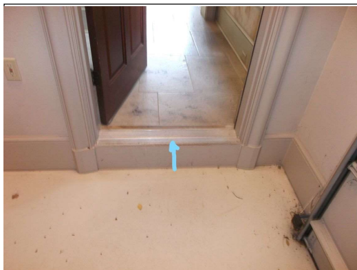
Step up from garage is a trip hazard (high)
