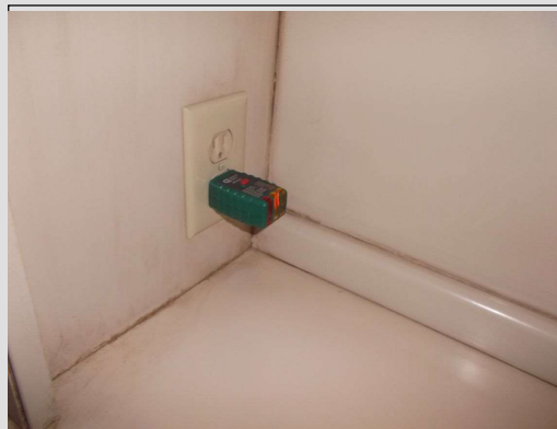
Outlets tested open ground at wall cabinets
