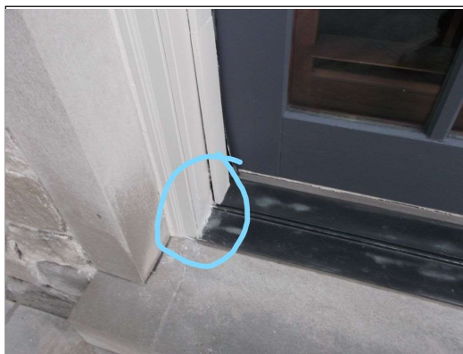
Water damage painted at front doors
