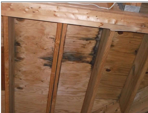
Dry water stains seen from the stairwell
