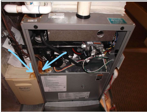
Rust in furnace at basement
