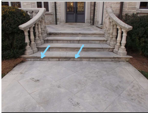
Settling crack across the bottom step joint
