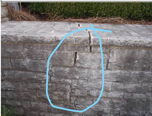
Movement cracks at the front yard wall
