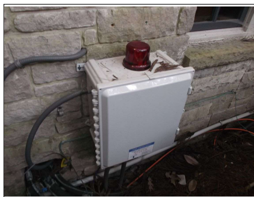
Ejection/septic controls at basement ground?
