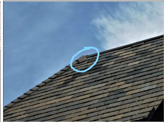
Detaching or loose shingle at front ridge
