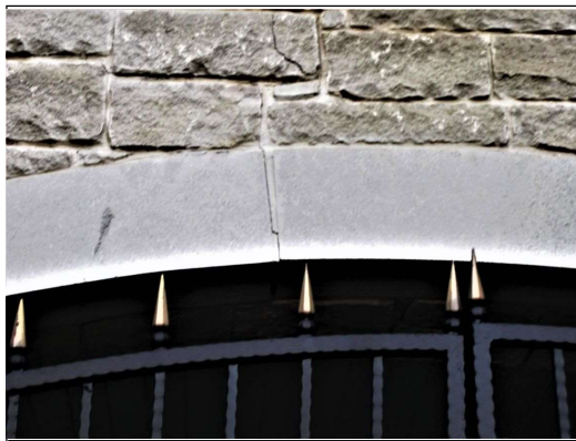
Settling crack at masonry header
