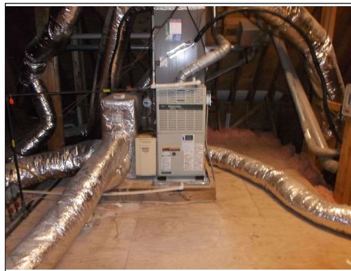
One older furnace in attic
