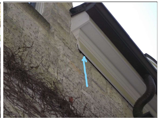
Freeze board gap at brick needs filler
