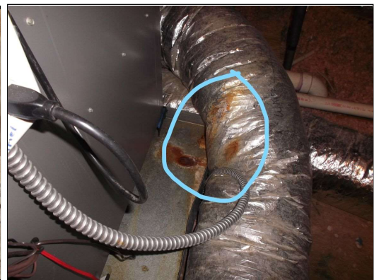
Dry water stains right side of furnace
