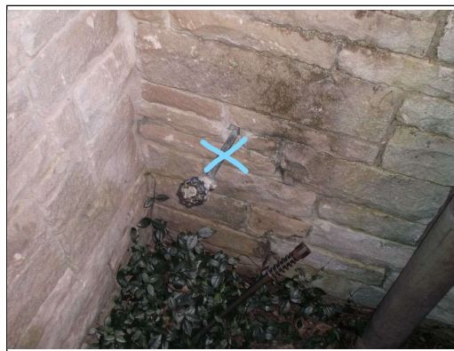
Hose faucet pipe too far out wall
