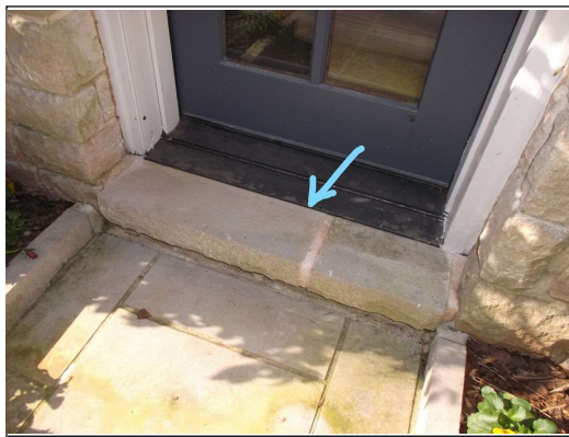
Missing caulk at threshold on masonry
