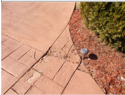
Cracks and damage at the driveway
