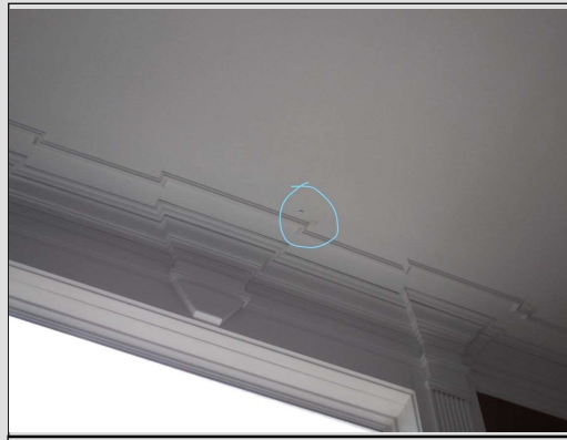
Nail pops in ceilings
