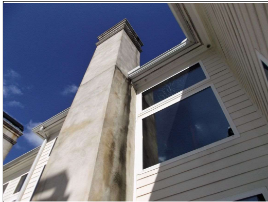
Missing flashing where roofs meet chimneys
