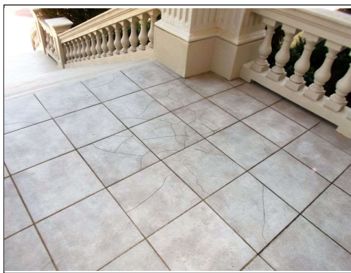
Cracks in the front portico floor tiles
