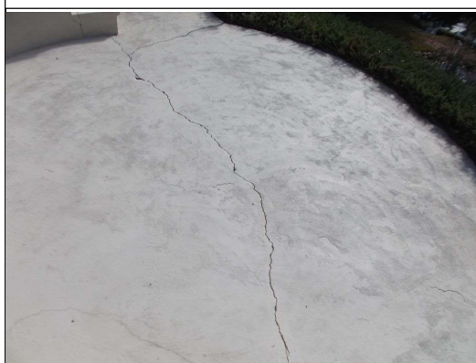
Crack in walkway
