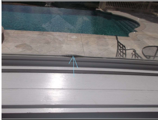
Glass sill defective
