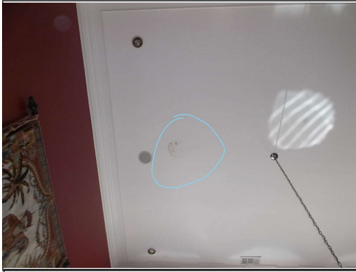
Dry water stains in ceilings
