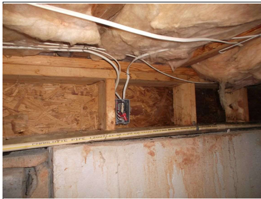
Open junction box in crawlspace
