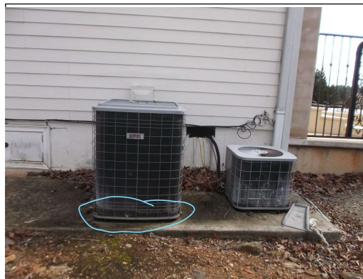
Debris and corrosion at the bottoms of ACs
