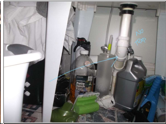
Sink waste pipe has no J-Trap
