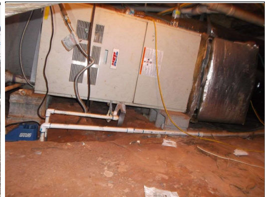
Furnace in the crawlspace defective
