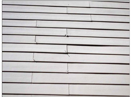
Siding damaged and nails extracting at areas
