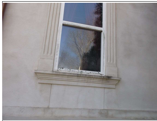
Some window sash are rotting
