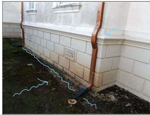
Poor soil slope and erosion at areas
