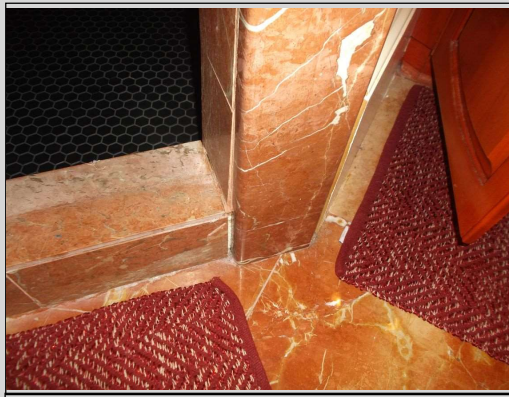
defective grout at master shower curb
