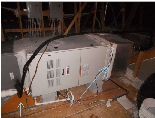
Rust in attic furnace drain pan
