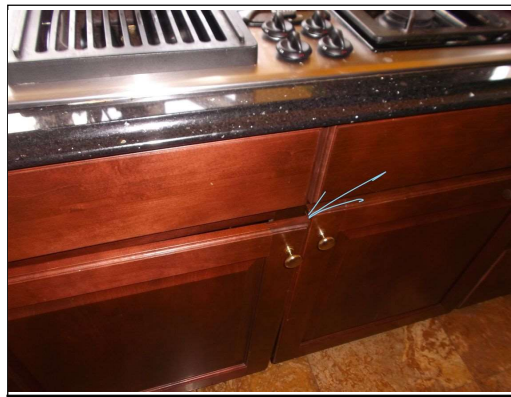
Base cabinet door bowed at cook top
