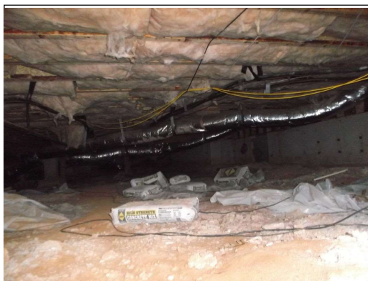
Concrete debris throughout crawlspace
