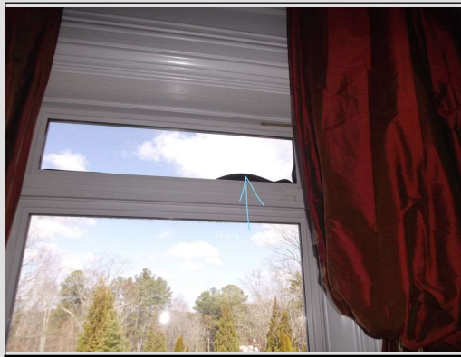
Window seals spill into glasses at areas
