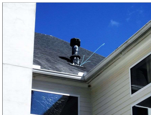
Vent pipe flashing on top shingles face nailed
