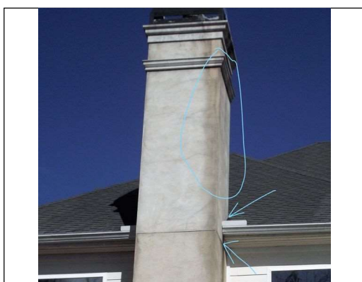
Defective flashing at chimney
