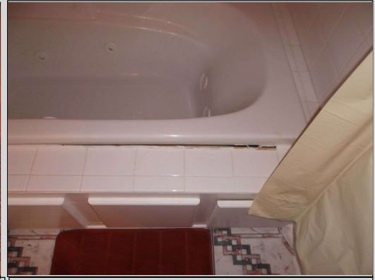
Tub movement at deck tile indicate settling
