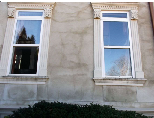
Stucco cracks may indicate water intrusion
