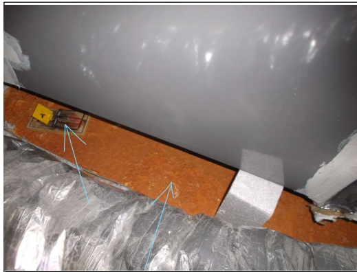
Rust and water in one attic furnace drain pan
