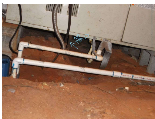
No sediment trap in gas pipe to furnace
