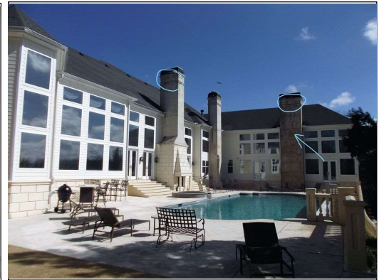
Water intrusion at chimneys
