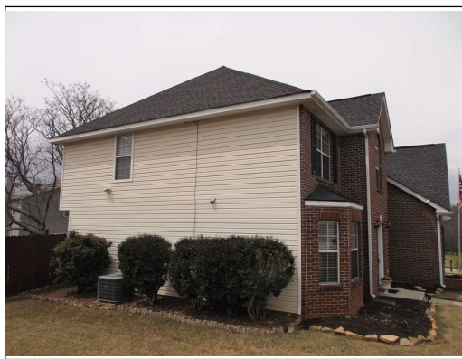
Missing gutter at right side of house
