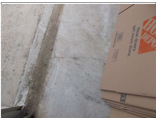
Crack in floor near door
