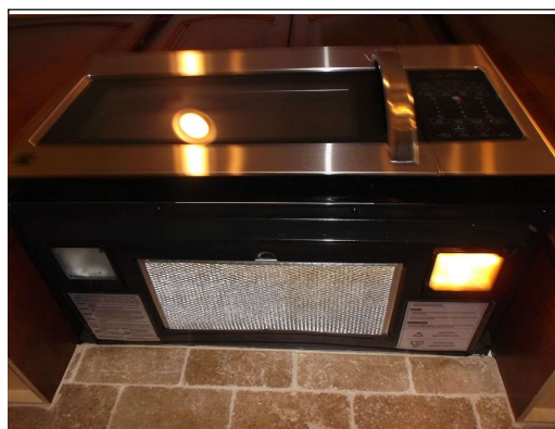
Left light out at exhaust hood
