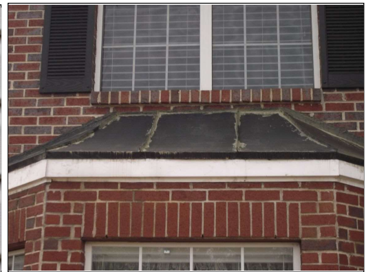
Wood fascia needs painting
