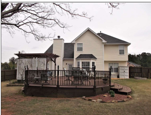
Wood deck railing loose/posts in soil
