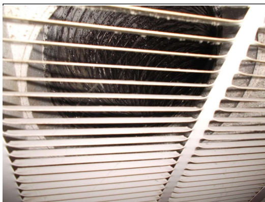
Dust inside air duct returns
