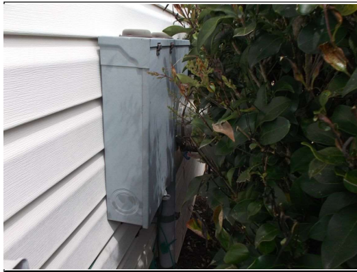
Bushes block access to meter and panel box
