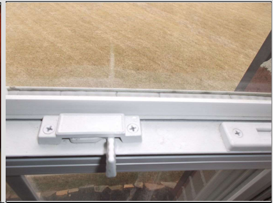
Seals between glass are cracking
