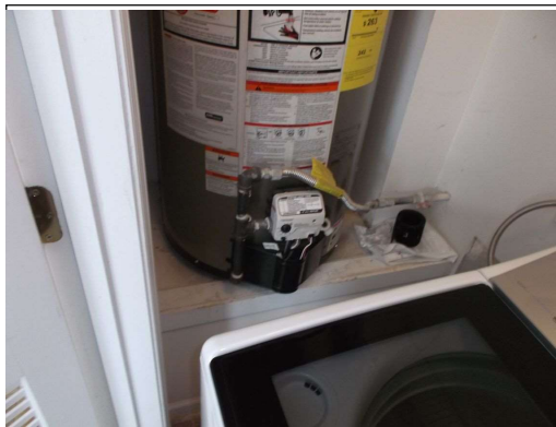
Water heater not in a drain pan
