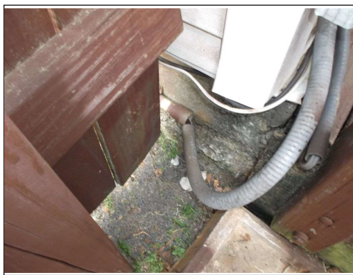
Detached conduit @ right rear corner of house
