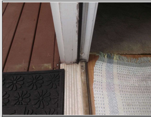
Water damage at rear door frame
