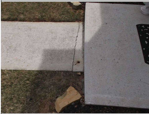
Porch settling and cracks in walkway
