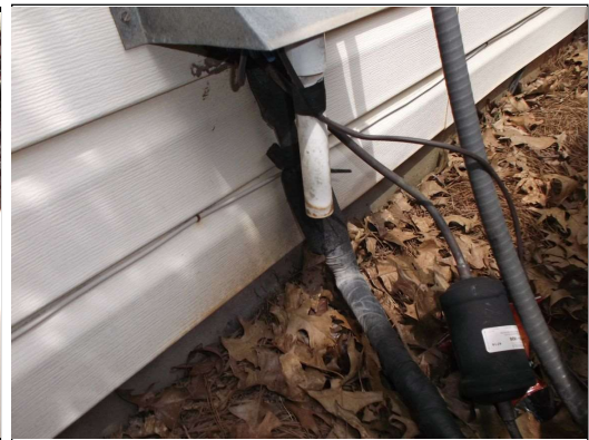
Condensate pipe drains at foundation
