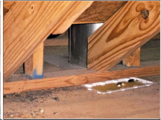
Chimney pipe too close to wood in attic;
