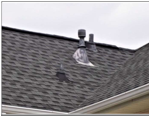
Pipe/vent flashing face nailed on top shingles
