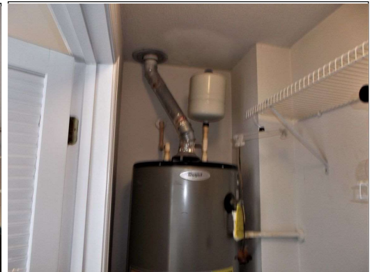
Expansion tank not braced from the wall
