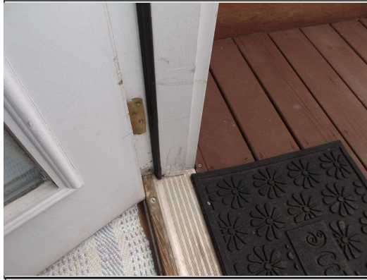
Rear door frame has water damage
