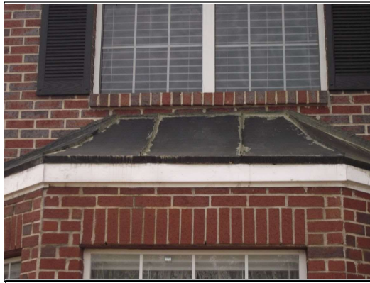
Caulk or sealant spilled on metal roof
