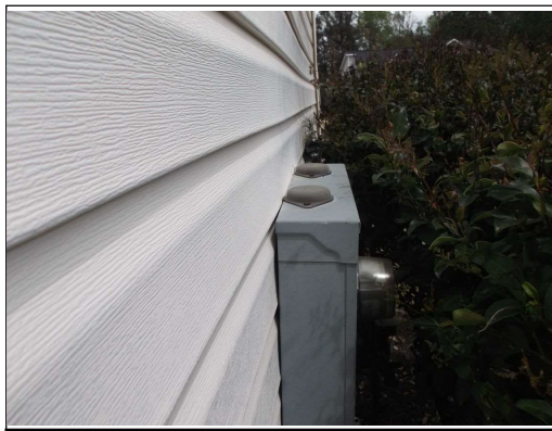
Missing bead of caulk over top of meter box
