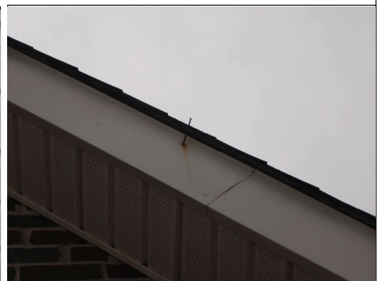
Nails rusting in front fascia
