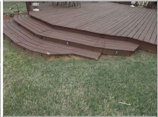
Deck wood resting in soil/dips & sags in floor
