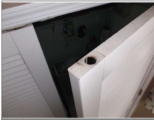
Missing snap hardware at top of laundry door
