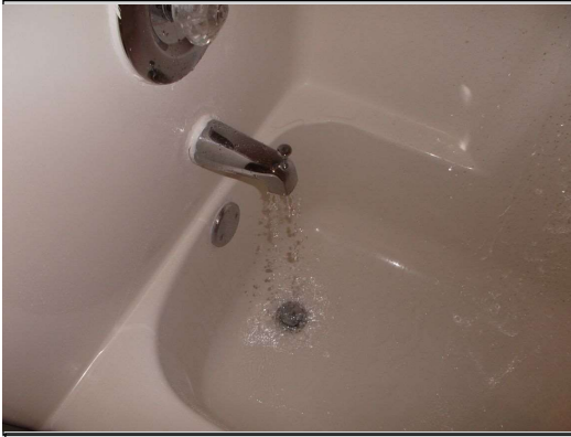
Water bypass when shower water flowing
