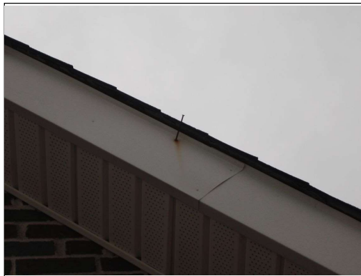
Nails rusting in metal fascia at the front
