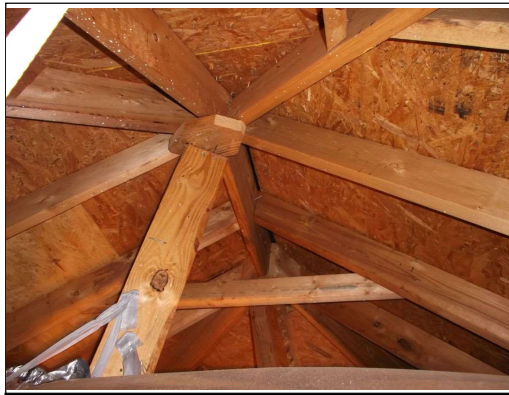
Plywood not cut wide enough for ridge vent
