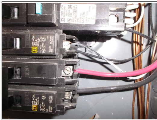
2 hot wires connected to one breaker
