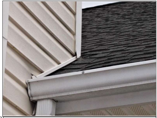
Cannot see roof to chimney flashing
