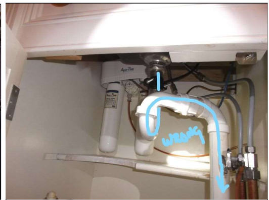
Sink drain pipe is a S-Trap
