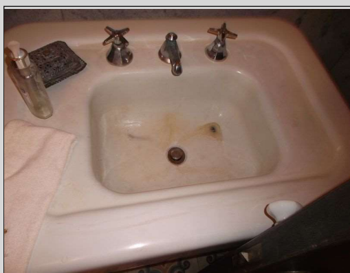
Sink bowl has rust in finish
