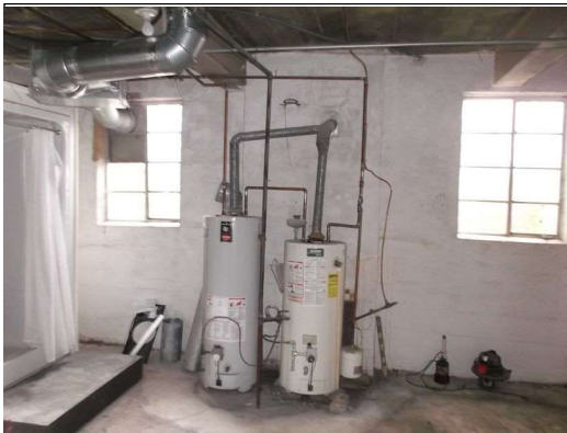
Water heaters at end of use
