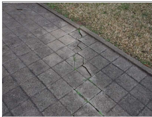
Moderate cracks in front walkway
