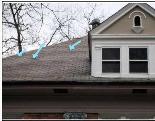
Broken slate shingles
