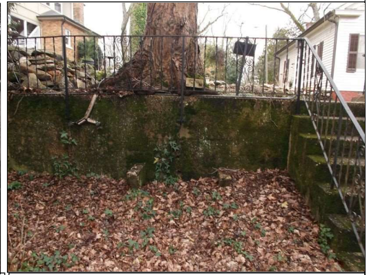
Rear yard retaining wall leaning and no holes
