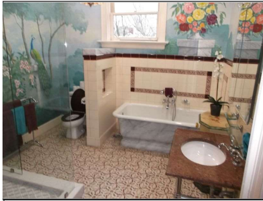
Tub faucet defective
