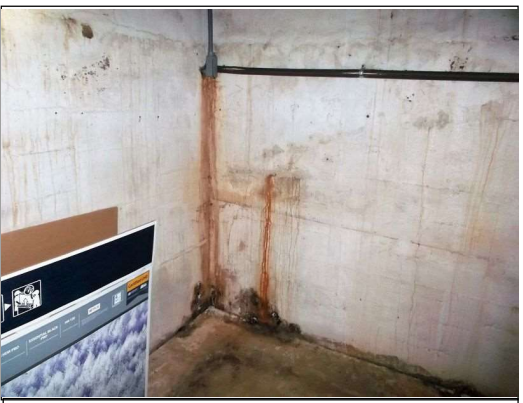
Water intrusion at front basement wall
