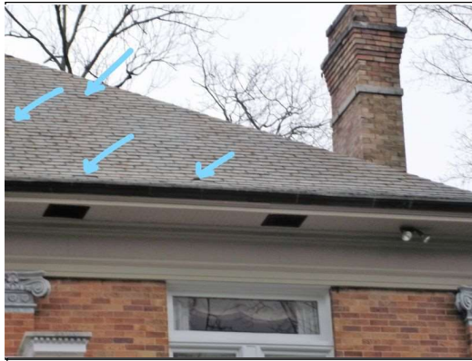
Broken and missing slate shingles
