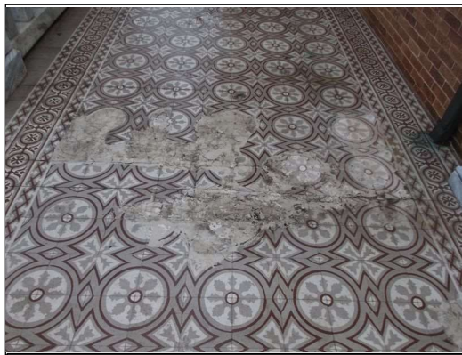
Front porch floor has water damage to tiles
