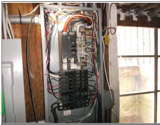
Sharp screws in panel box
