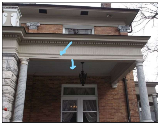
Water damage and sagging beam front porch
