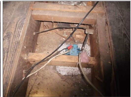
Exposed wire connections in attic floor
