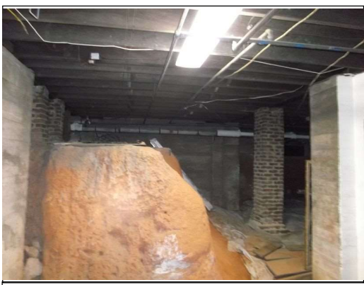
Exposed soil in crawlspace
