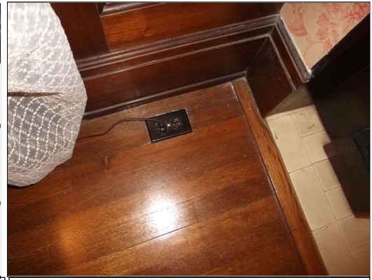
Improper receptacles in floors
