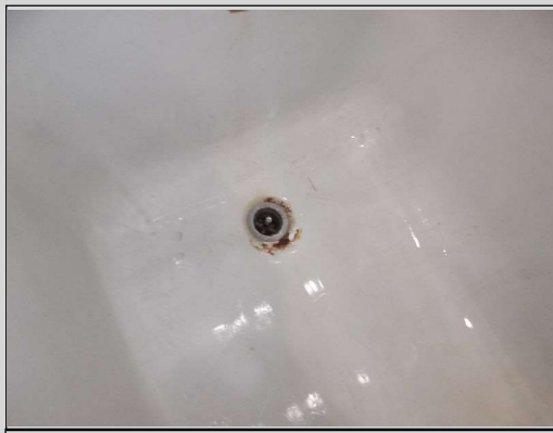
Rust in tub finish and stopper missing
