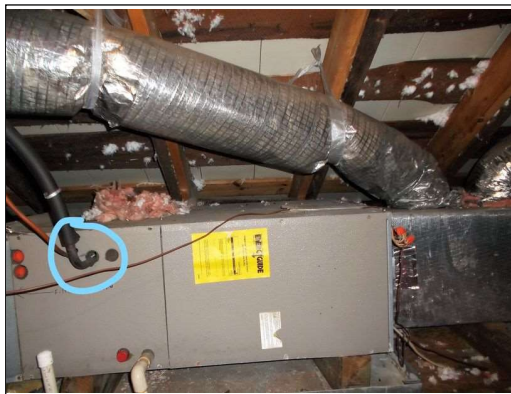
Missing refrigerant line insulation at out house
