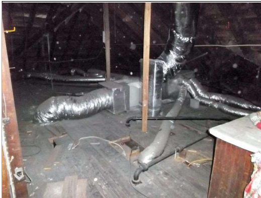
2nd attic furnace needs repair
