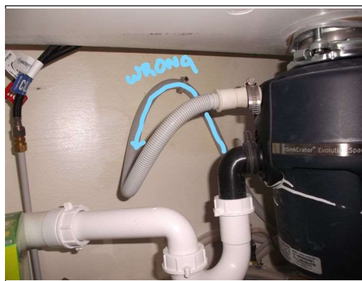
Dishwasher drain pipe not high looped
