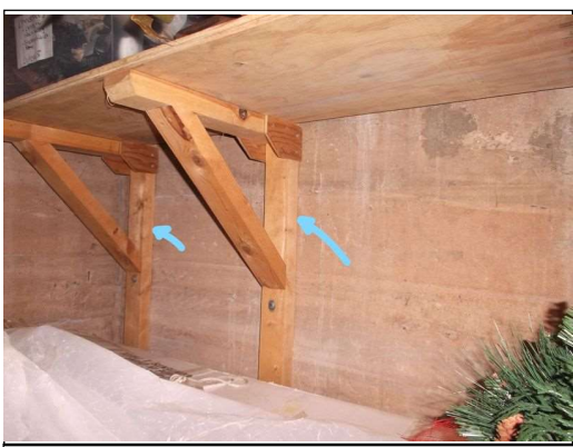
None treated wood attached to masonry
