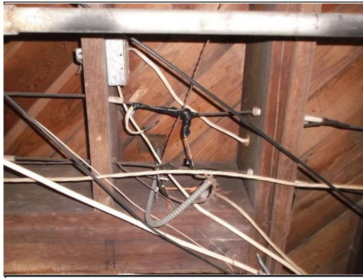
Exposed wire connections @ basement ceiling
