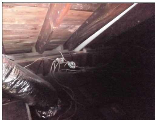
Exposed wire connections
