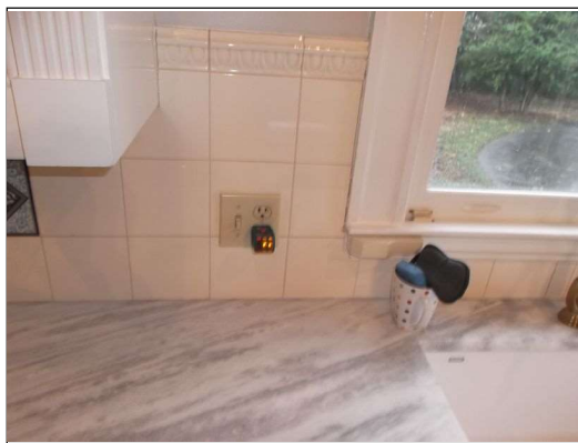
Kitchen outlets not GFCI protected
