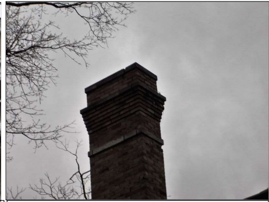
Defective &amp; deteriorated mortar @ Chimney
