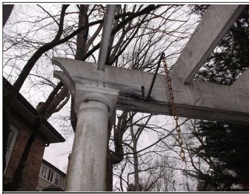
Water damage to rear courtyard trellis wood
