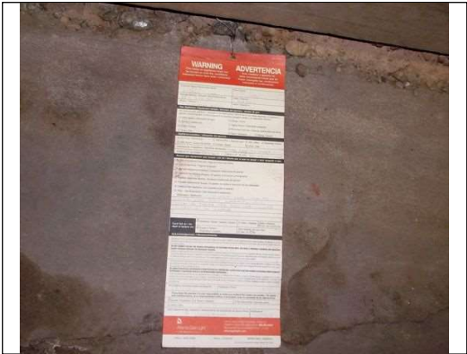
Furnace has been red tagged in basement
