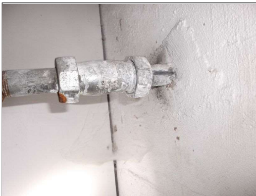
Main water pipe galvanized steel end of use
