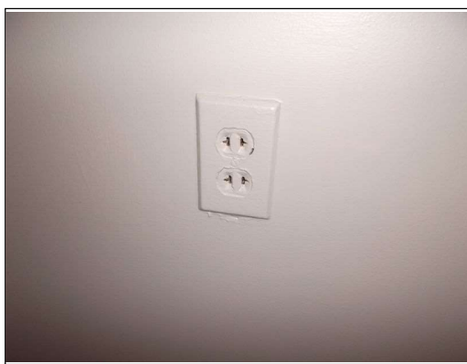
Outlets have no ground several areas
