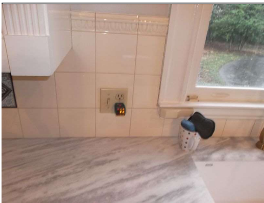
Outlet not GFCI protected
