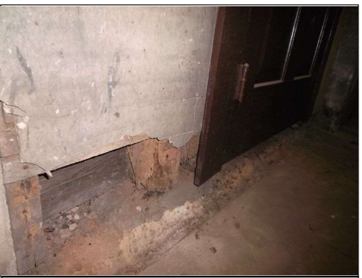
Basement wall framing dry rot several areas
