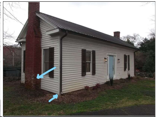
Damaged chimney brick @ guest house
