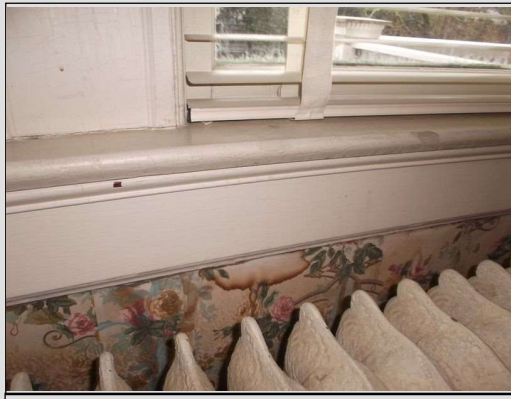
Water stains below windows
