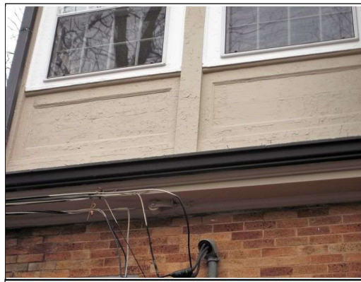
Defective paint at wood at box windows
