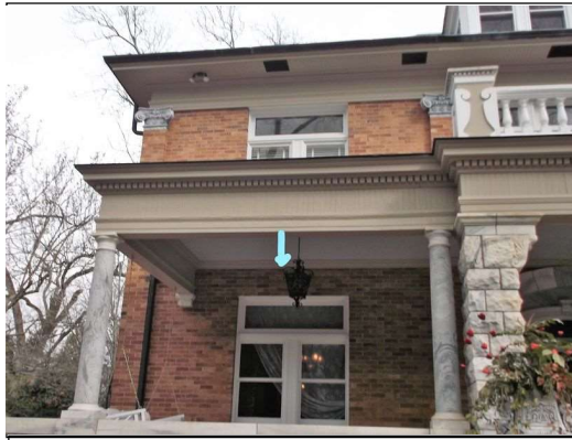
Front left porch beam sagging
