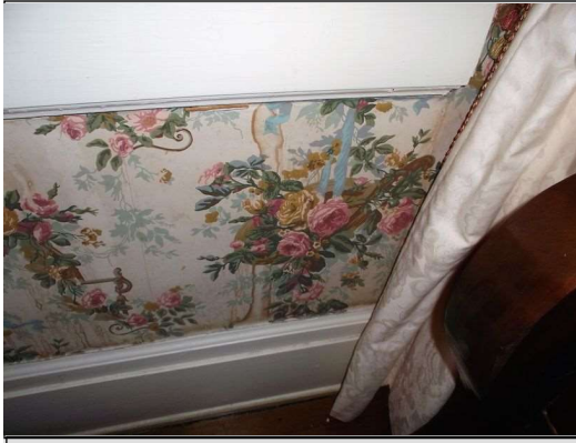
water stains in wal paper
