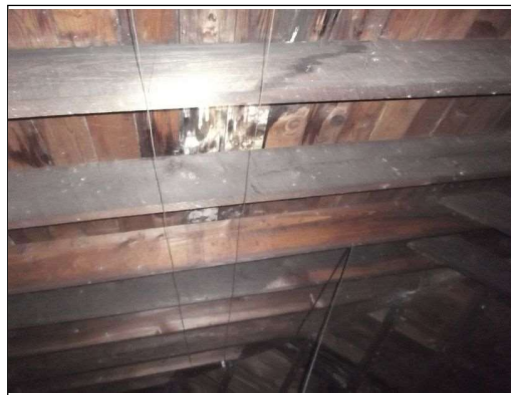
Mold, rot under roof decking
