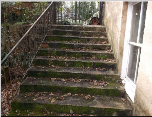
Rear stairs to basement cracking and broken
