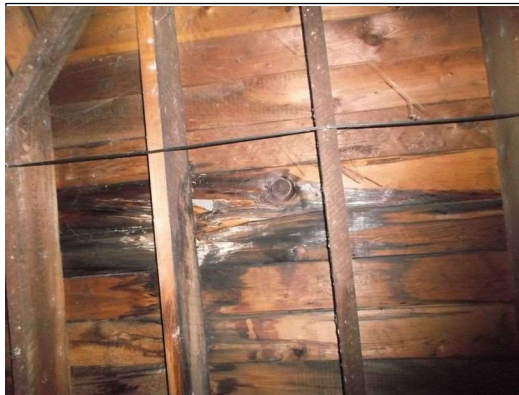
Mold and fungus under roof decking
