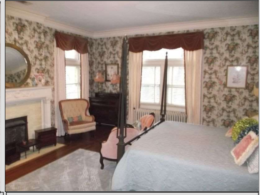
2nd bedroom floor slopes to exterior wall
