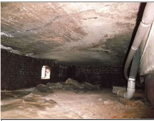
Exposed soil in crawlspace under porch
