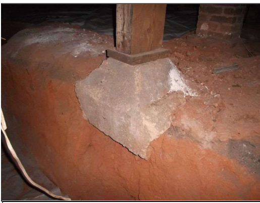
Foundation poorly rests on dirt
