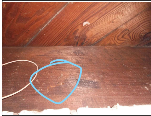
Termite trails in some floor joists
