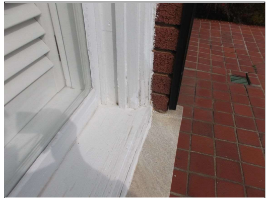
water damage to front window frames
