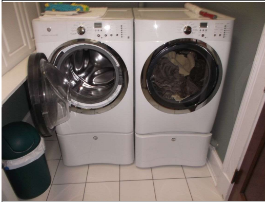
No washer drain pan installed
