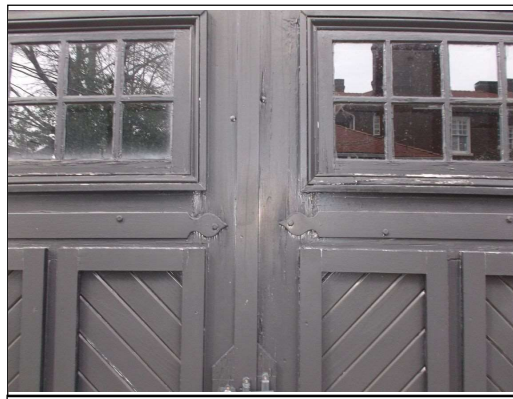
Garage doors have water damage
