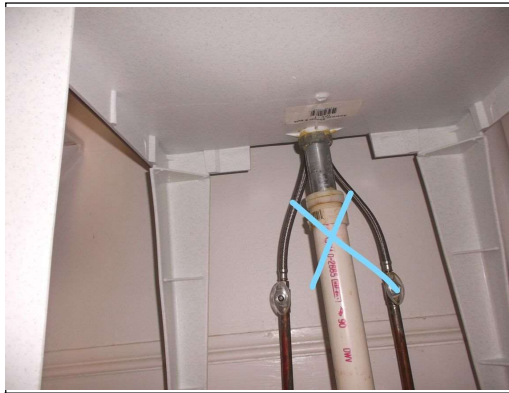
Washing sink drain pipe improper/unsafe
