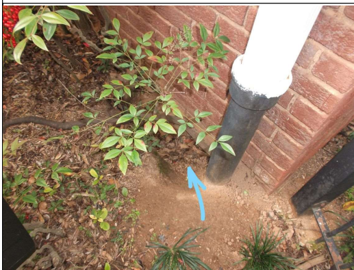
Hole in the soil at the foundation left side
