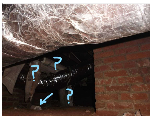
Damaged and loose Asbestos materials
