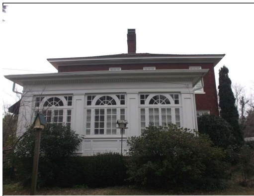
Defective paint at sun porch trim
