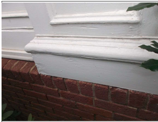
Water damage to wood trim
