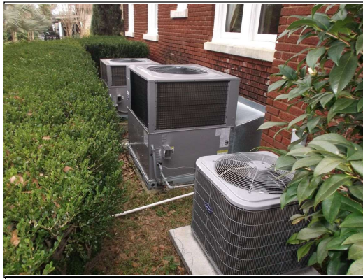
Bushes too close to HVAC units
