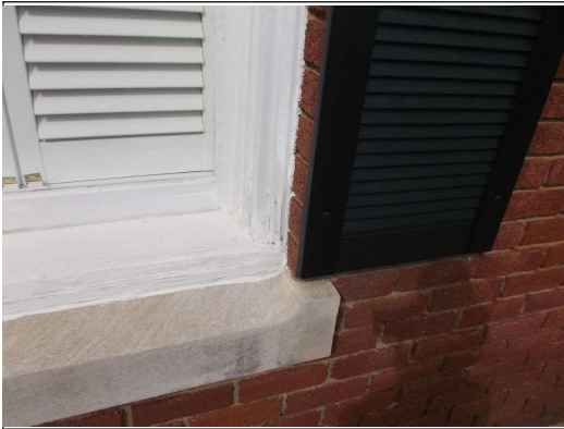
Window trim has water damage
