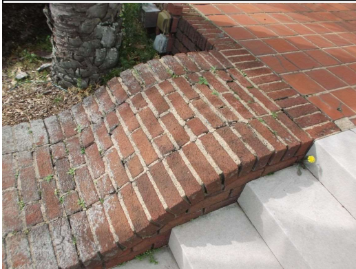
Deteriorated mortar at front porch step walls
