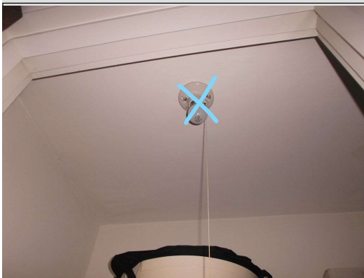
Exposed light bulbs in closets
