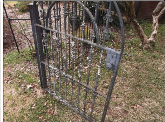
Wrought iron fence & gates need wash, paint
