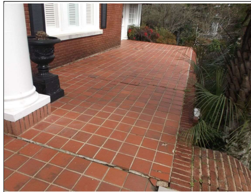
Front porch floor has settling cracks
