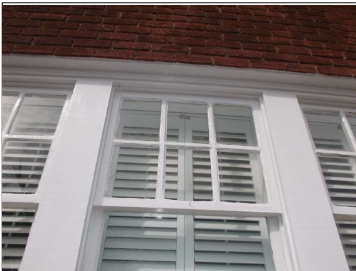
Window glass putty defective several area
