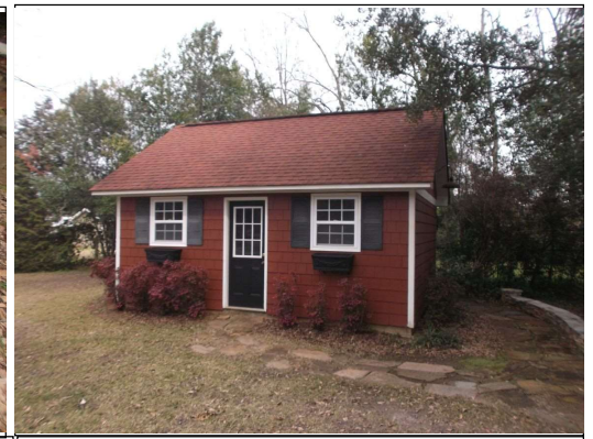
No gutters at storage house
