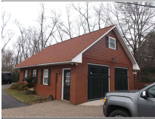
No gutters at main garage
