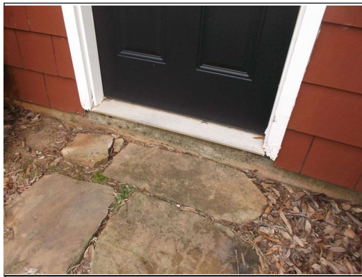
Water damage to storage house door frame
