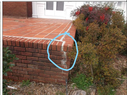
Front porch floor brick has movement cracks
