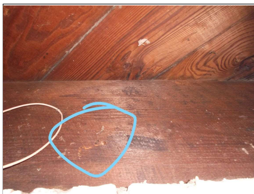
Termite trails in some floor joists & rim joists
