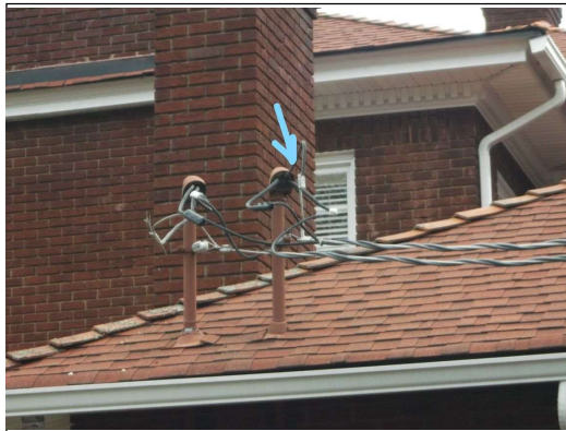
Improper drip loop in service cables
