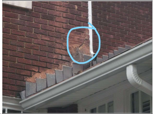
Settling crack in brick above sun porch roof
