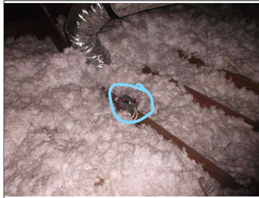
Open junction boxes &amp; exposed connections
