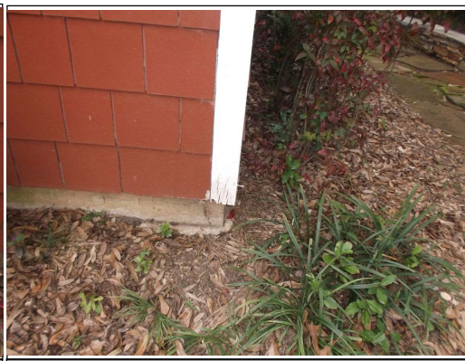
Water damage at storage house trim
