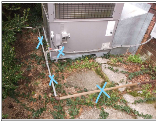
Water pipe for gas pipe 2nd HVAC heat unit
