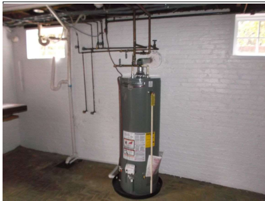
No expansion tank above water heater
