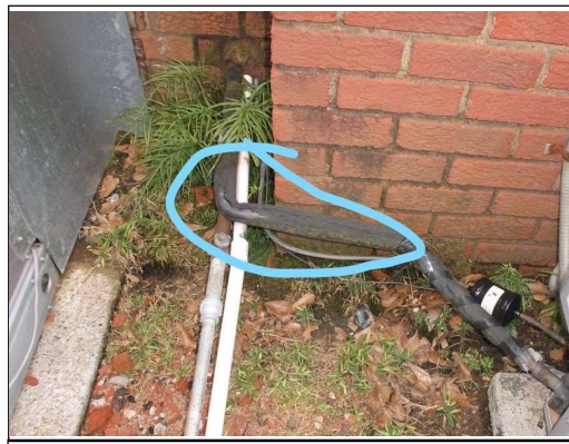
Refrigerant line insulation deteriorated
