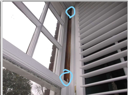
Sash cords and springs broken at windows
