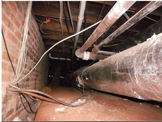
Missing moisture or vapor barrier
