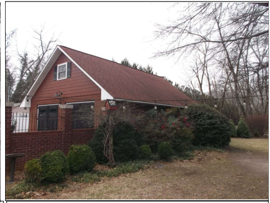
Bushes touching side of building
