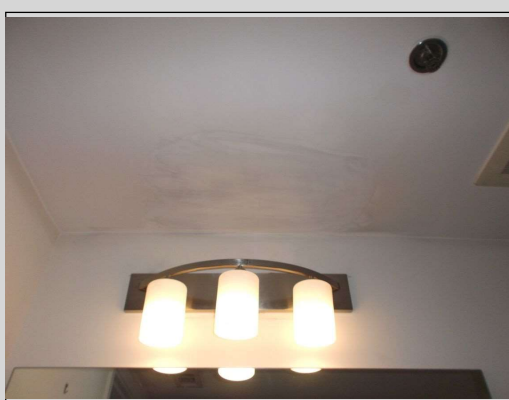
Dry stains in ceiling
