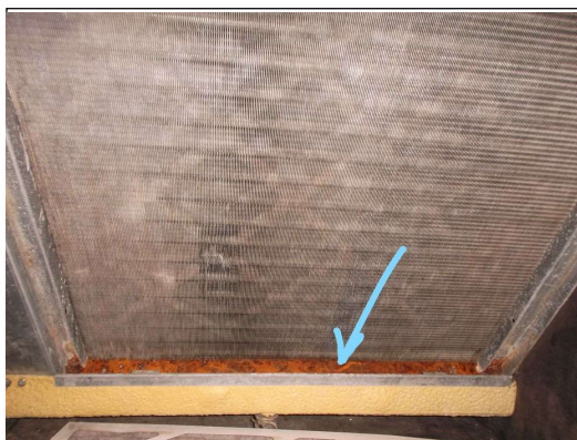
Rust in condensate tray
