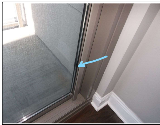
Seal bleeds into sliding door glass
