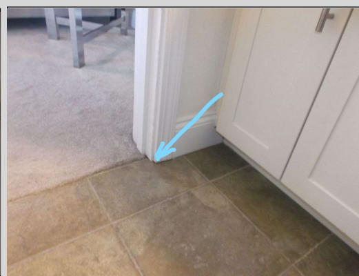
Missing caulk at gap below door trim and tile
