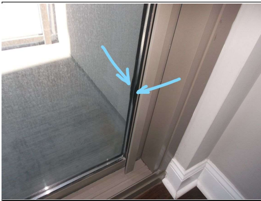
Seal bleeding into sliding door glass
