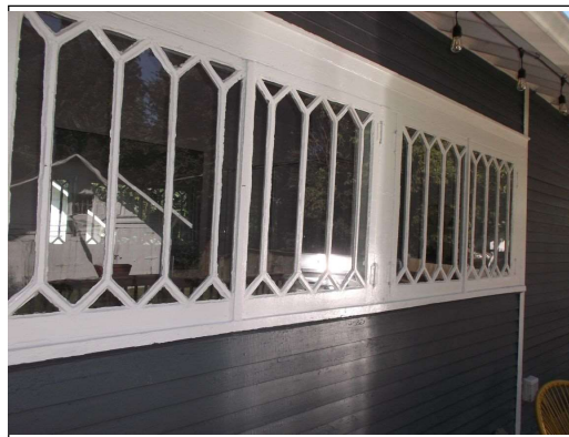
Several windows painted shut
