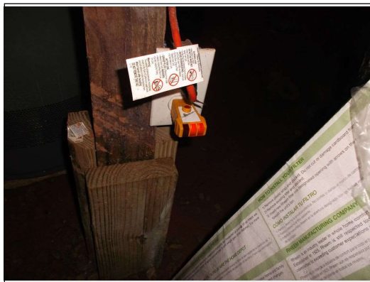
Outlet not GFCI protected
