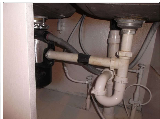
Tape wrapped around sink pipe
