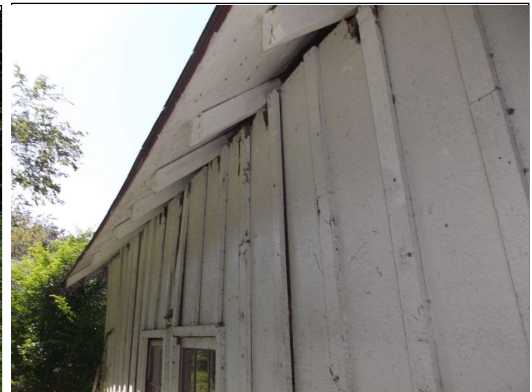
Defective and damaged
