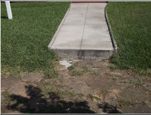
Walkway step too high and trip hazard
