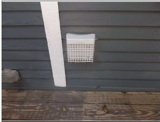
Improper dryer vent terminal
