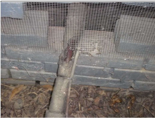
Missing refrigerant line insulation
