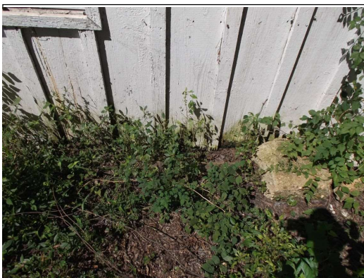
Soil contact siding and rot
