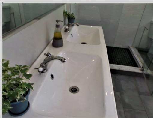
Little water flow from sink faucets
