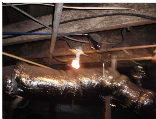
Mold like substance on floor joists
