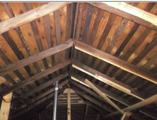
No collar ties on the rafters near the ridge
