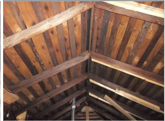
Defective rafter cuts to ridge boards
