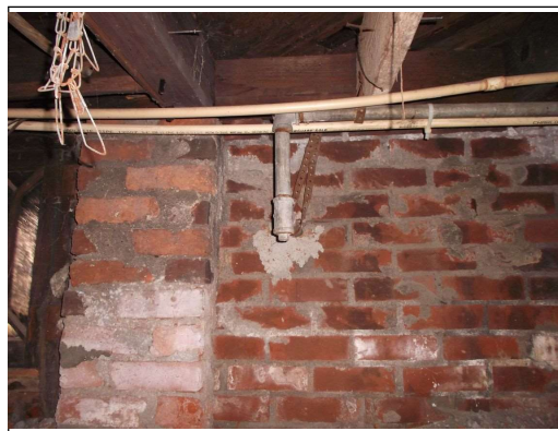
Water pipe for gas pipe in crawlspace
