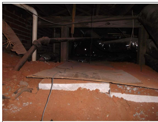
Missing moisture barrier and debris
