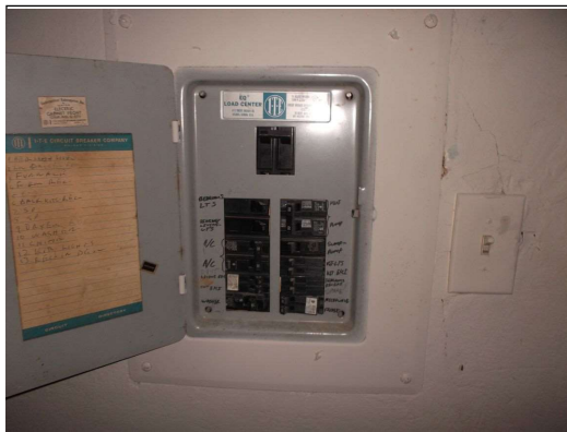
Panel too small for house
