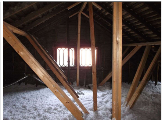
No gable venting
