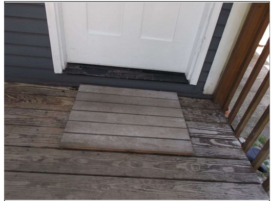
Rear door threshold not fully supported
