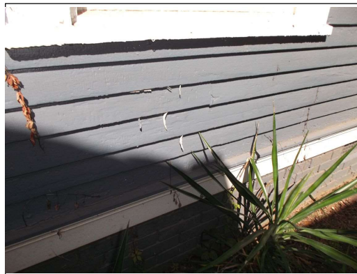
Paint peeling at siding
