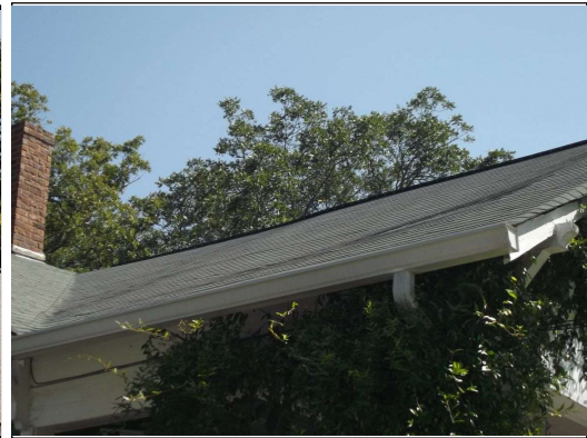
Dips at the roof deck at the left side
