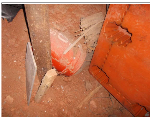
Missing moisture barrier/wet soil
