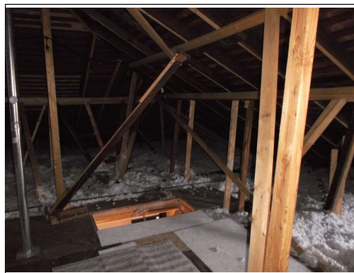
No eave venting
