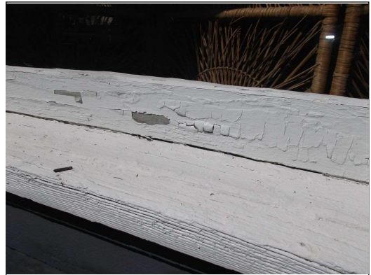
Paint peeling at windows
