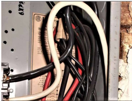
3 black or hot wires pigtailed at top of panel
