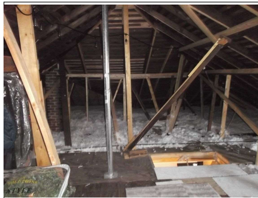
Defective roof brace supports
