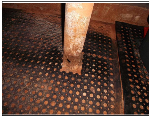
Steel posts rusting at the bottoms
