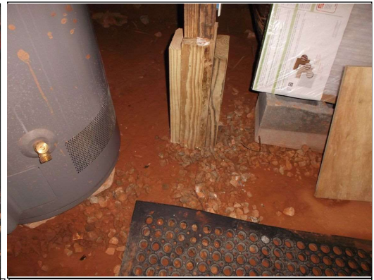
Wood posts in direct contact with soil
