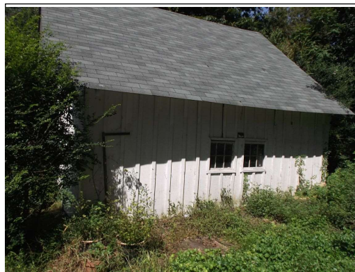
Soil slopes toward garage/no gutters
