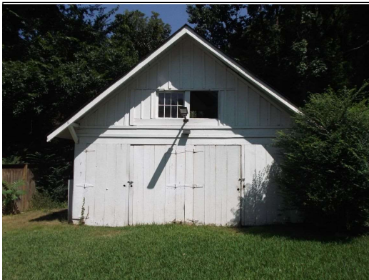
Doors need repair and adjusting
