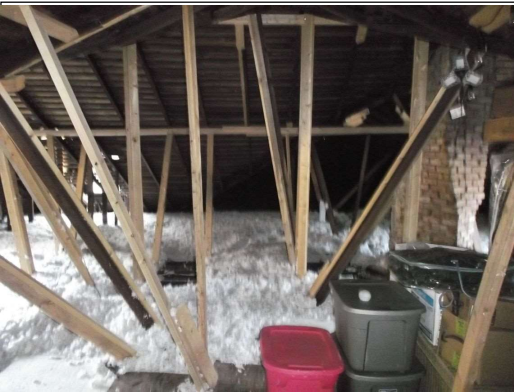
Defective roof brace supports/single 2x4s
