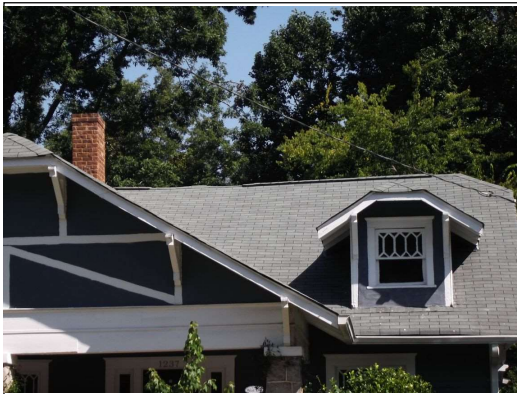
Main roof ridge sagging & slopes to left
