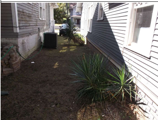
Poor soil grading and slope at right side
