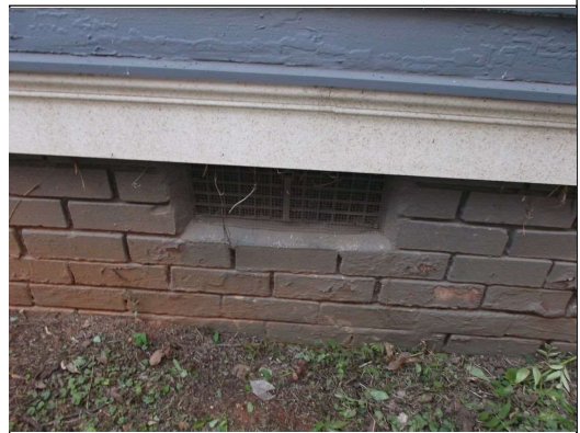
Foundation vents defective, damaged...
