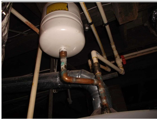
Expansion tank rests on water pipe
