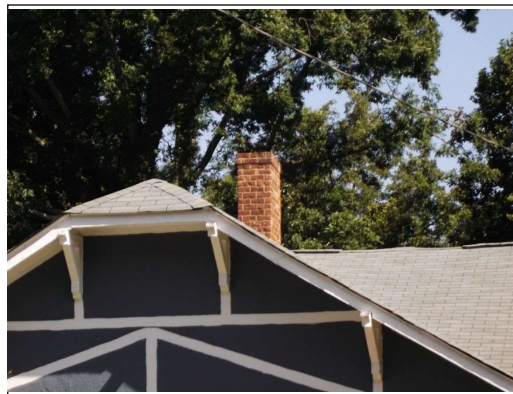
No rain cap nor spark screen at chimney
