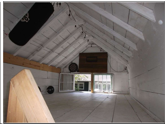
Cannot verify garage wired properly
