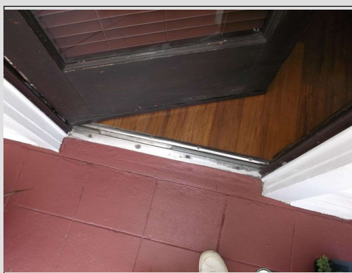
Front door threshold weather strip damaged
