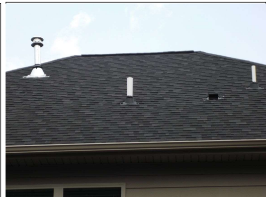
Wrong sealant @ metal pipes/sealant on pipe.
