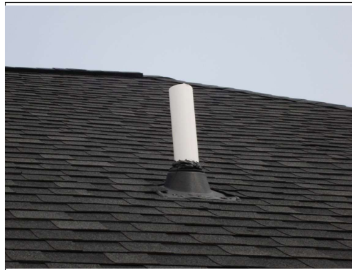
Flashing on top shingles, tar, nailed
