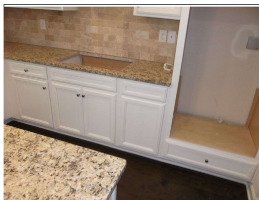
Missing cabinet knobs
