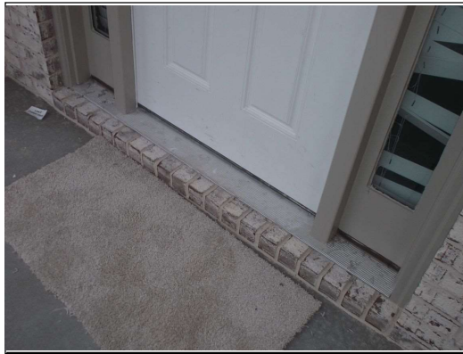
Front door threshold not supported
