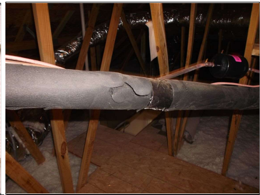
Damaged refrigerant line insulation at attic
