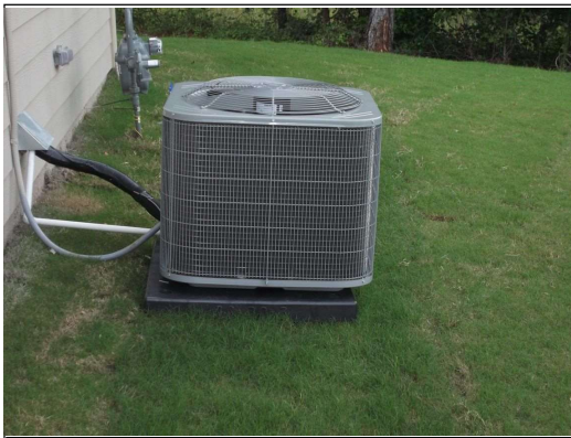
AC leaning away on the pad
