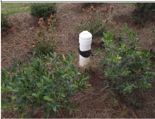
Pipe risers in the front yard
