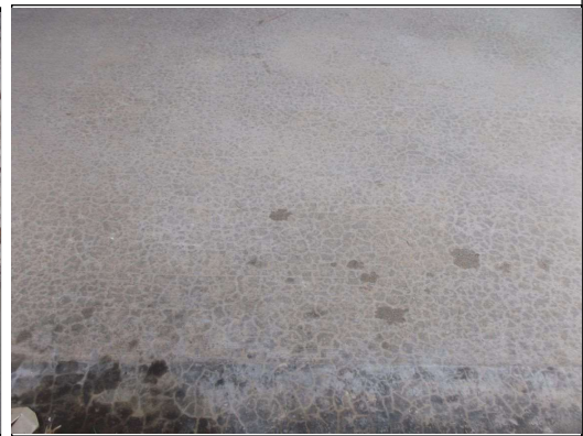
Spider cracks in patio floor
