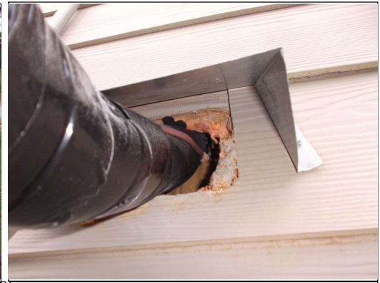
Opening in wall @ AC refrigerant lines enter
