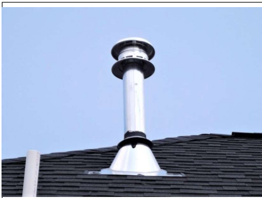
Flashing on top shingles face nailed
