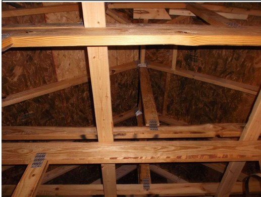
Ridge plywood not fully cut out at vent
