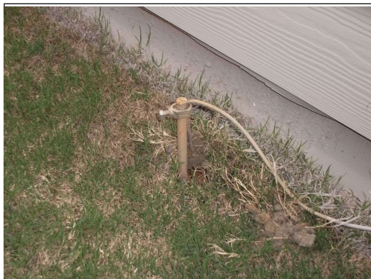
Ground rod too high above the ground
