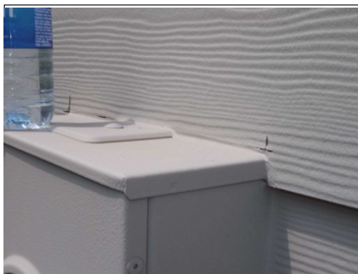
Missing caulk at the top of meter box
