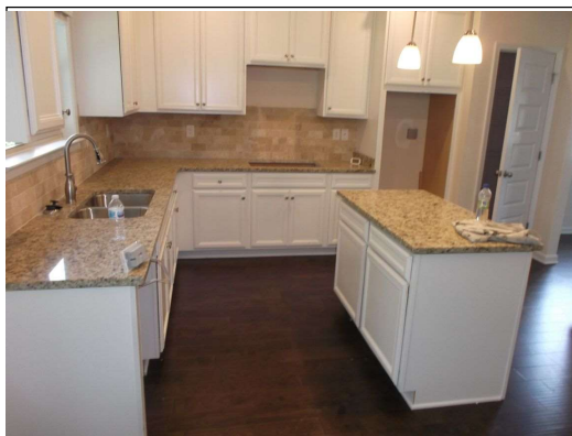
Appliances not installed
