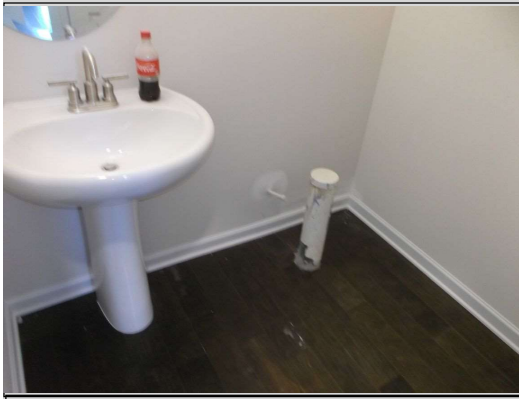
Toilet not installed
