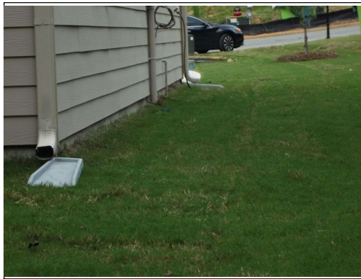
Poor soil grading
