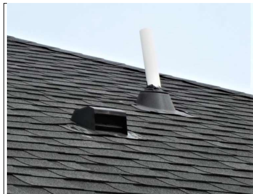
Flashing on top shingles face nailed
