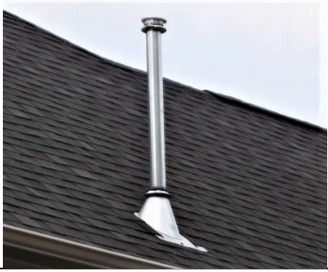
Pipe too high above roof
