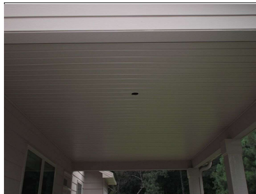
Missing light fixture at patio
