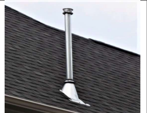
Pipe too tall/flashing on top shingles nailed
