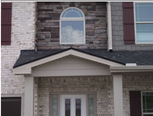
Painters residue on roof shingles
