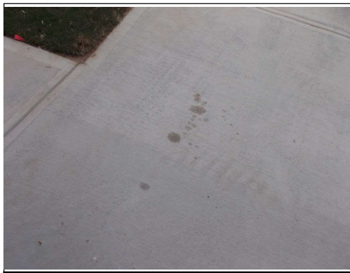
Oil in the driveway
