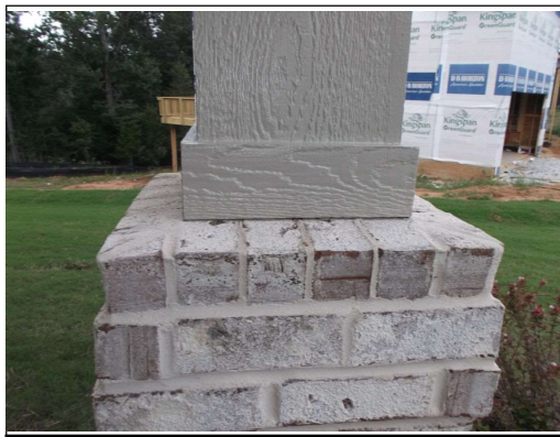
Missing bead of caulk at porch posts
