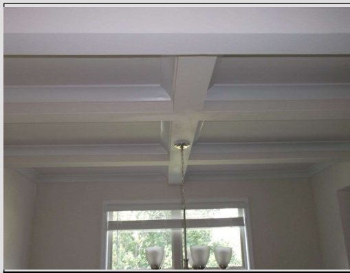
Incomplete finishing and painting
