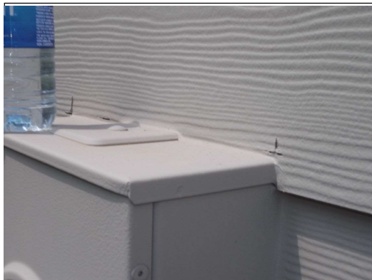
Missing bead of caulk across meter box
