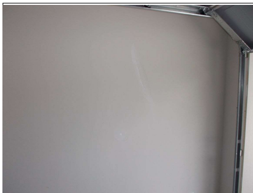
Wall needs painting
