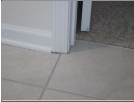
Gap at door frames and floor covering
