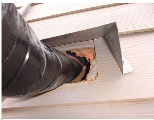
Open hole in the wall at AC lines
