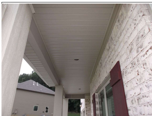
Missing light fixtures at front porch
