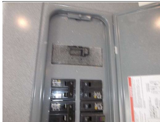
Paint on main breaker at panel
