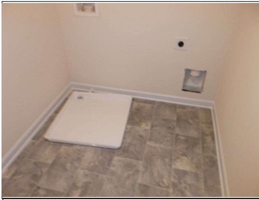
Drain pan incomplete/gaps at dryer box
