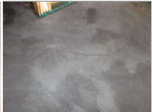
Hair line crack in floor
