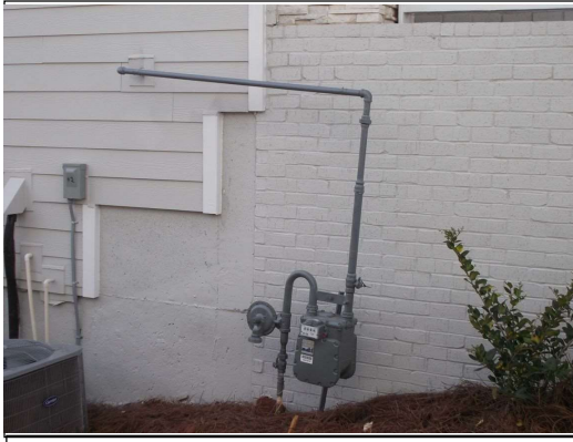
Gas meter to house pipes poorly installed
