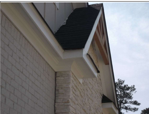
Missing short gutter front left side of garage
