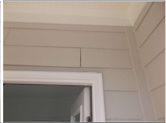
Excessive gap and siding not level
