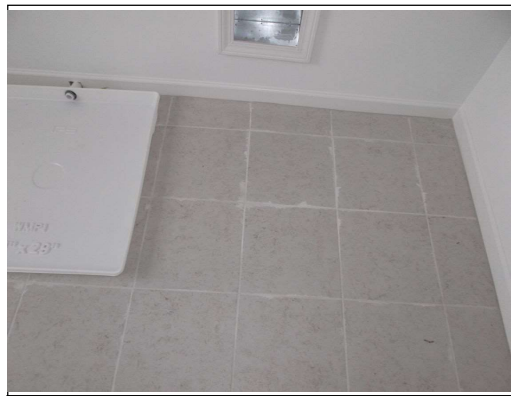
Grout spilled on floor tiles
