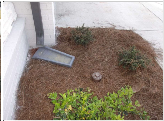
Poor soil slope away & debris under pine straw
