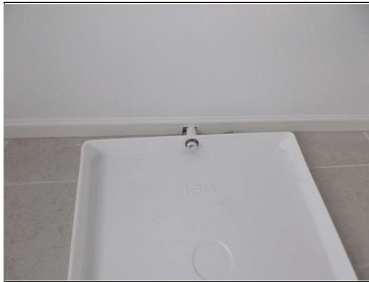
Missing caulk at hole in baseboard
