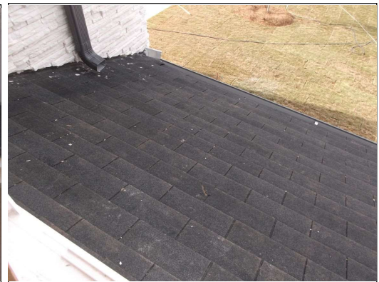
Workers residue & damage at porch shingles
