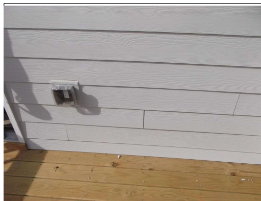
Excessive gaps between siding panels
