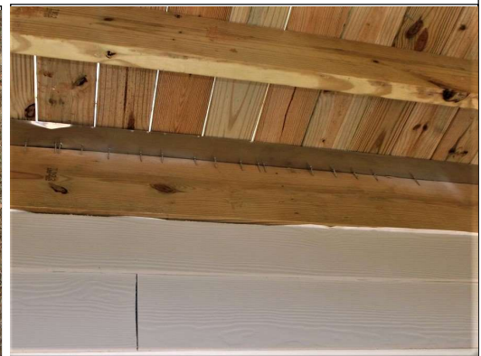
Many nails have punctured the flashing
