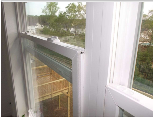
Master bed window will not snap in place
