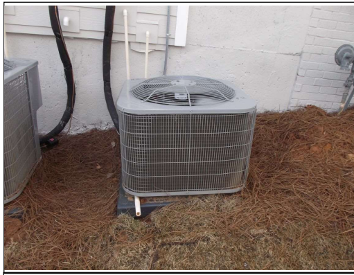
Right AC unit leaning to the left
