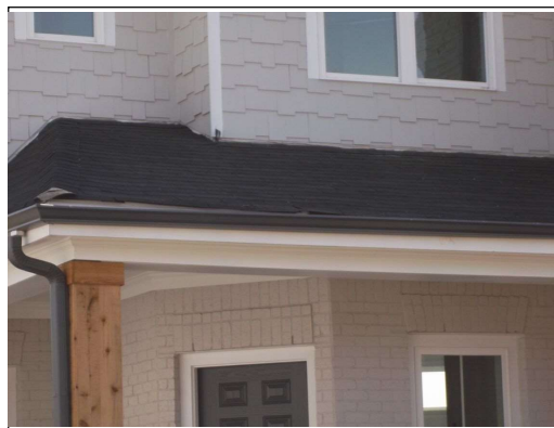
Shingle lifting at th front porch
