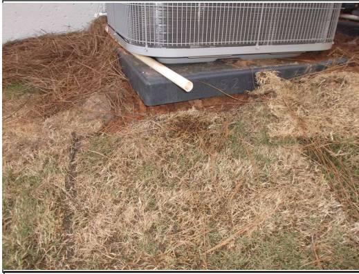
Missing soil under left AC base
