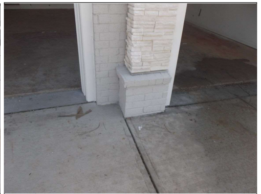
Weep holes not visible
