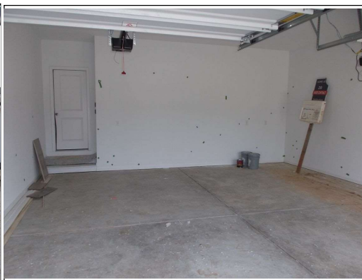
Tape indicating defective finish?
