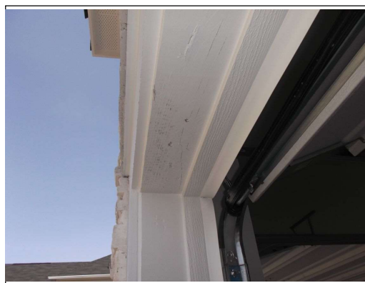
Defective door frame
