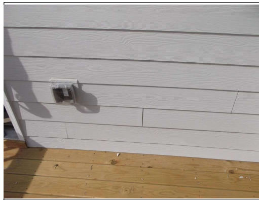
Gaps in siding at rear of house
