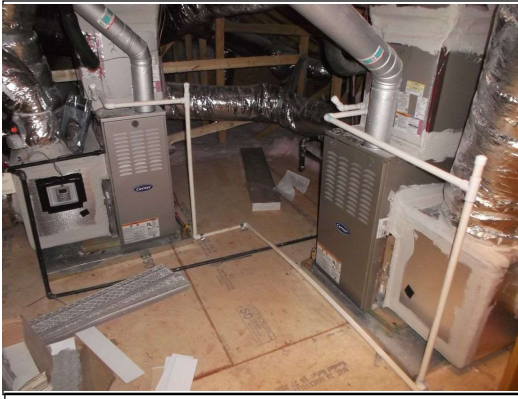
Right furnace has vibration when operating
