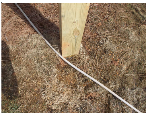
Deck posts in the soil/not enough pine straw
