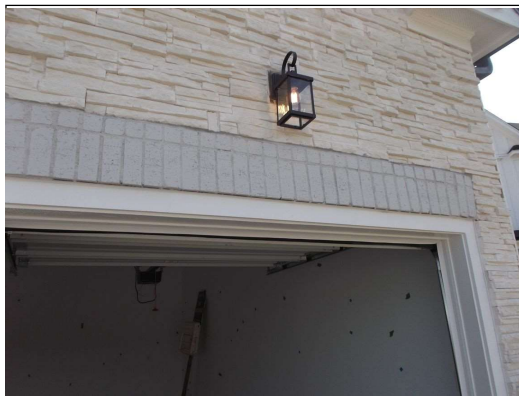
Missing weep holes?
