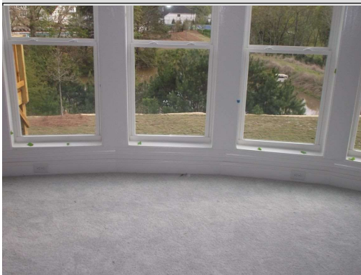
Windows not square in the wall
