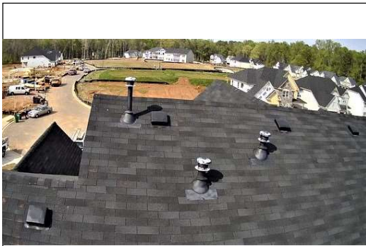
Pipe flashing on top shingles face nailed
