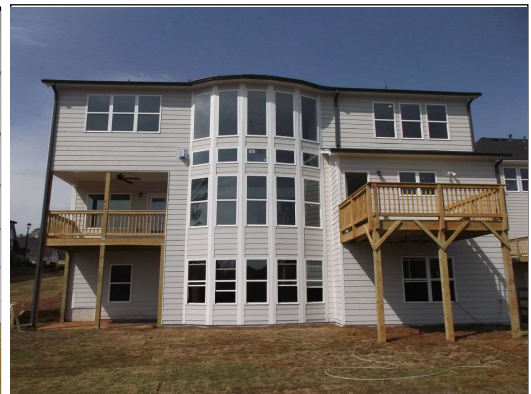
Gutter sagging at bay window & left side
