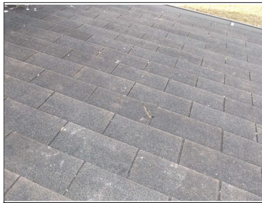
Damaged shingles at front porch roof
