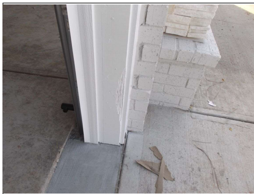
Damaged door frame
