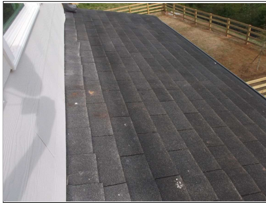
Workers residue on lower rear roof shingles
