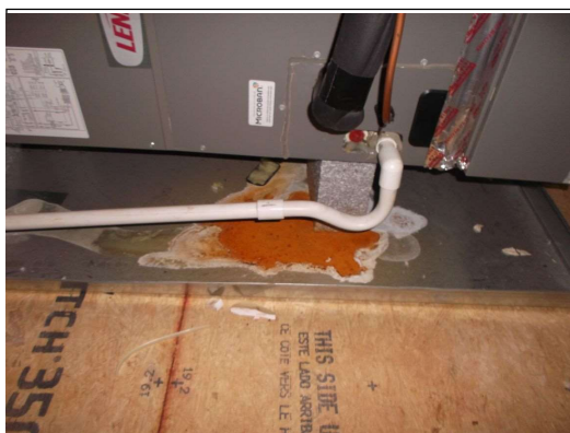
Calcium and rust in furnace drain pan
