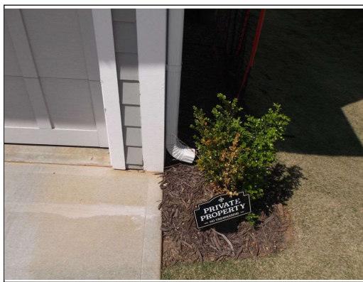
Downspout pour into soil right corner
