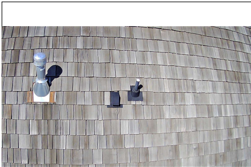
Flashing on top of shingles face nailed
