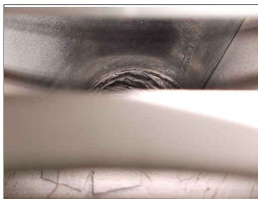
Slight dust in return air duct 1st floor
