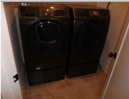
No washer drain pan installed
