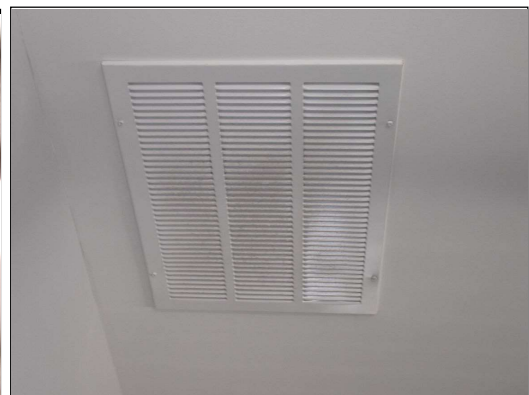
Dust on garage return register grill
