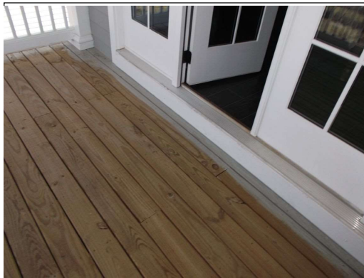
Painters residue on 3rd level floor
