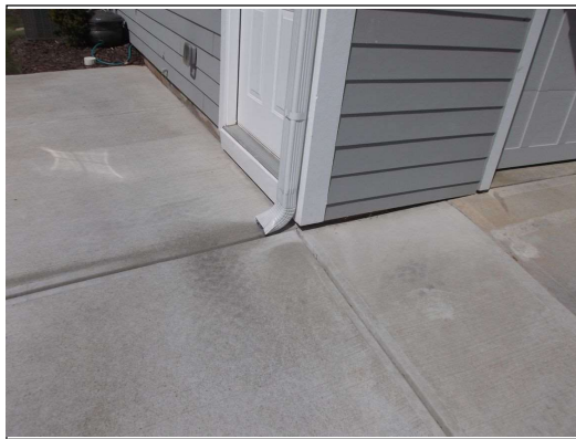
Downspout crushed left corner of garage
