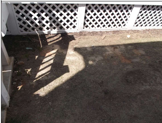
Soil erosion at the rear yard near the porch
