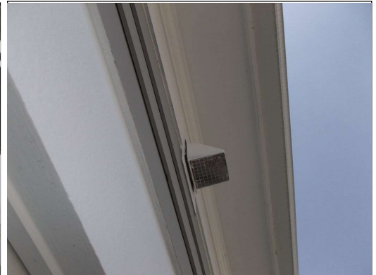
Missing caulk bead @ exhaust vents on wall
