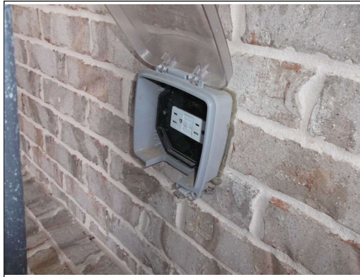
1st level exterior outlet restricts plug in
