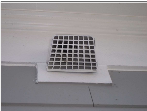
Wasp nest inside exhaust vent terminal
