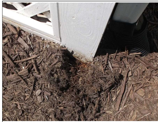
Rear deck posts contact soil
