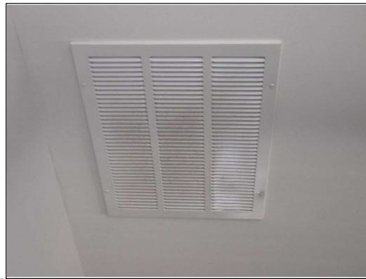
Return register grill cover has dust
