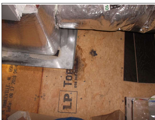
Water stains on attic floor
