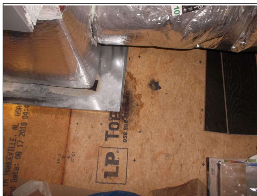
Dry water stains on attic floor at drain pan
