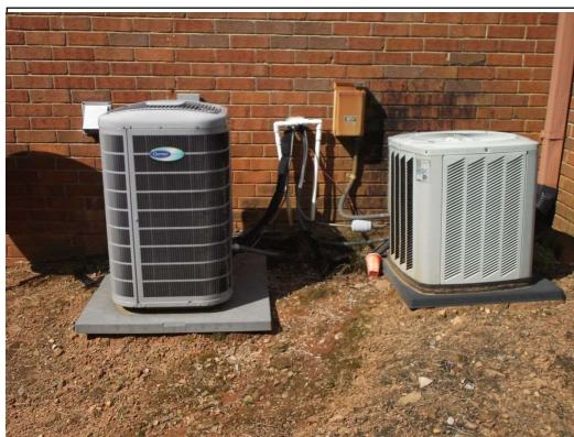
AC units located on the sunny side of house
