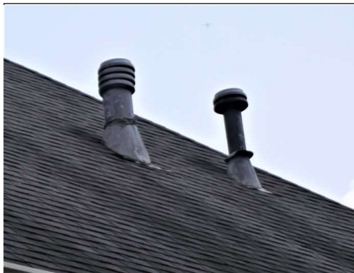
Missing rain collar left pipe/nails in flashing
