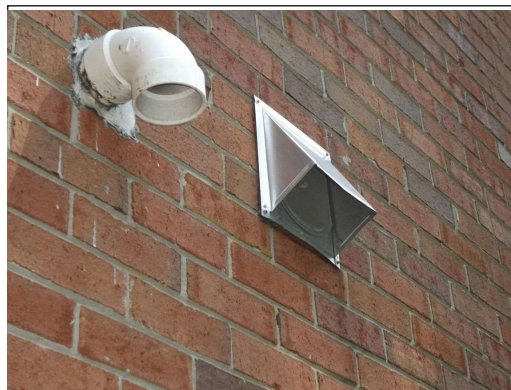
Missing caulk bead at terminals and fixtures
