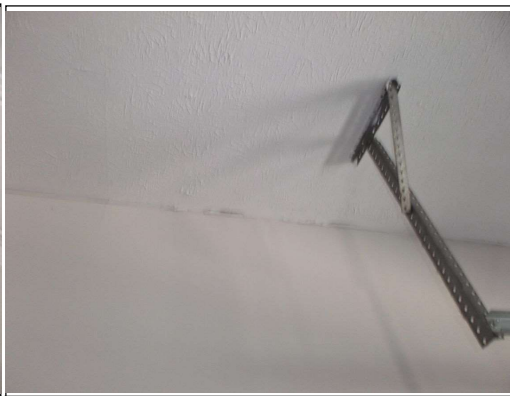
Tape peeling at ceiling to wall
