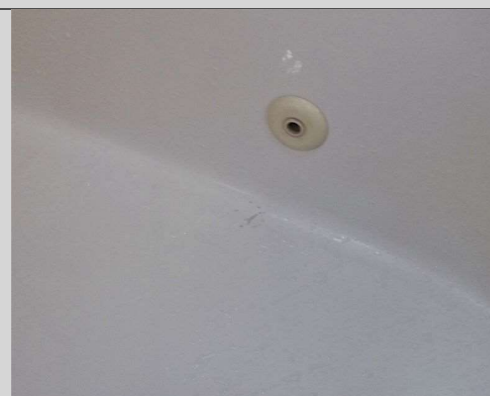
Cracks in tub fiberglass at floor
