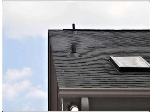
Flashing on top shingles face nailed
