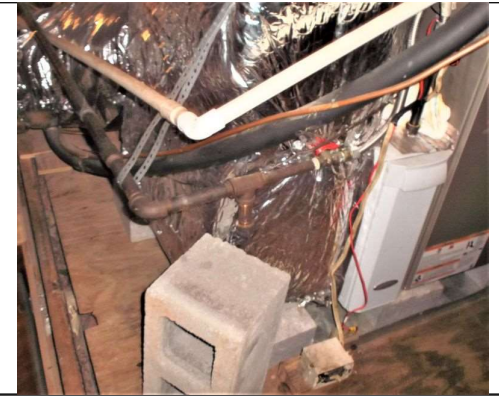
Improper sediment trap in gas pipe
