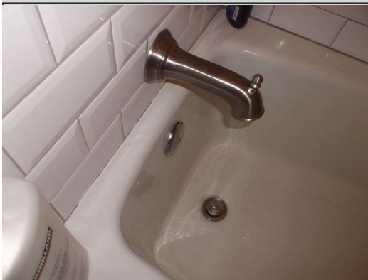
Tub overflow cap upside down
