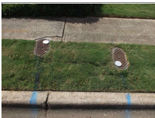
2 water meters at street
