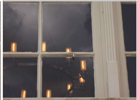
Paint peeling and broken glass
