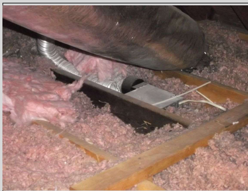
Exhaust fan duct disconnected
