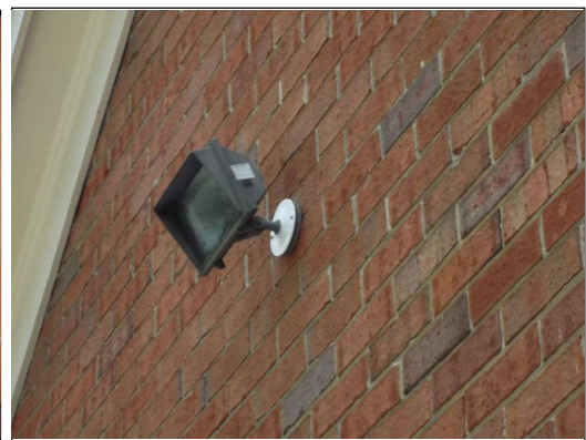
Missing bead of caulk around light fixtures
