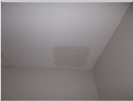
Incomplete ceiling repair
