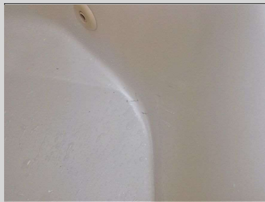
Cracks in fiberglass corner...
