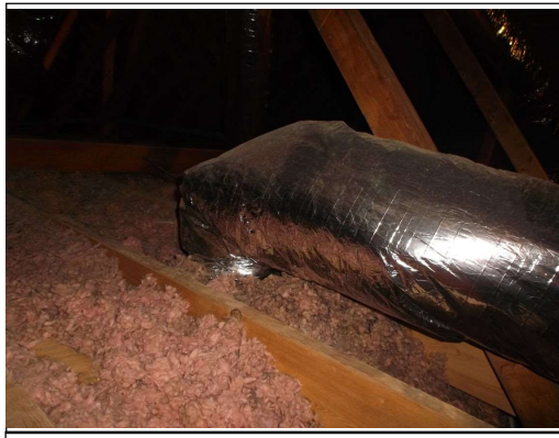
Partially twisted and crushed duct
