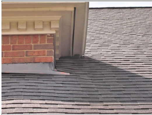
Debris in gutter
