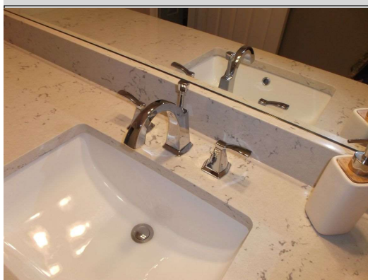
Sink faucet loose at the base
