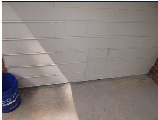
Siding damage at basement level
