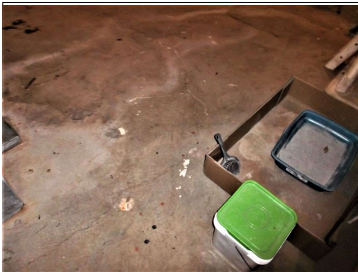
Moderate cracks in utility room floor
