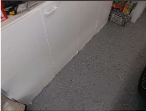
Water damage to cabinet doors
