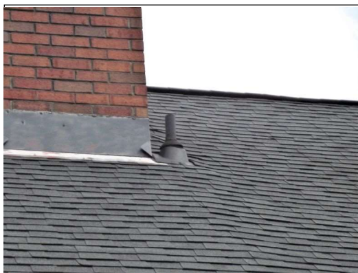
Flashing on side flashing face nailed
