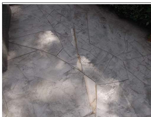
Outer kitchen floor settling, cracking, rotating
