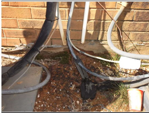
Missing refrigerant line insulation
