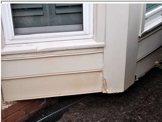
Water damage at front bay window
