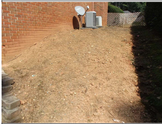
Major soil erosion at left side of house
