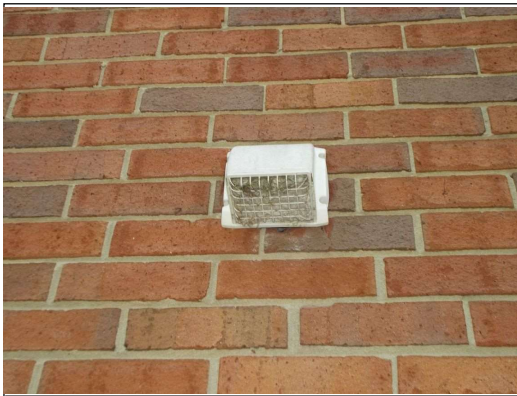
Improper dryer vent and clogged with lint
