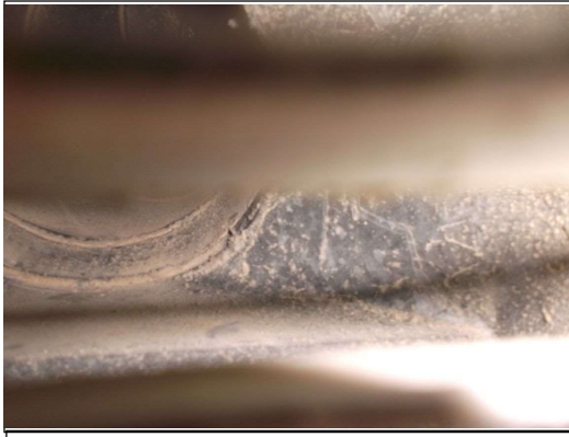
Air return duct dusty
