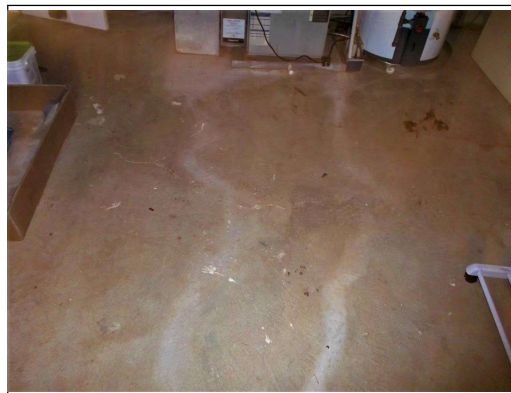
Stains on floor and cracking
