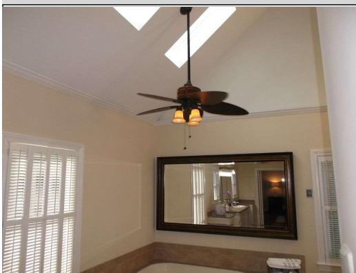
Ceiling fan closer than 8 feet from tub
