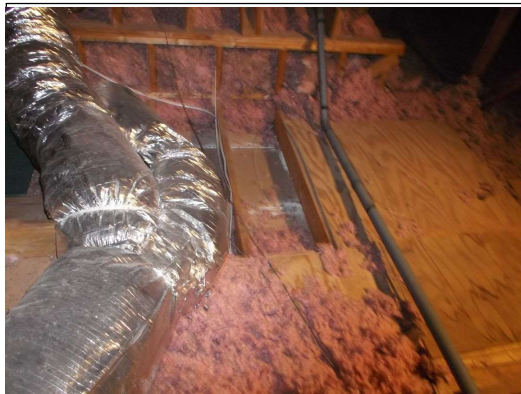
Missing ceiling insulation
