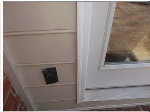
Damaged siding left side of patio door
