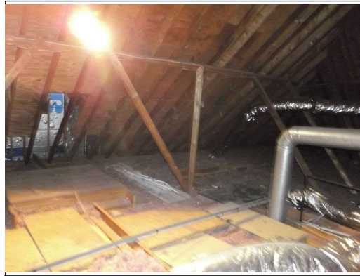
Flooring weak and poorly placed
