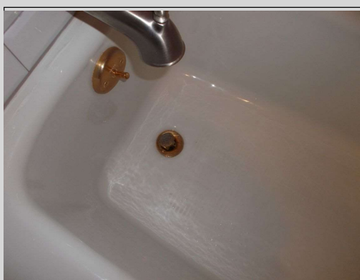
Tub stopper appears defective
