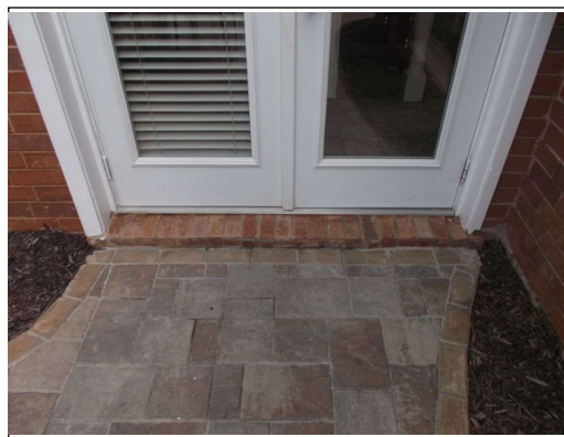
Missing bead of caulk at threshold on brick
