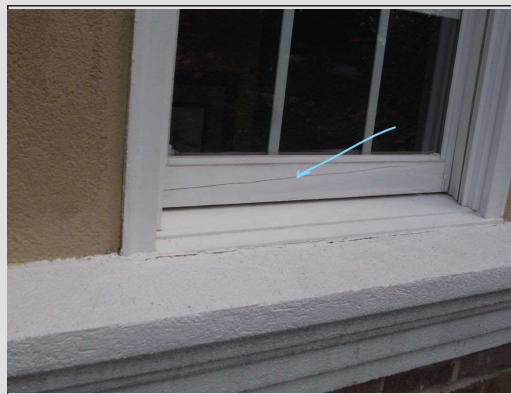
Split in window sash at the front right
