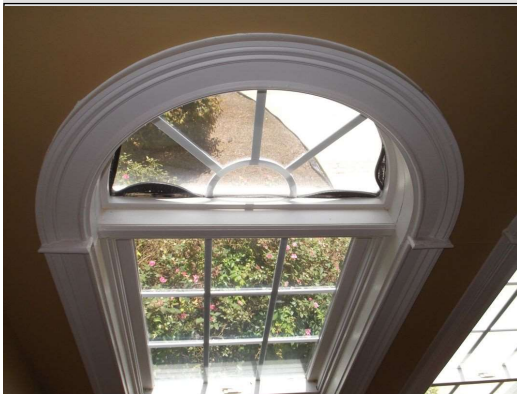
Stairwell window seal defective
