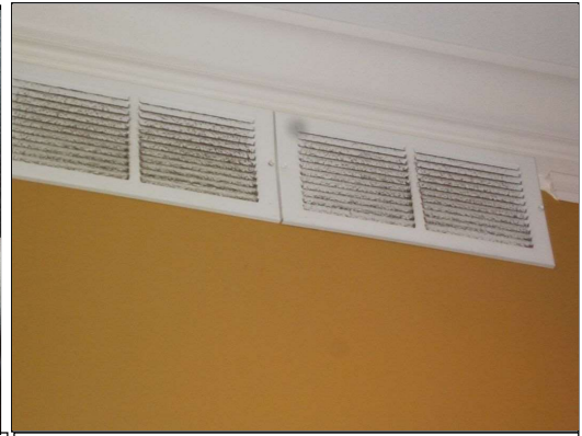
Air duct system dusty
