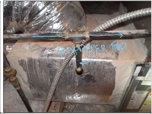
Improper sediment trap in furnace gas pipe
