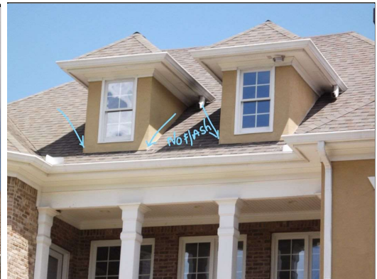
No flashing extending out of stucco
