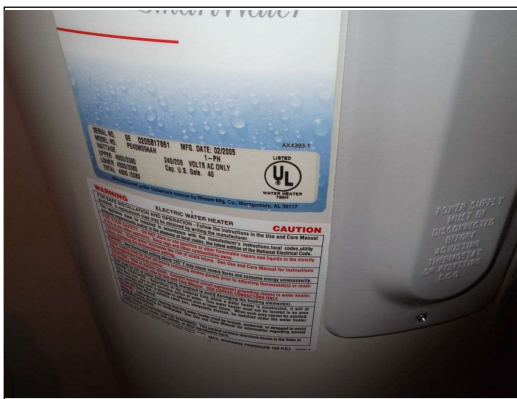
Water heater date 2005 is at end of use
