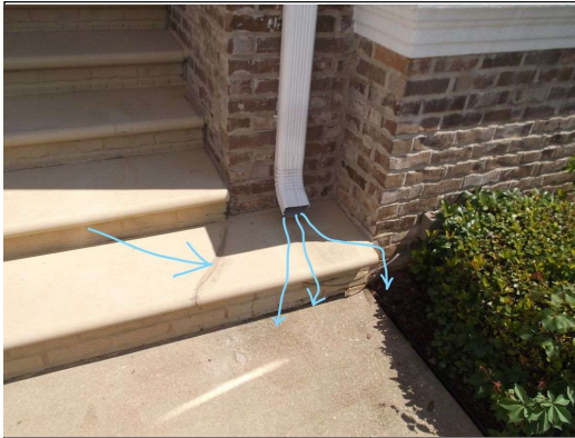
Settling crack front stairs, cause downspout
