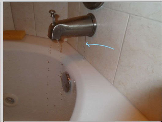
Tub faucet drains water back onto wall
