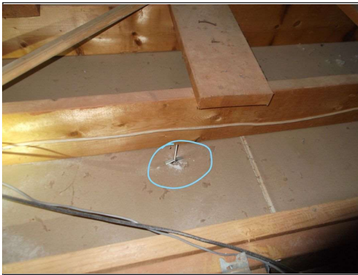
Garage ceiling lights attached to sheetrock
