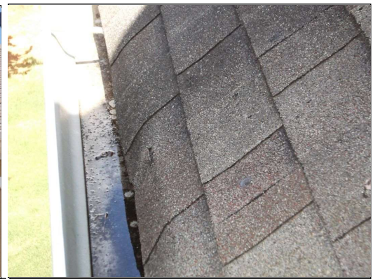
Shingle damage at the rear roof
