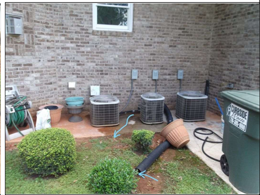
Poor soil slope and missing ground cover
