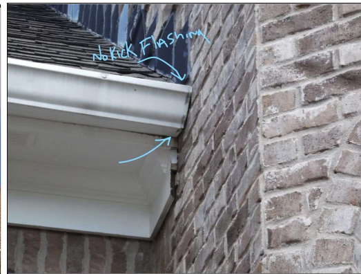
Roof water bypass flashing @ front of house
