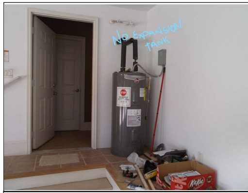
No expansion tank above water heater
