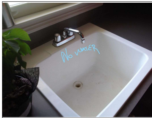
No water at the laundry sink
