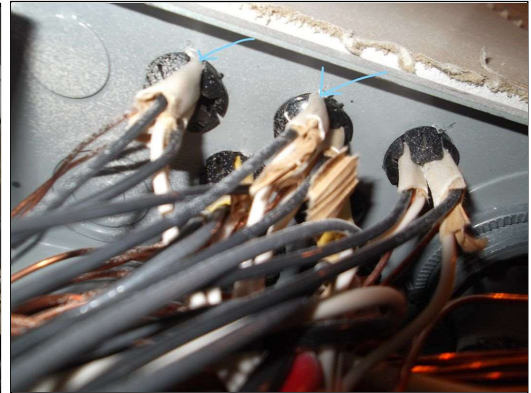
Electrical cables contact sharp metal in panel
