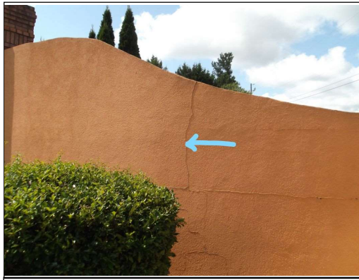
Settling cracks in masonry fence wall
