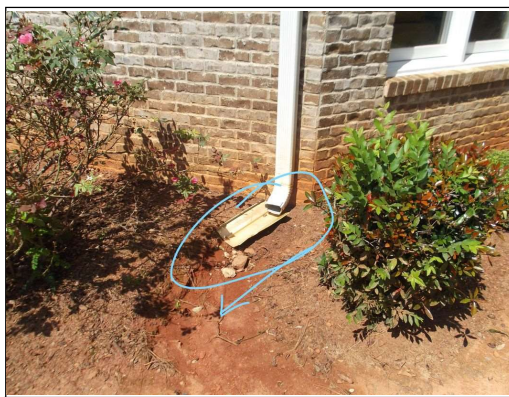
Soil erosion at downspouts
