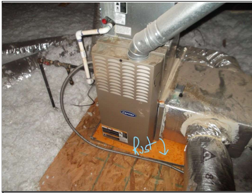
Rust in attic furnace drain pan
