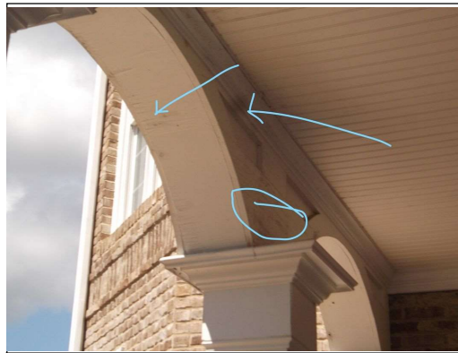
Front porch wood trim water damage
