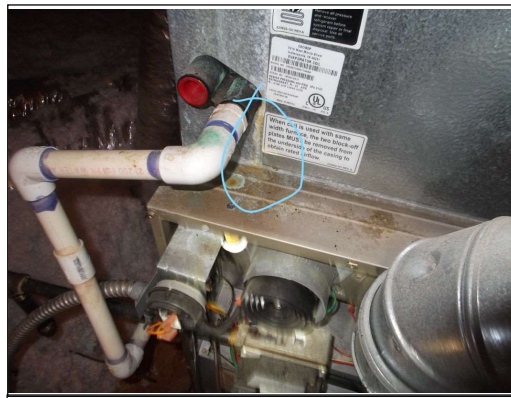
Rust at air handler at attic furnace
