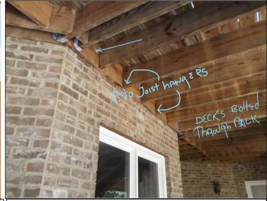
Wood deck unsafe, bolted through brick
