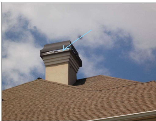
Chimney cap needs painting
