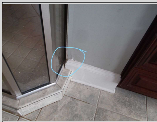
Slight water damage at master bath shower
