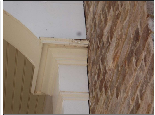
Front porch post water damage
