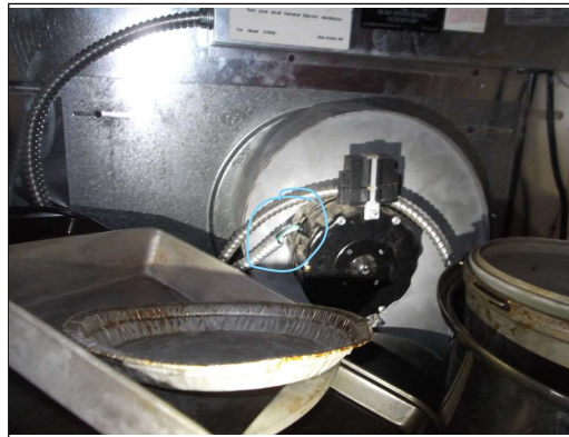
Damaged conduit at the stove exhaust fan
