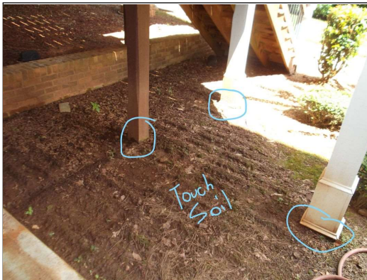
Wood deck support posts contact soil
