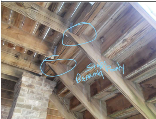
Deck stairs poor bearing on deck rim joist
