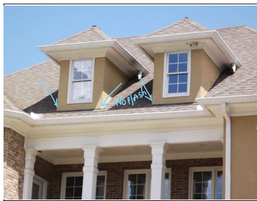
Cannot see flashing extending out stucco
