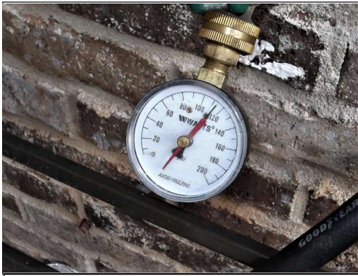
Water pressure 112 is too high
