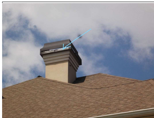
Paint peeling at chimney cap
