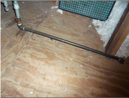
Gas pipe not supported and secured to floor
