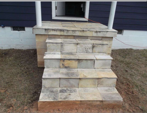
Need handrails/floor slope away/loose tiles
