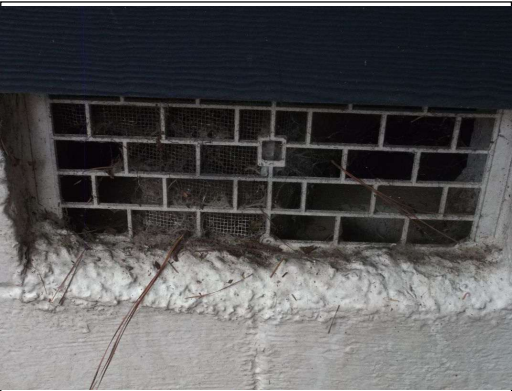
Vent needs replacement
