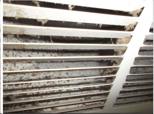
Air duct dusty
