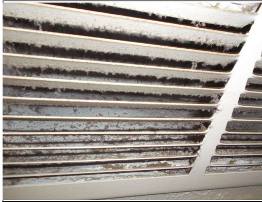
Air duct dusty
