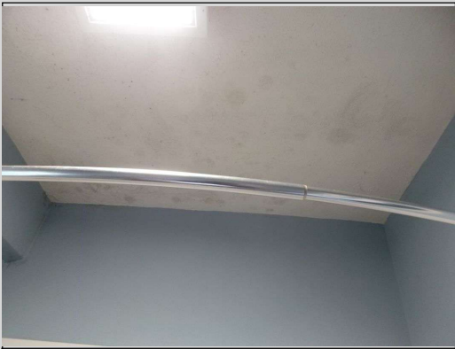
Stains in bath ceiling
