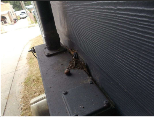
Missing bead of caulk over box
