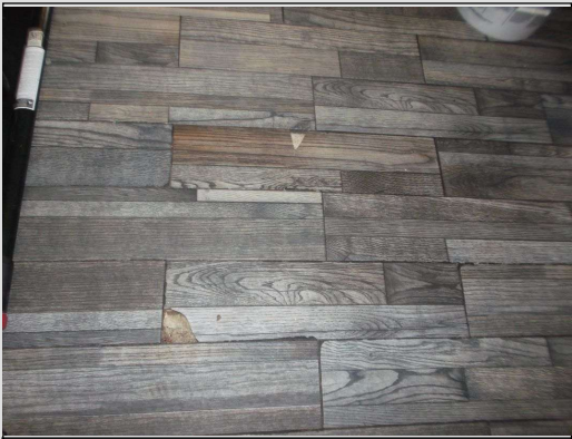
Broken and damaged tiles
