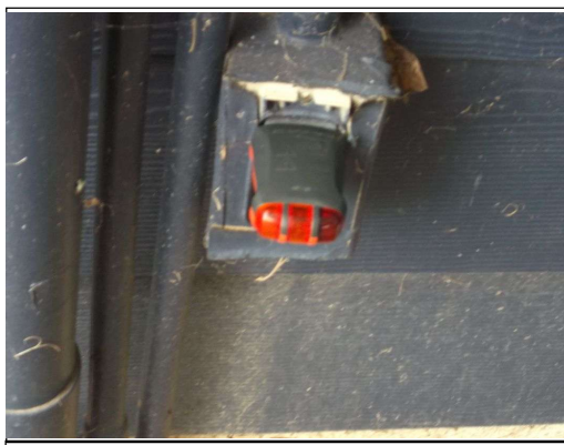
Receptacle not energized
