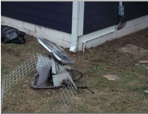
AC detached and damaged
