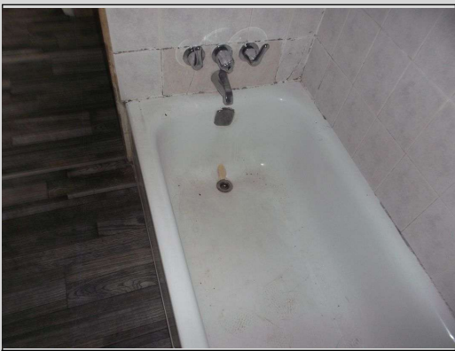
Stains in tub, broke tiles, faucet handles loose
