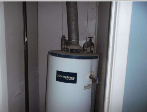
Galvanized water pipes may have rust inside
