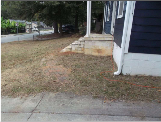
Walkway need relay/porch floor slope away
