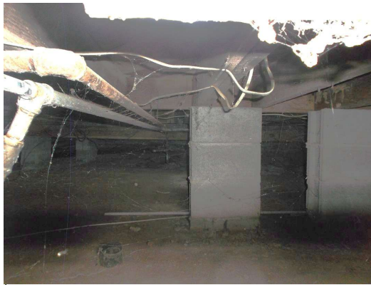
No plastic on the ground
