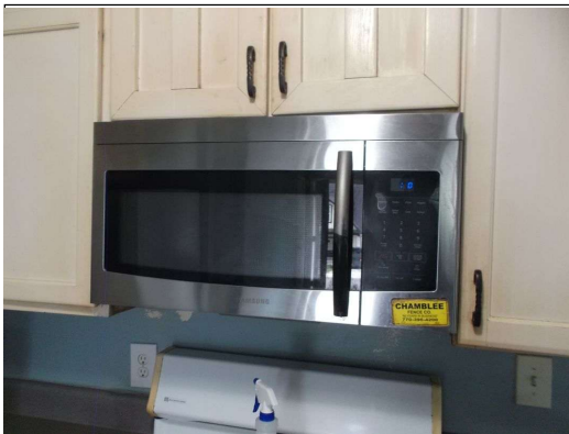
Microwave not working properly
