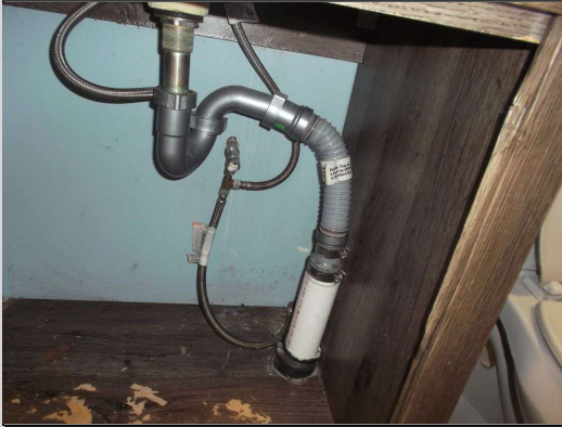
Sink drain pipe is a S-Trap unsafe
