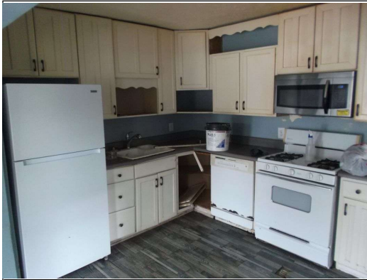
Cabinet damage, floor sinking
