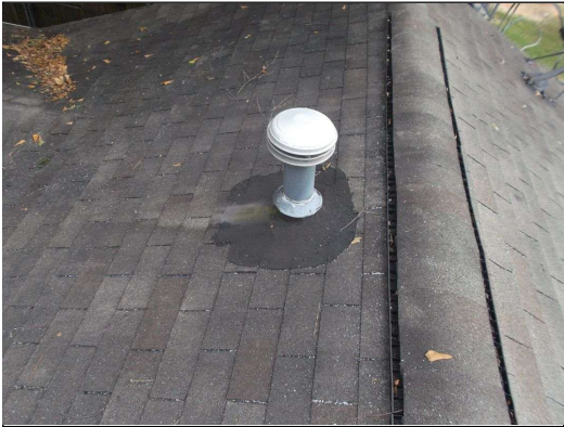
Tar around flashing and pipe
