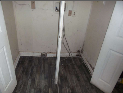
Floor sink, mold on wall, no drain pan
