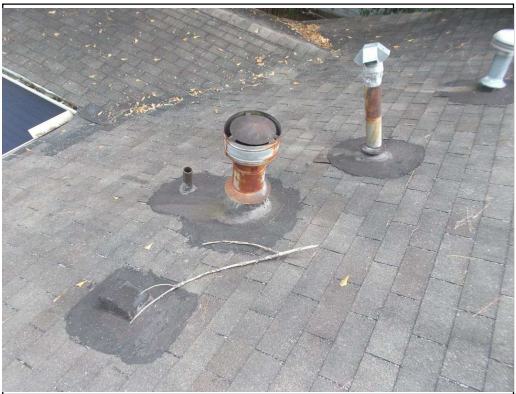
Tar around flashing and boots
