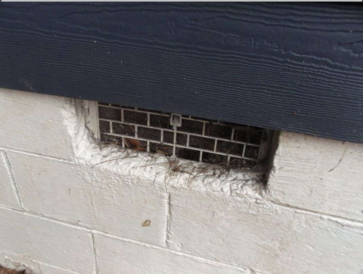
Vent need replacement
