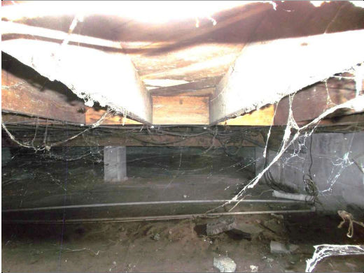
Missing moisture barrier plastic
