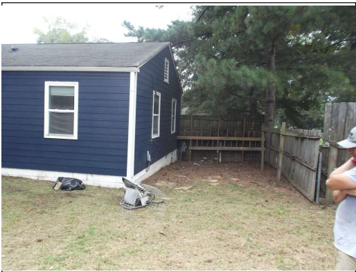
Poor soil slope away
