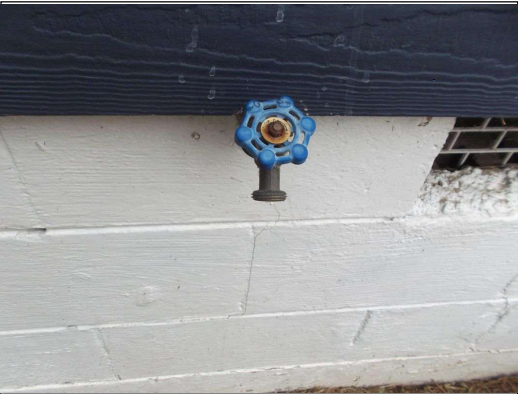
Missing anti siphon devices at hose faucets
