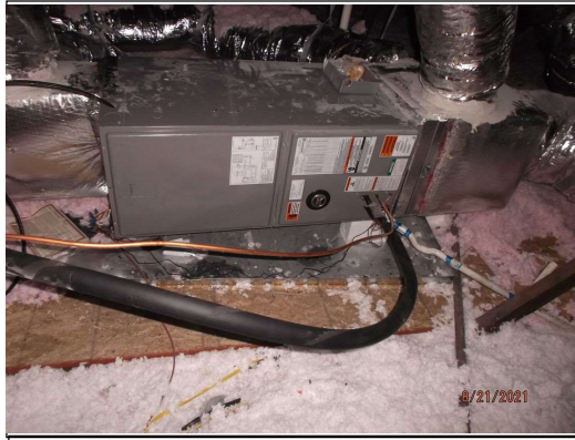
Furnace makes whistling noise operating
