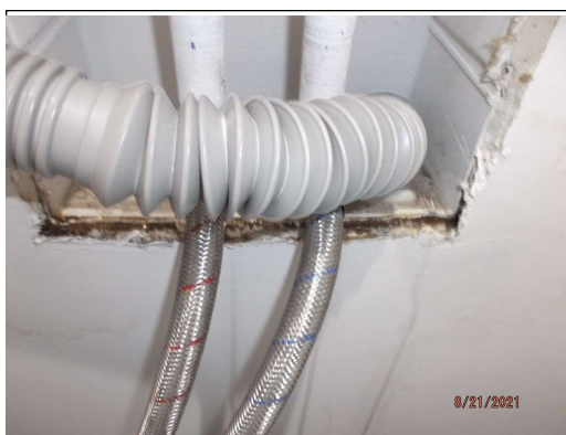
Pipes leaking at the washer hookup box
