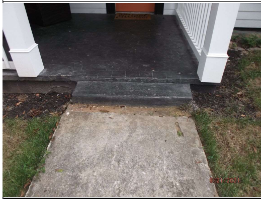
Front steps uneven and trip hazard
