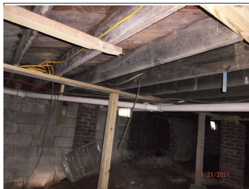
Fungus on floor framing
