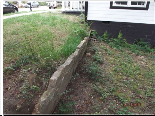
Retaining wall major leaning and no holes
