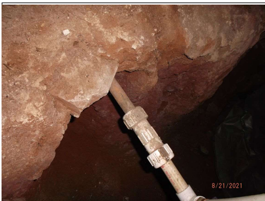
main water pipe steel?
