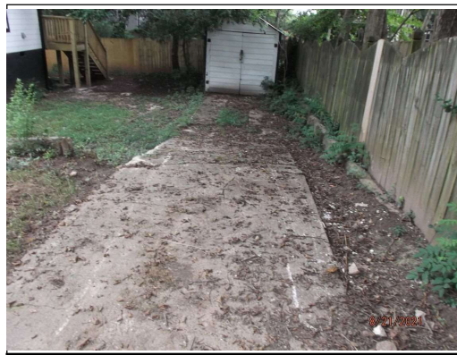
Driveway major damage and steep
