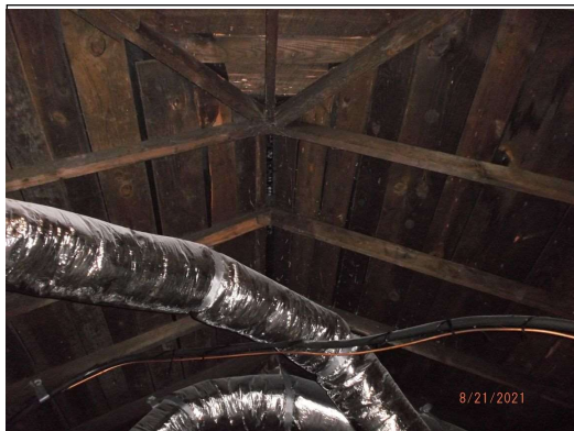
Not enough ridge ventilation
