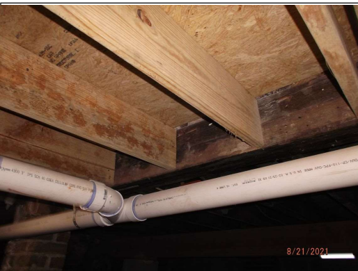
Missing joist hangers or 2 by 2 ledger at areas
