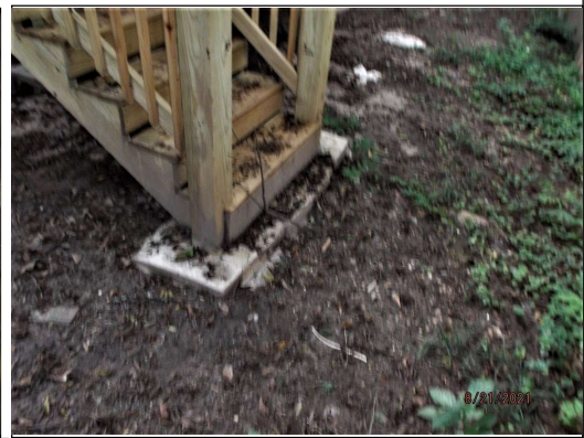
Missing stoop and no handrails
