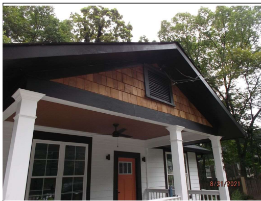
Missing flashing where shingles rest on beam
