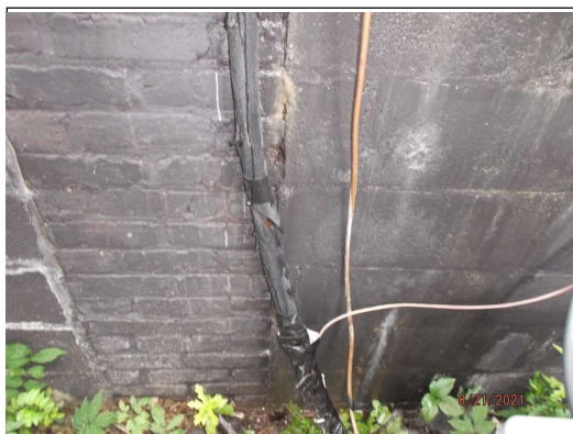
Deteriorated refrigerant line insulation
