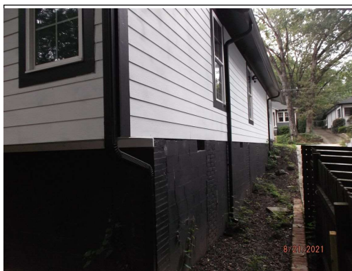
Foundation vents missing at all sides
