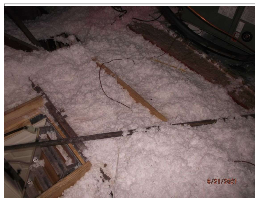
Missing service floor leading to furnace
