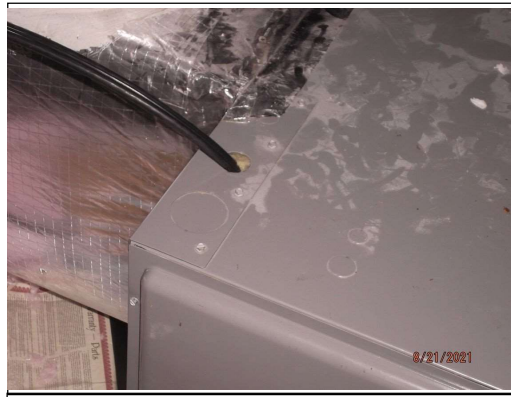
Electrical cable contact sharp metal in hole
