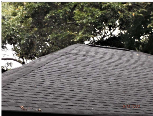
Ridge vent too small/hump in roof shingles
