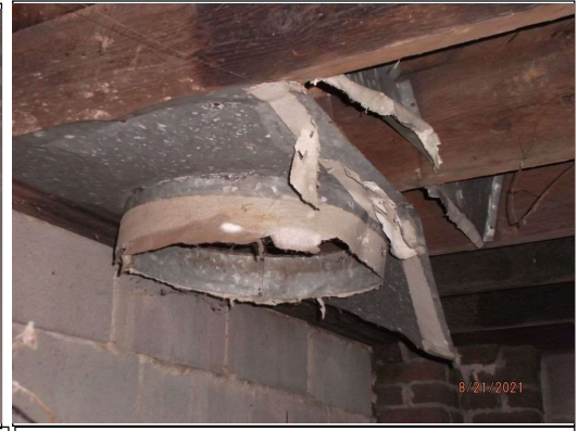
Damaged Asbestos remains on old metal duc
