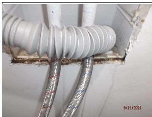
Pipes leaking into wall and floor
