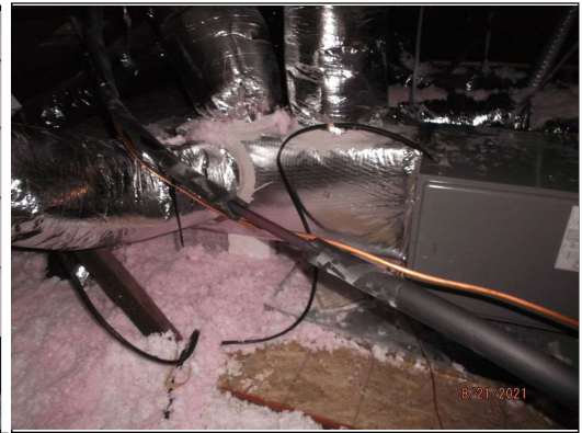
Missing refrigerant line insulation at attic
