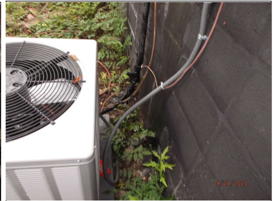
AC conduit not clamped to foundation wall
