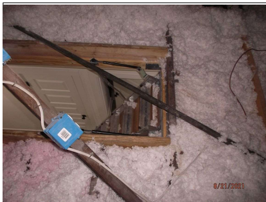
Pipe crosses over stair entry safety issue
