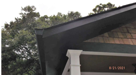
Missing drip cap flashing at fascia boards
