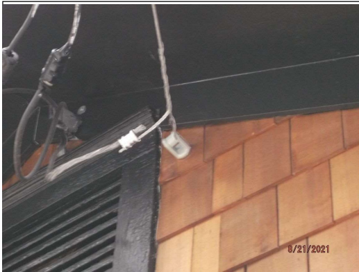
Improper service cables anchor
