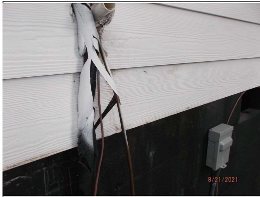
Damaged refrigerant line insulation
