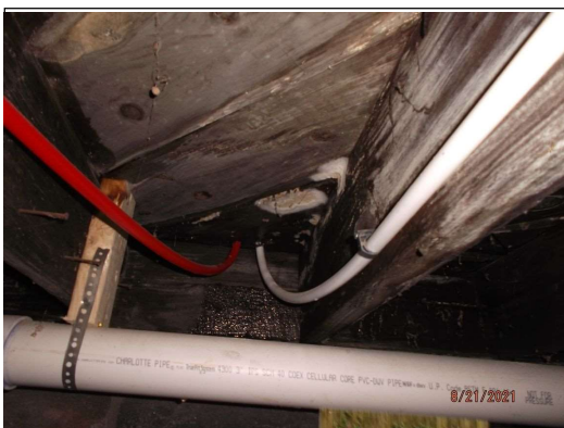
Laundry room water pipes leaking water
