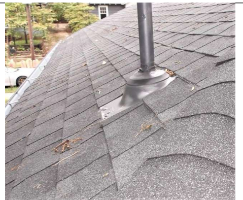
Flashing on top shingles and face nailed
