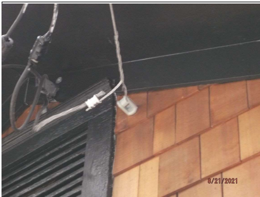
Improper anchor for service cables
