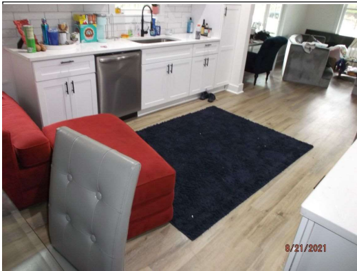
Floor sagging and slopes to sink wall
