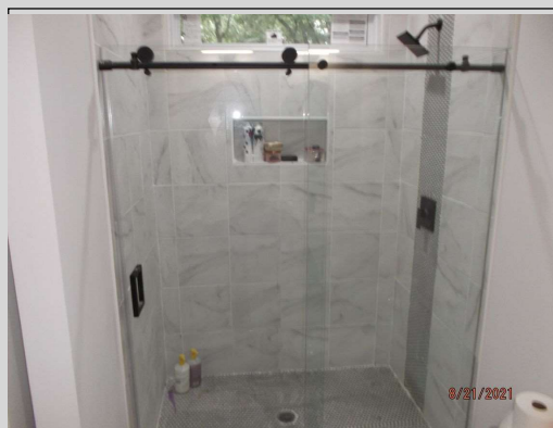
Shower head loose/poor floor tile installation
