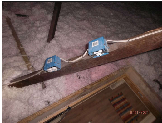
Missing outlet covers
