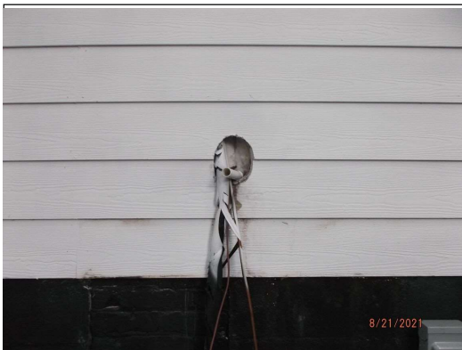
Hole in wall at AC pipes and no hood
