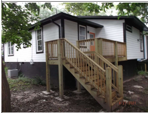
Deck missing bolts at house and missing post
