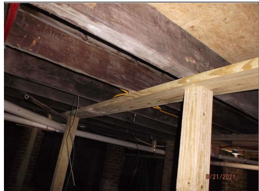
Improper wood for a beam
