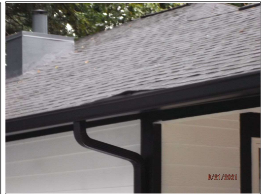
Hump in shingles left side
