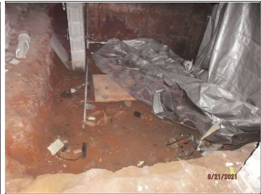
Debris and missing moisture barrier
