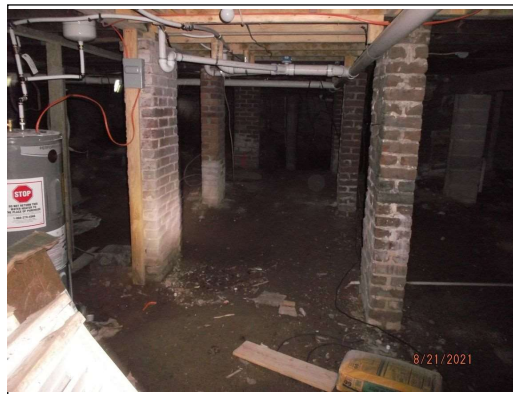
Soil wet, debris, no moisture barrier
