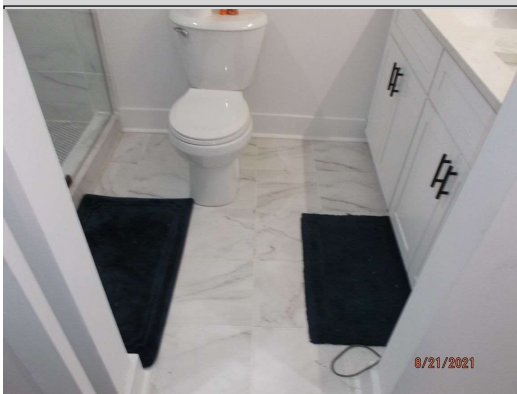
Missing caulk where toilet rest on the floor
