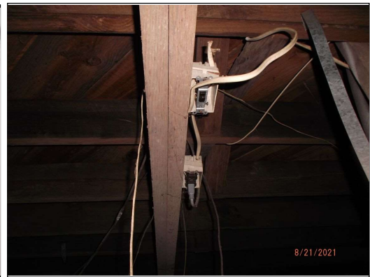
Missing box covers in the basement
