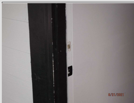
Missing strike plate at the front door
