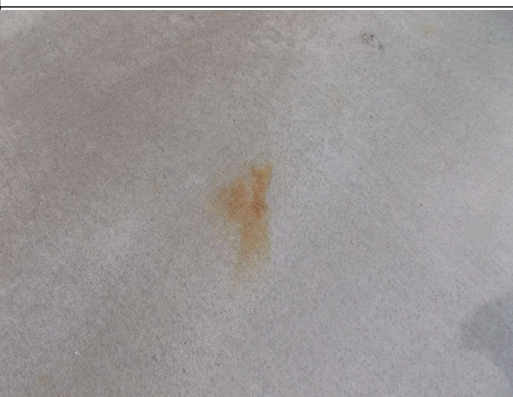
Stains in the driveway
