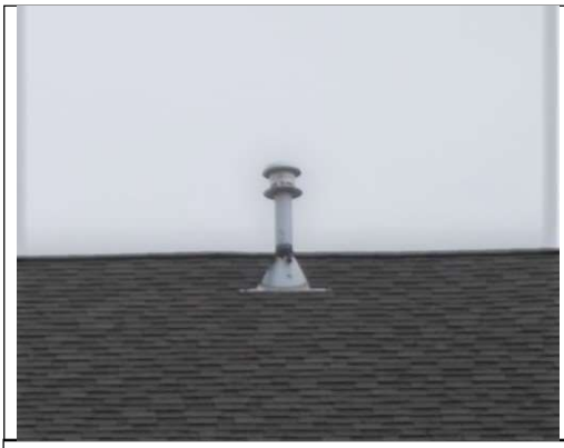
Flashing on top shingles face nailed
