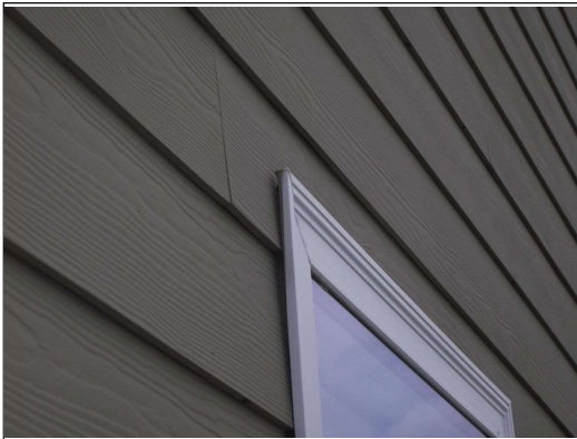
Missing flashing over windows
