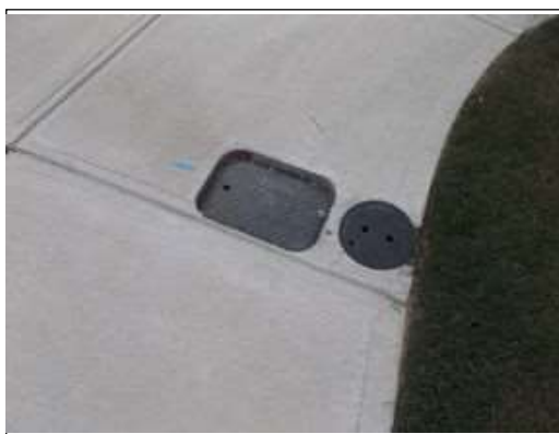
Water meter hole in sidewalk trip hazard
