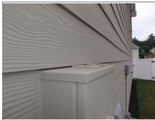
Missing bead of caulk across top of panel
