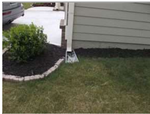
Poor soil slope away from side of garage
