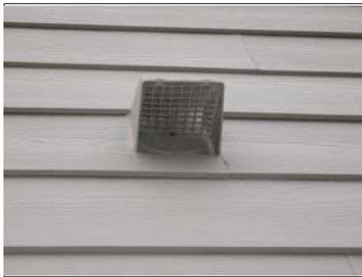
Dryer vent blocked and grill improper
