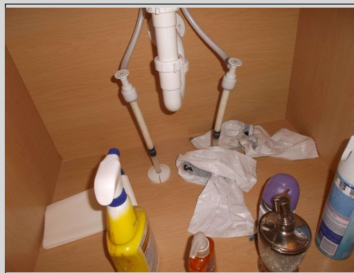
water pipes in storage area
