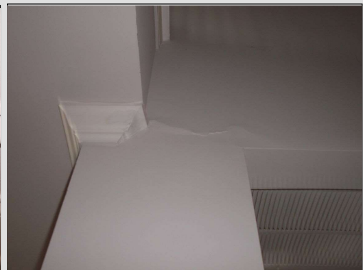
Sheetrock crushing at stairwell post
