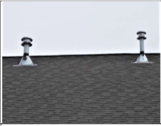
Missing rain collars on gas vent pipes & tar
