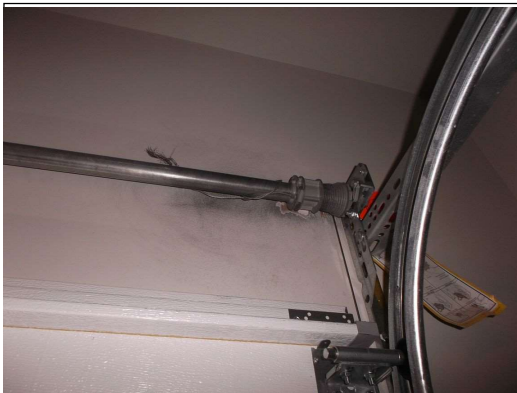
Excessive door tension cable damaging wall
