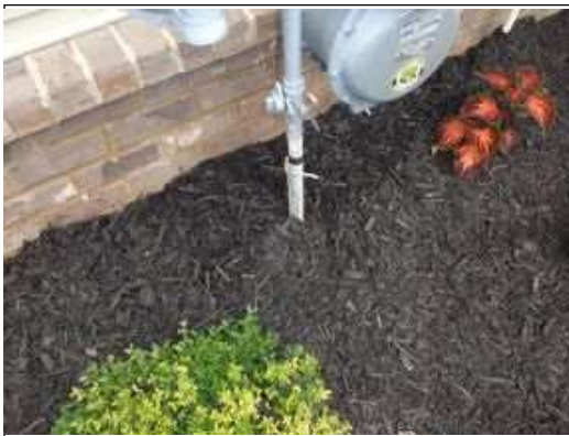
Ground wire not clamped to gas pipe
