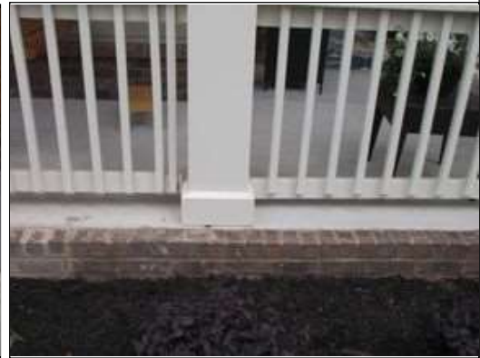
Railings not even at post connection
