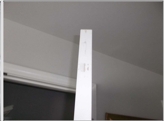
Double doors rub and defective paint
