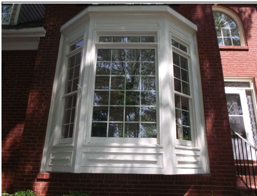
Water damage to wood painted over
