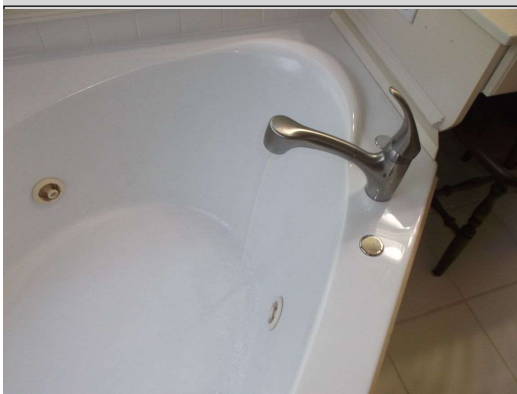
Low water flow at tub faucet
