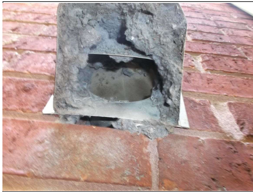
Vent terminal clogged with lint
