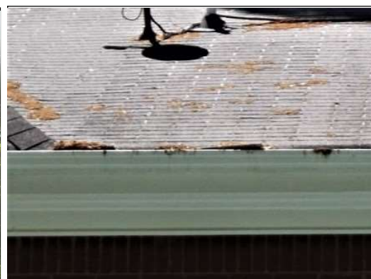
Debris in gutters
