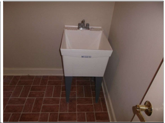
Wash sink not bolted to floor and wall
