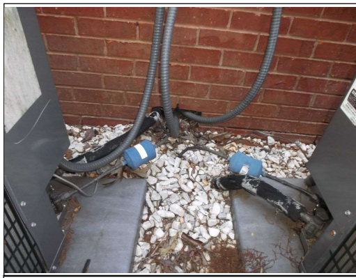
Refrigerant line insulation worn
