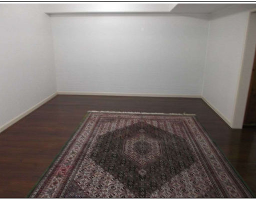
Missing outlets around room walls several rm
