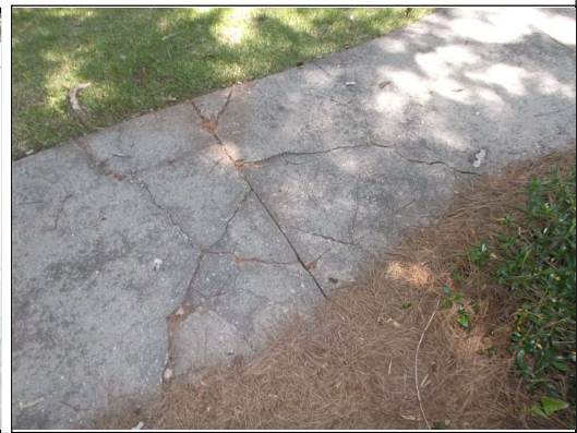
Major cracking in the walkway near driveway
