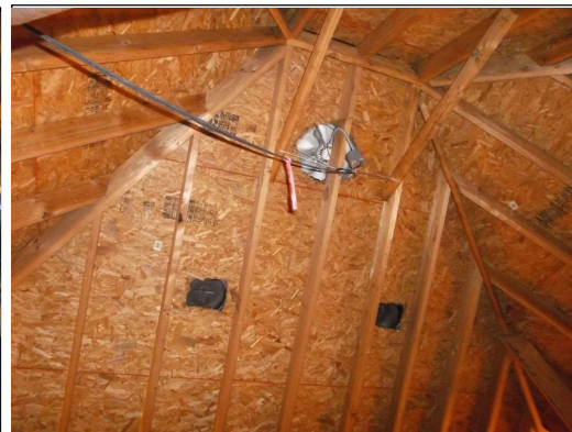
Missing spacer between OSB panels
