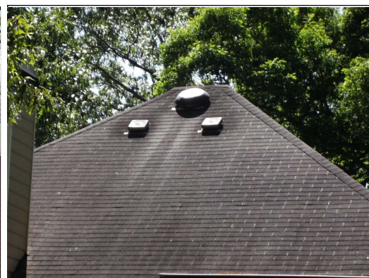
Roof worn, vent flashing on shingles nailed
