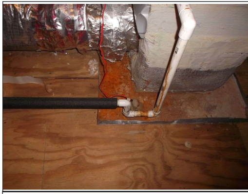
Major rust in furnace drain pan in attic
