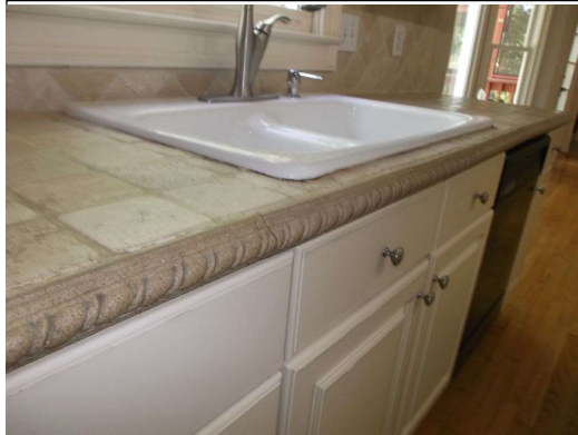
Missing bead of caulk at sink rim on tile
