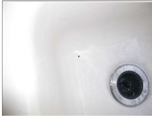
Hole in left sink bowl can rust through
