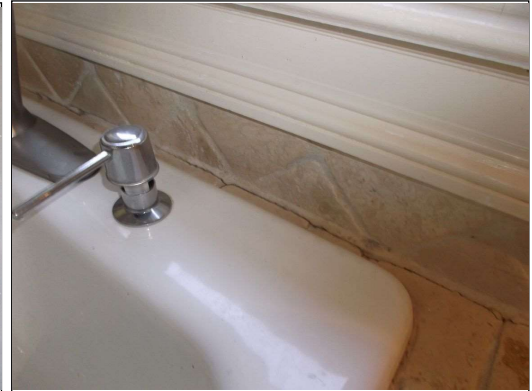
Cracks in grout at back splash
