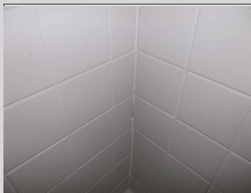
Missing caulk at shower corner
