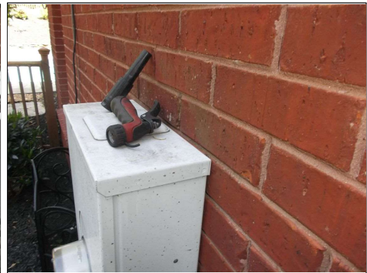
Missing bead of caulk across top of meter box
