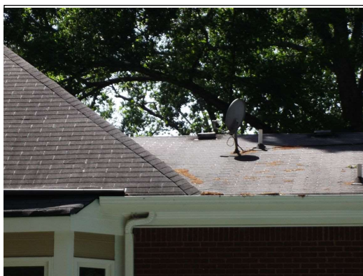
TV dish on roof/shingles show wear
