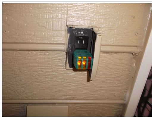
Screened porch outlet not GFCI unsafe
