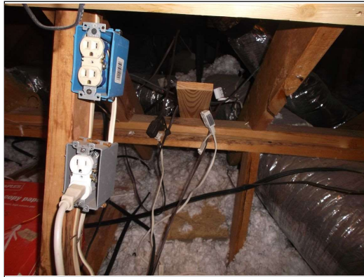
Drop cords for wiring in the attic
