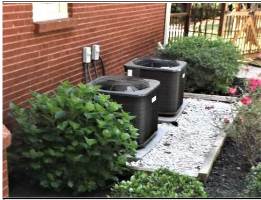
AC units aging
