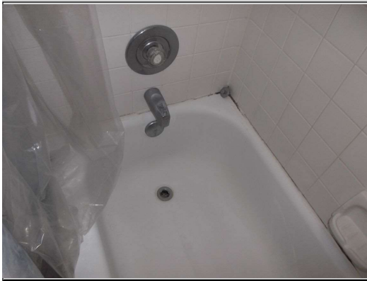
Stopper missing/mold on caulk
