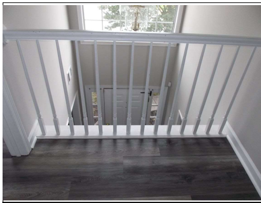
Guards spaced too wide at balcony
