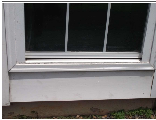
Bay window sash not square in frame
