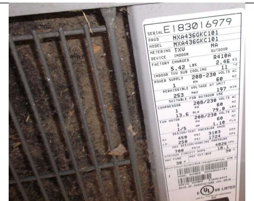
AC units fins need cleaning
