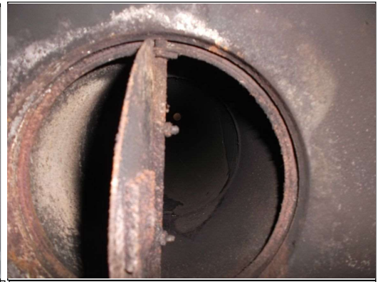
Creosote in chimney flue
