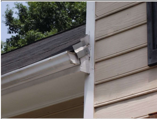
Rot and defective repair at soffit
