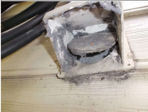
Dryer vent clogged and door stuck open
