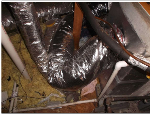
Air duct sharp turn
