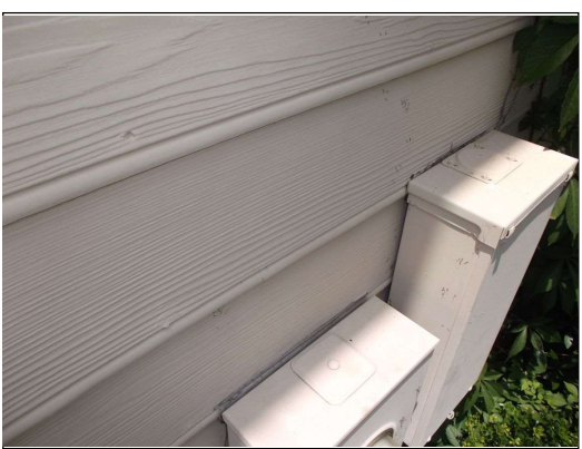
Missing caulk over electrical boxes
