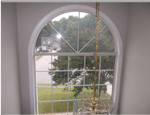
Arched window glass fogged
