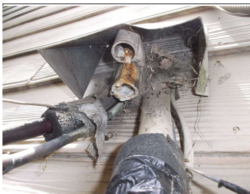
Condensate pipes drip at the wall
