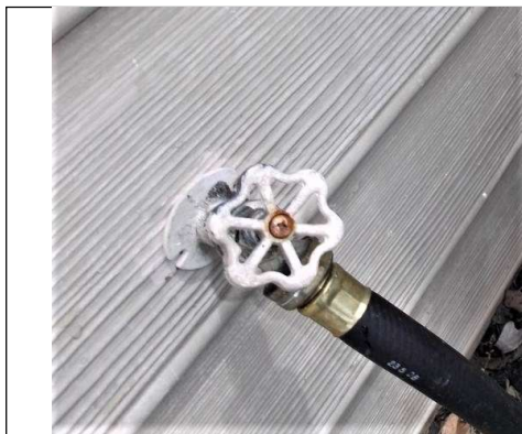
Missing anti siphon device at front faucet
