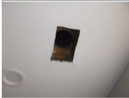
Missing vent register cover
