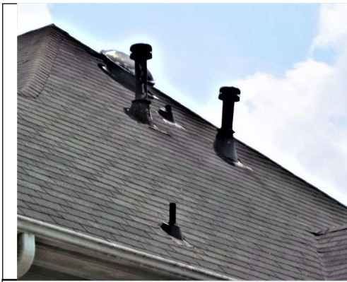
Pipe and vent flashing nailed on top shingles
