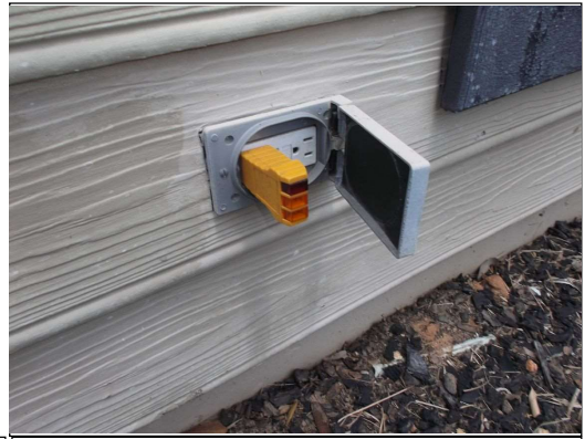
Rear outlet not energized and not reset able
