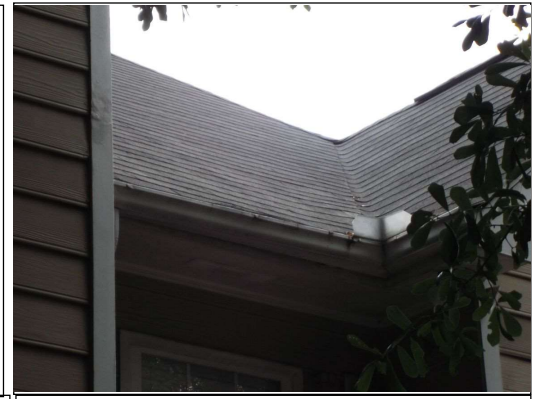
Slight dip in roof deck left of valley
