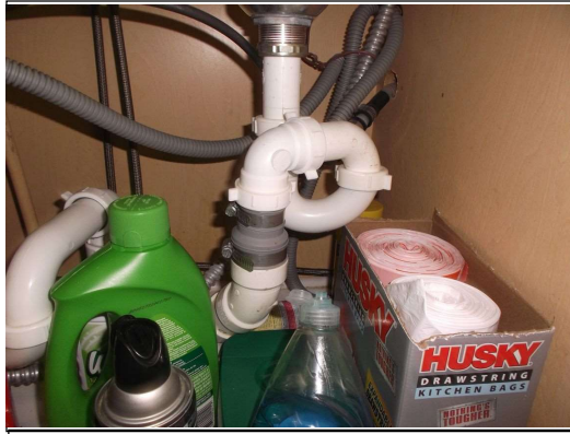
Drain pipe is a S-Trap
