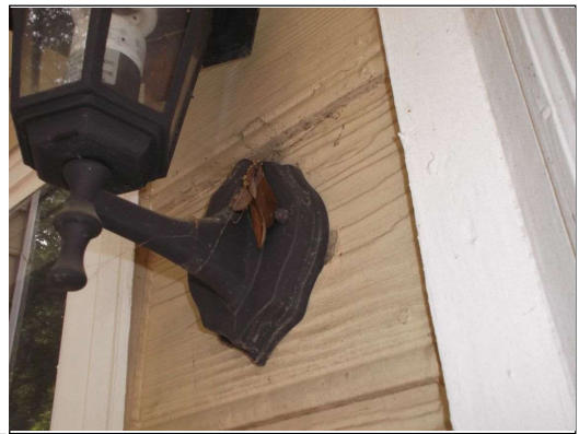
Missing caulk around light fixtures on siding
