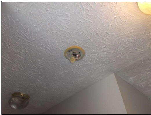
Missing smoke alarm
