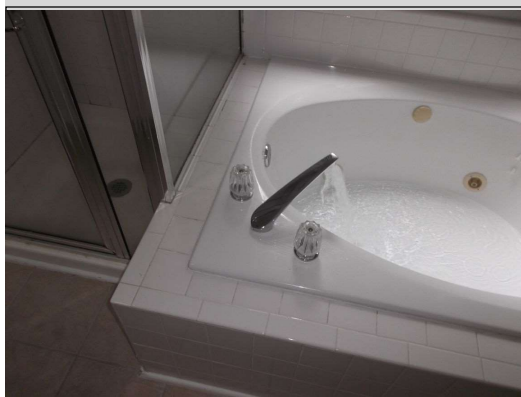
Tub spout loose, caps missing at knobs
