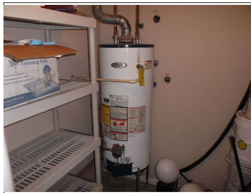
No expansion tank above water heater
