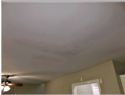
Dry stains in ceiling above bar stools
