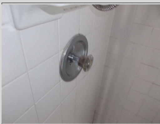
Shower knob missing cap
