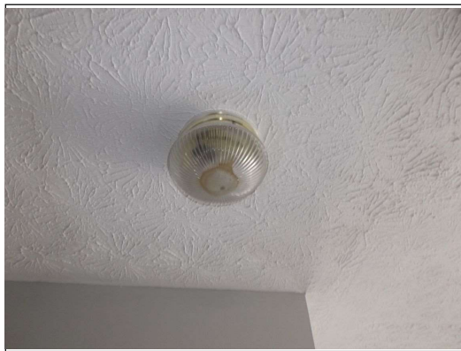
Water in 2nd floor hall light fixture
