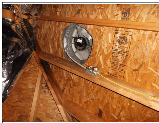
Exposed wires at attic fan junction box
