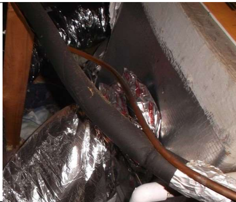
Air duct detaching from collar
