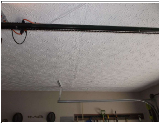
Defective ceiling repair at seam
