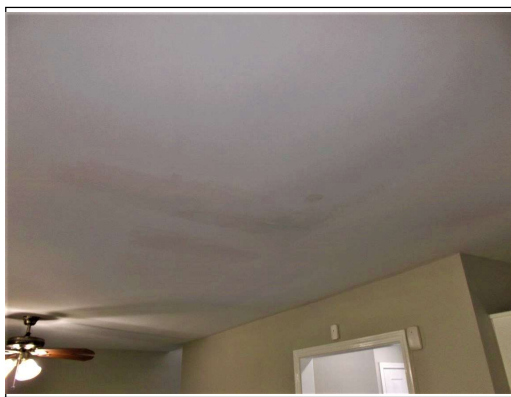
Dry stains in the ceiling over bar stools
