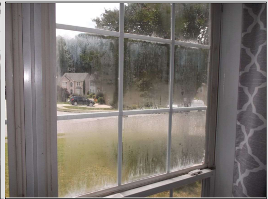
Glass fogged at the office
