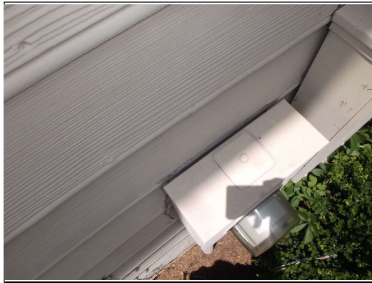
Meter box detaching from the wall/no caulk
