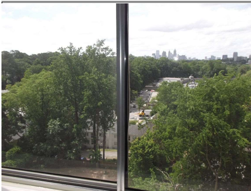
Glass weather strip detaching/window worn
