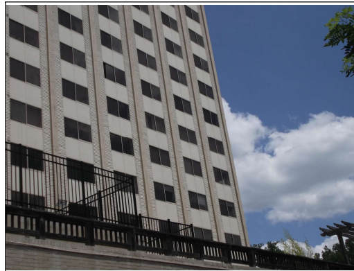
Screens missing and windows worn
