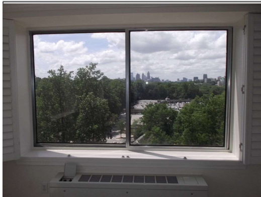
Window not opening
