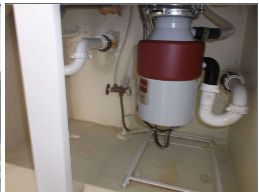
Sink cabinet has water damage painted over
