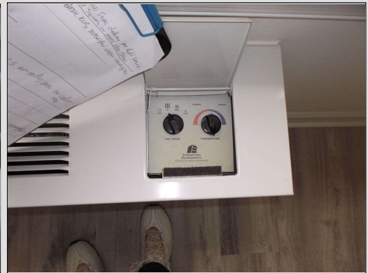
Poor cooling system in great room
