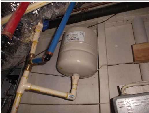
Expansion tank rest on the water pipe
