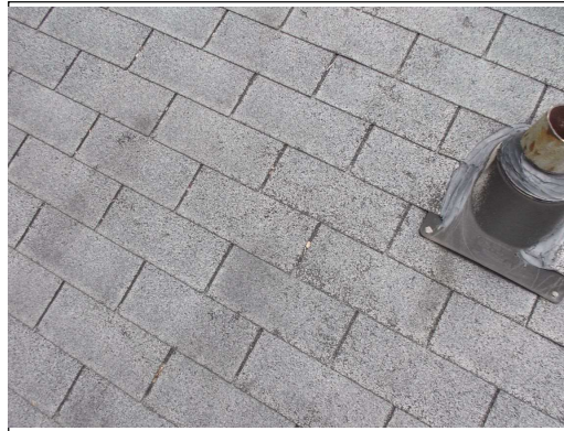
Shingles worn several areas
