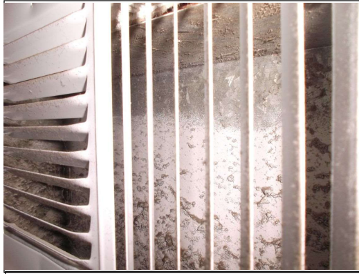
Dust in air ducts
