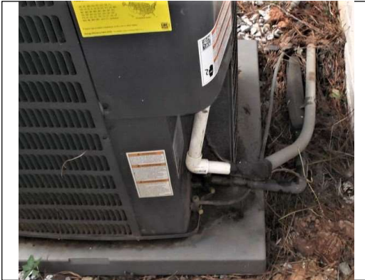
Water pipe for electrical conduit at AC
