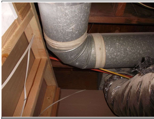
Asbestos tap wrapped on ducts
