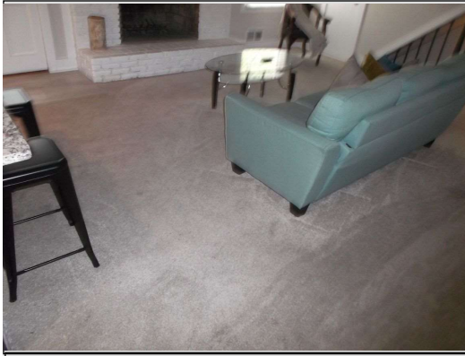
Floor sagging and carpet soiled
