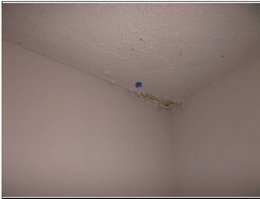
Water damage at laundry ceiling
