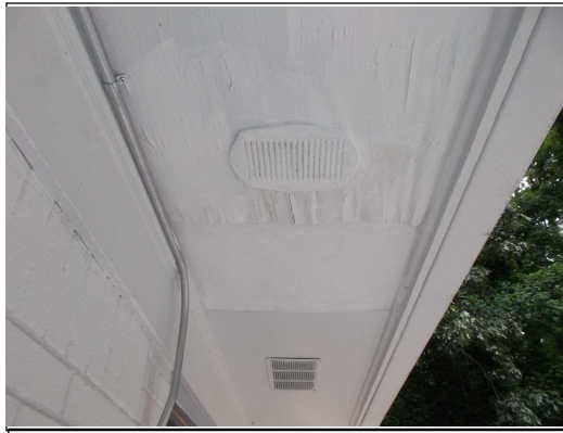
Water damage at soffit painted
