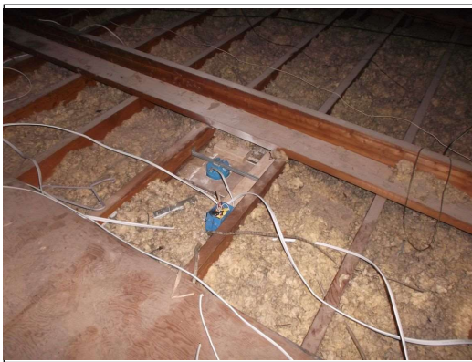
Exposed wires in attic several areas
