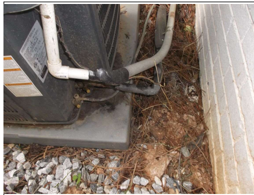
Refrigerant line insulation missing at AC
