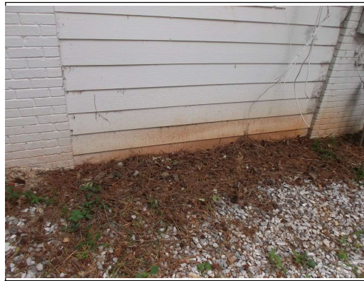
Siding touch ground right side of house
