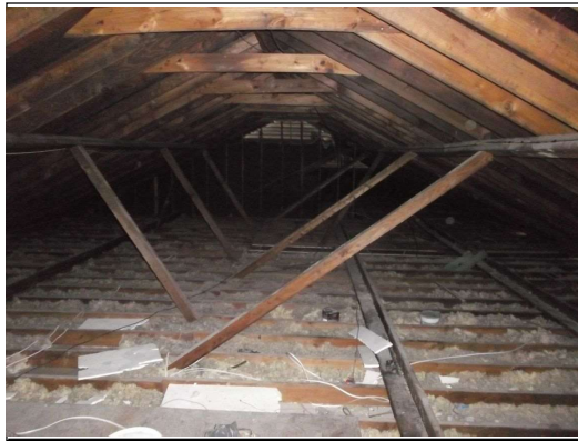
Debris in attic
