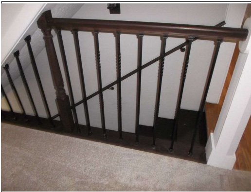
Guards spaced too wide
