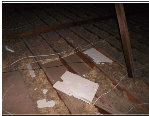
Missing and poor insulation coverage
