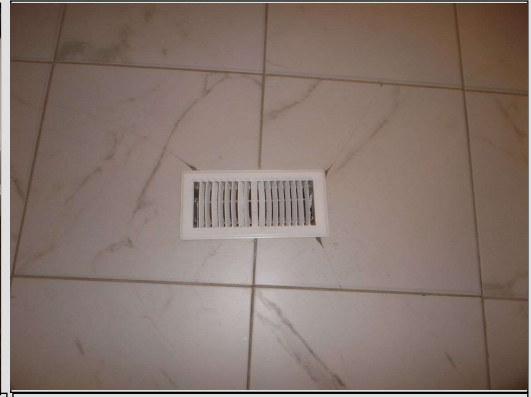
Cracks in master bath floor tile
