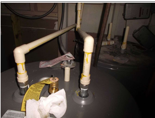
Water pipes not supported above water heater
