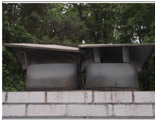
Chimney cap on left drain under right one
