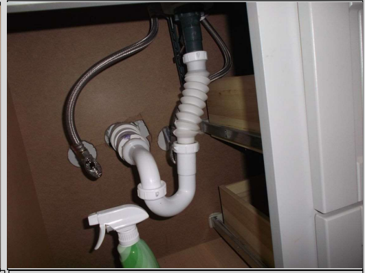
DIY drain pipe
