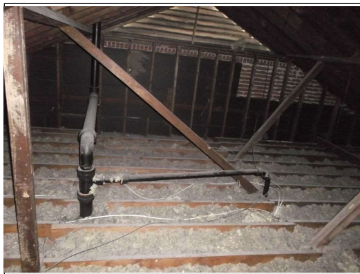
Poor insulation coverage
