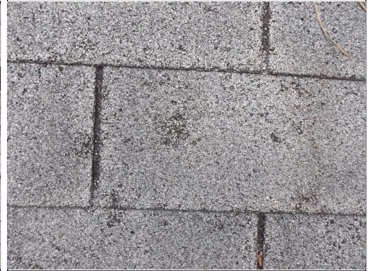
Nails pushing through shingles
