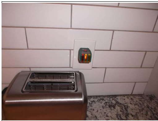
Outlets not grounded
