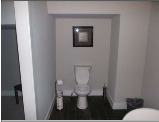
Low headroom over toilet
