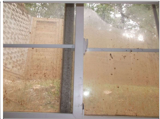
Window glass broken and wont close
