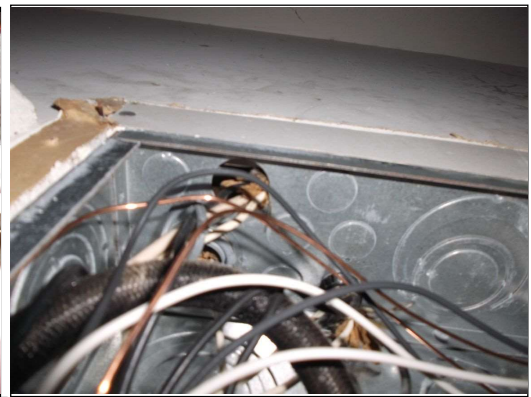
Wires enter panel hole contact sharp metal
