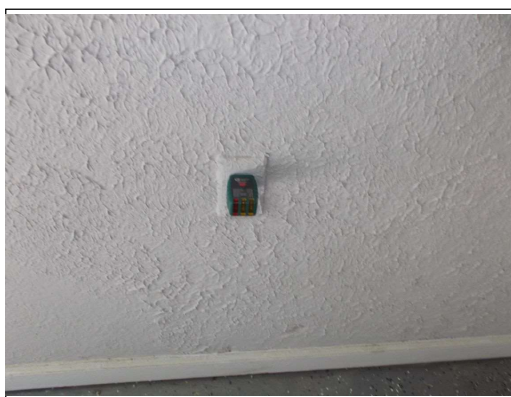
Garage outlet defective, not energized
