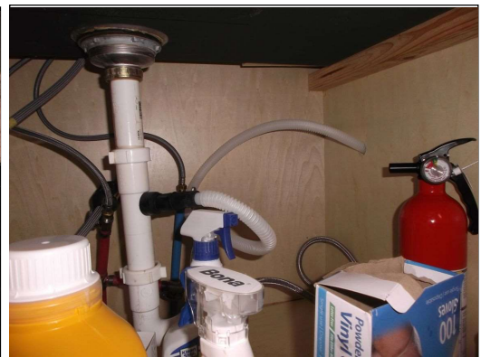
Dishwasher drain pipe not high looped
