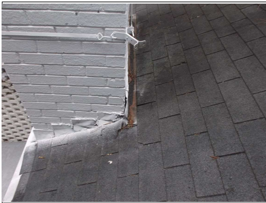
Flashing detaching at the back of chimney
