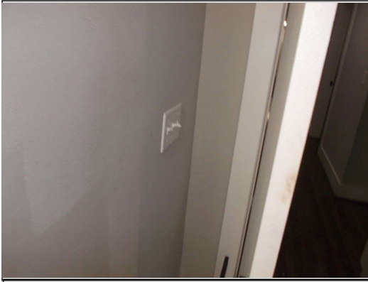
Light switches behind door
