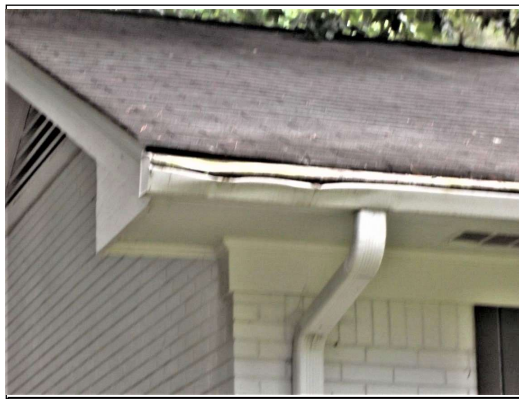
Garage gutter bent
