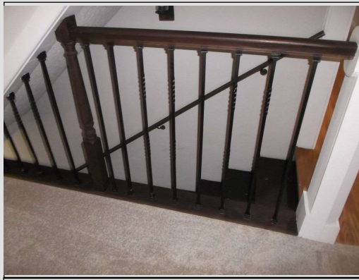
Great room stairwell guards space too wide
