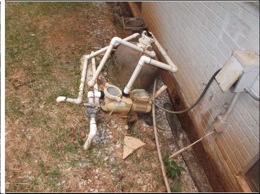
Pool equipment collapsing, stress on pipes
