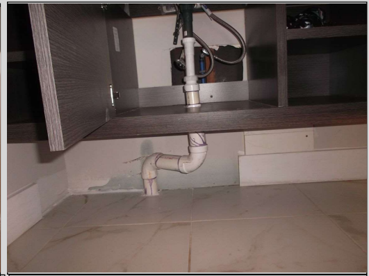
Improper drain pipe
