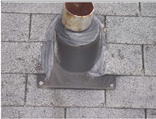
Flashing on top shingles face nailed
