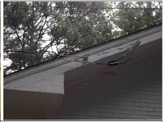
Service cables poorly anchored to fascia
