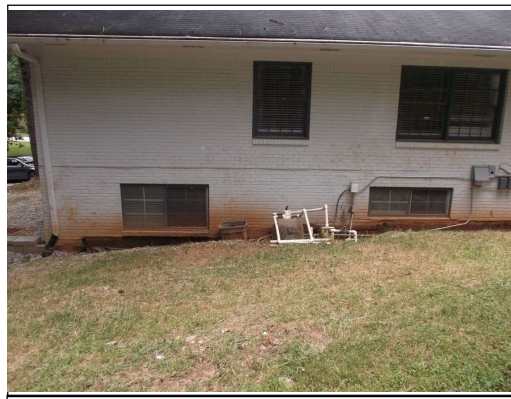
Mud on brick/gutter overflows
