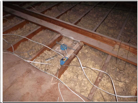
Exposed wire connections
