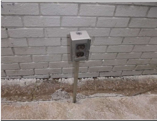
Defective receptacle at front porch
