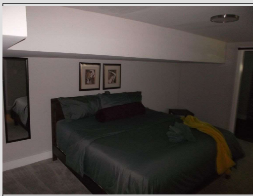
Basement bedroom ceiling too low over bed
