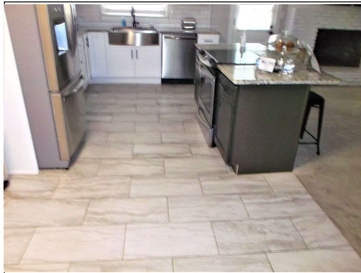
No exhaust fan above stove/ no light
