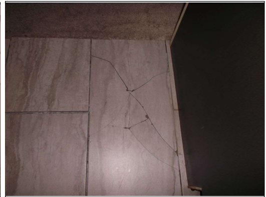
Floor tiles broken several areas
