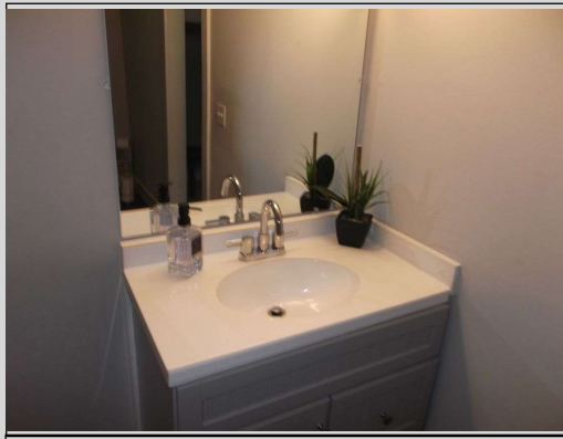
No outlet at sink
