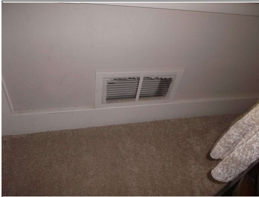
Air return grill at air register
