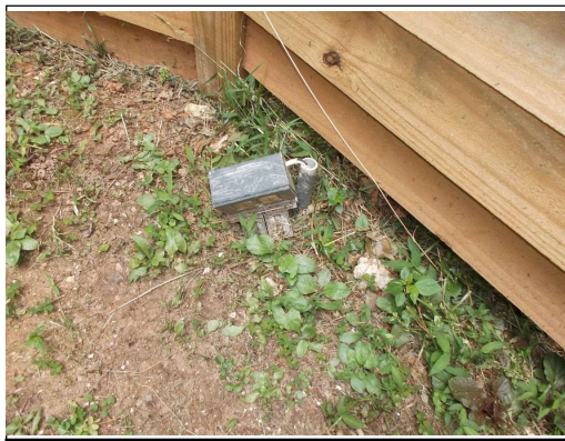
Pool side receptacle and box damaged
