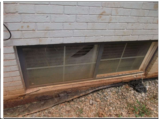
basement window broken not closing
