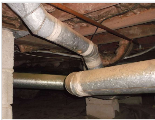
Asbestos like tape on old metal air ducts
