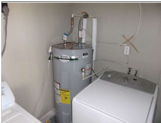
No expansion tank above water heater
