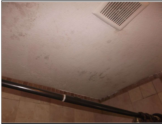
Ceiling sagging and mold at the hall bath
