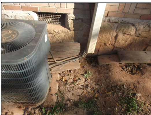
Refrigerant line insulation missing
