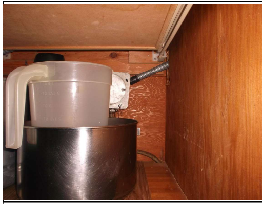
Missing bushing at conduit into box (tape)
