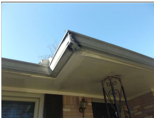
Water damage to fascia and plywood soffit
