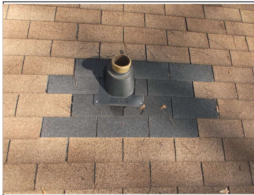
Flashing on top of shingles and face nailed
