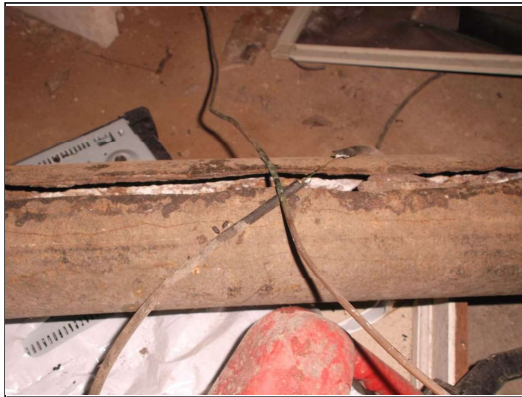
Split waste pipe in the crawlspace
