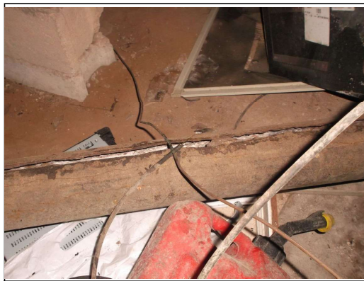
Split in waste pipe
