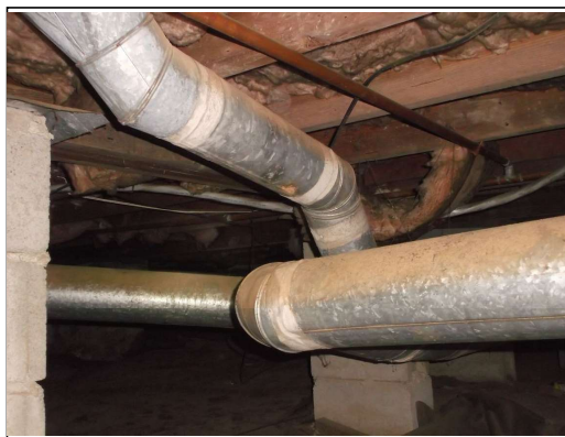
Asbestos tape on old metal air duct pipes
