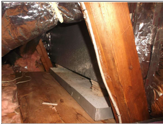
Furnace located in tight space attic access
