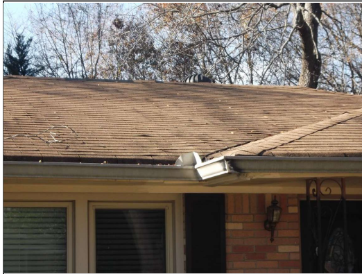
Defective shingles and roof decking at valley
