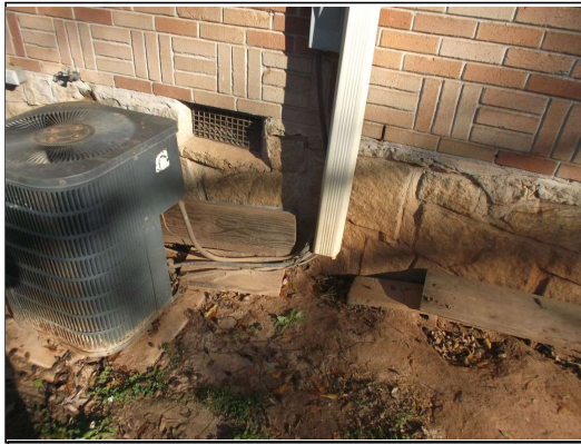
Refrigerant line insulation missing
