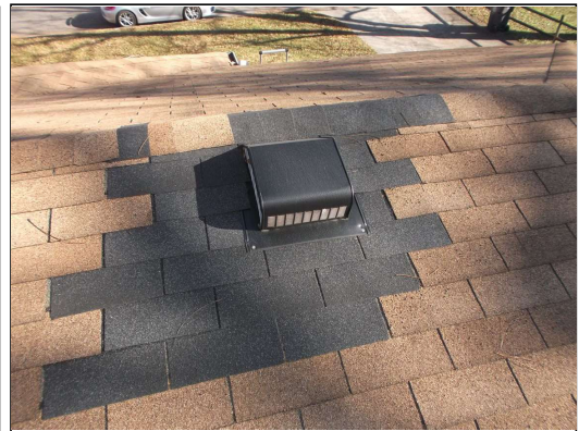
Wrong color shingles/flashing on top shingles
