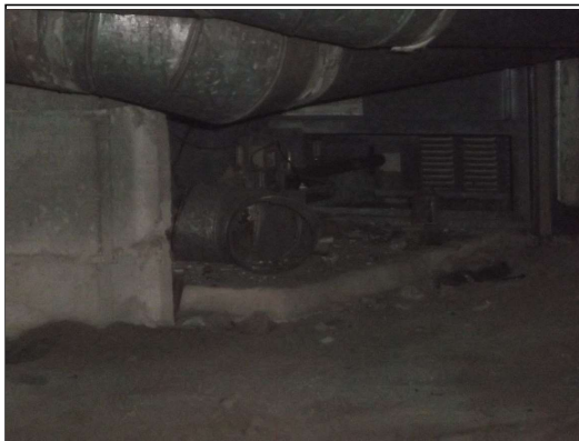
Old furnace still in crawlspace
