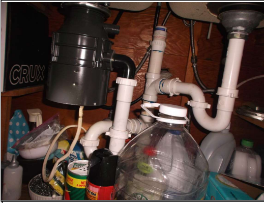
Improper electrical cable for disposal
