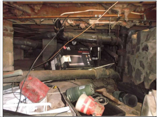
Unknown material wrapped around water pipe
