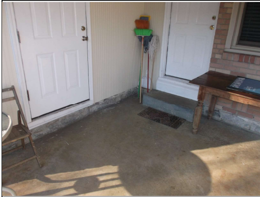
Steps up to doors too high at carport
