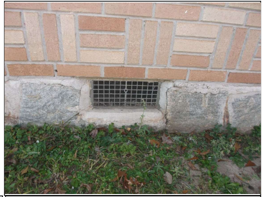
Foundation vents screen and doors missing
