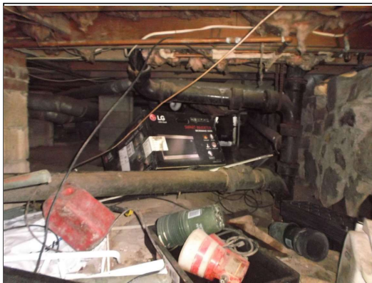
Belongs and debris in crawlspace
