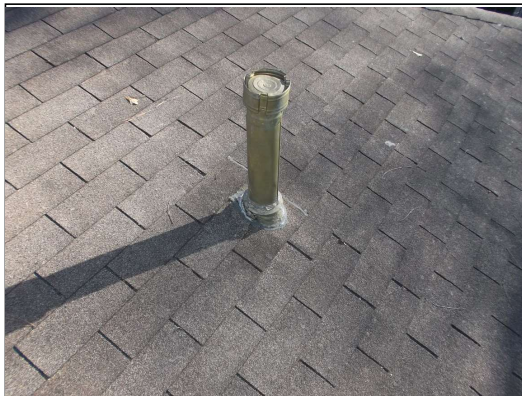
Shingles install all the way around pipe wrong
