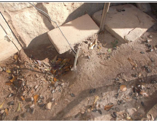
Ground wire poorly attached to ground rod
