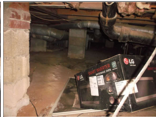
No plastic covering soil at areas in crawlspace
