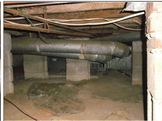
Damaged, loose, deteriorated Asbestos tape
