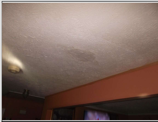
Defective ceiling repair at the living room
