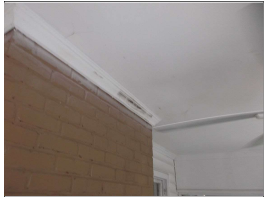
Mold on molding at porch may indicate leak
