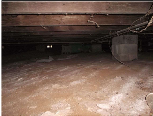
Missing moisture barrier
