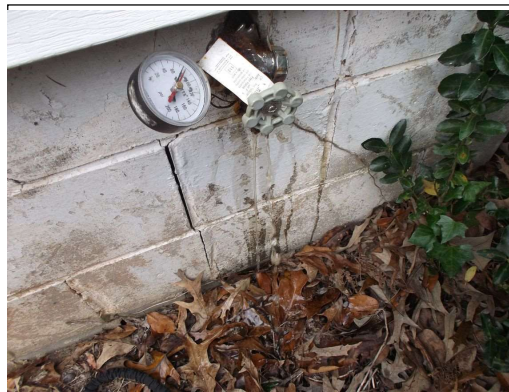
Verify hose faucets leaking at the handles
