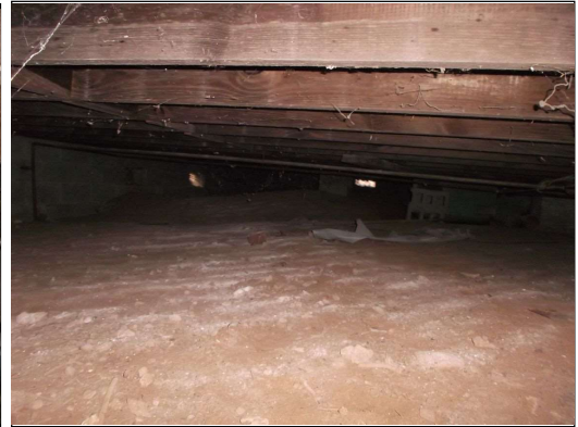
Missing moisture barrier
