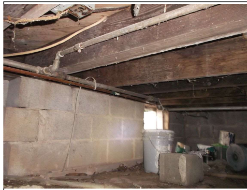
Slight fungus like substance on floor joists
