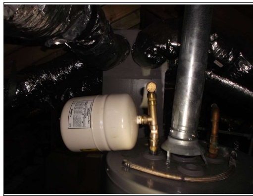
Expansion tank supported with water pipe
