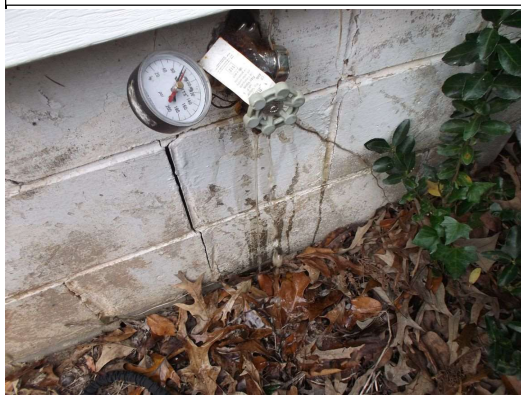
Slight cracks in foundation/faucet loose
