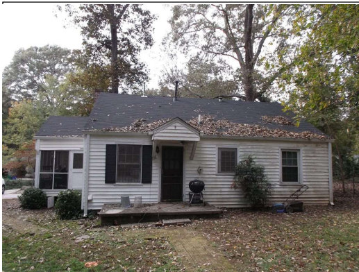
Siding needs wash & contact the ground
