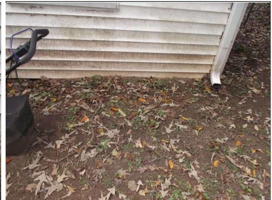
Siding in the soil, needs wash
