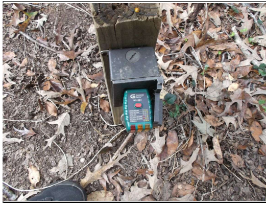
Yard outlet tested open ground/no GFCI
