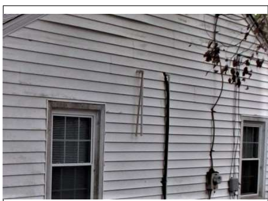
Condensate pipe not routed away
