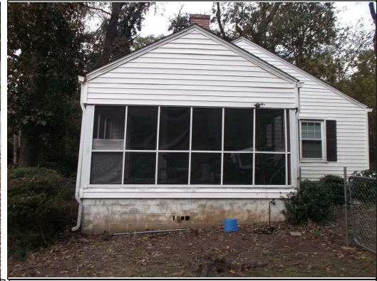
Screened porch framing leaning
