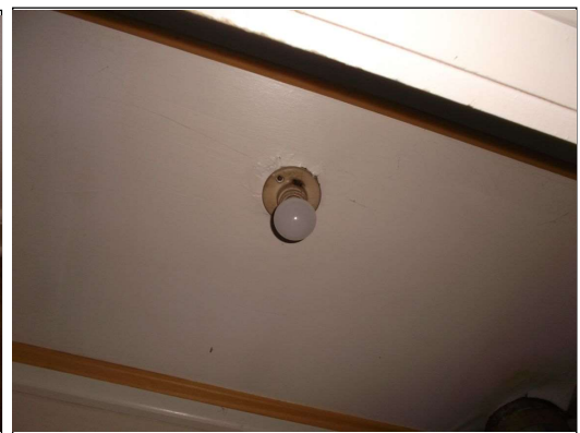
Exposed light bulbs in closets
