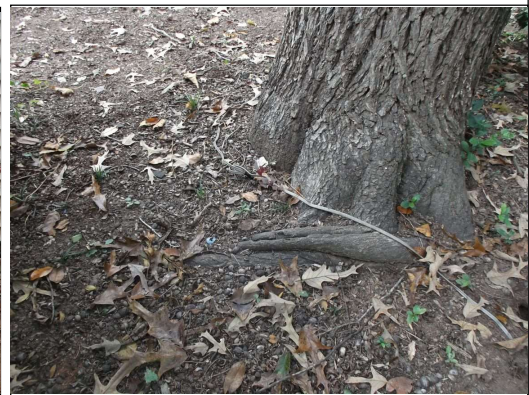
Electrical cable &amp; connections exposed
