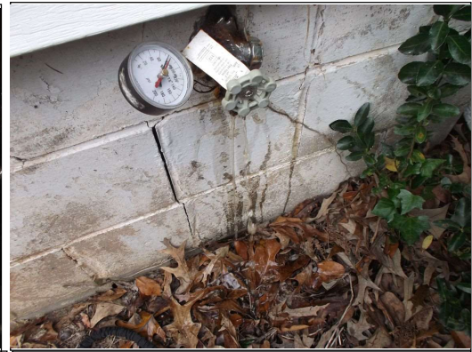
Verify if hose faucet leaks at the handle
