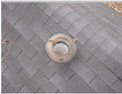
Missing rain cap on gas vent pipe
