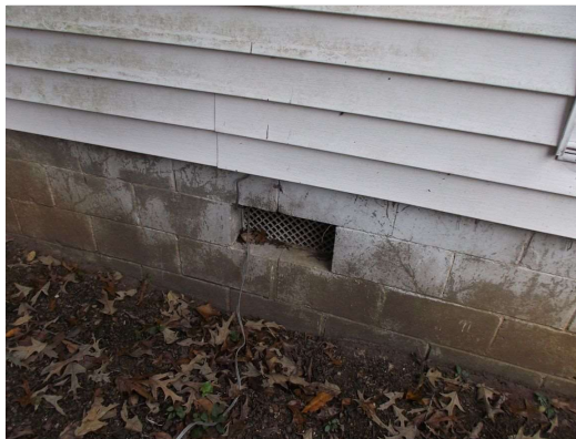
Defective foundation vents
