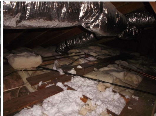
Water pipes in attic not wrapped in insulation
