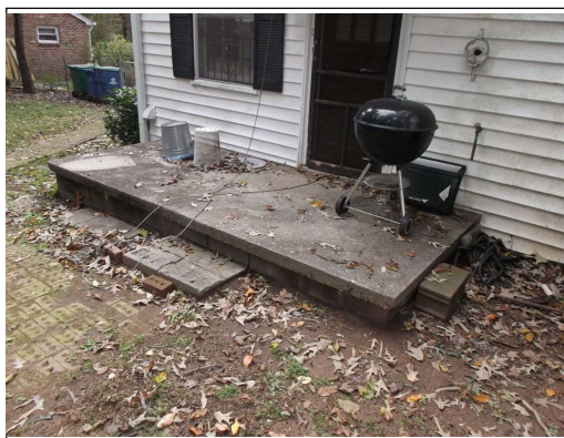
Rear patio has poor slope away from house
