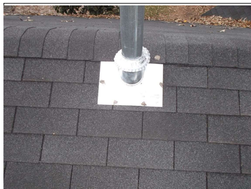
Flashing on top of shingles face nailed
