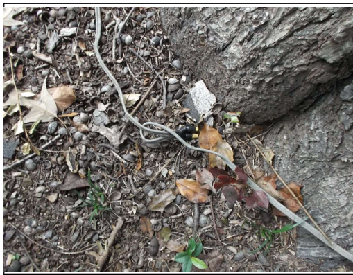
Exposed cable and wire connections
