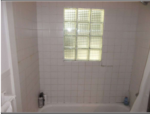
Wall defective and may have water damage
