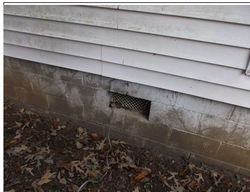
Foundation vents no screens and no doors
