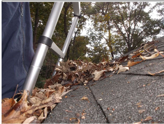
Shingles roll up near gutter
