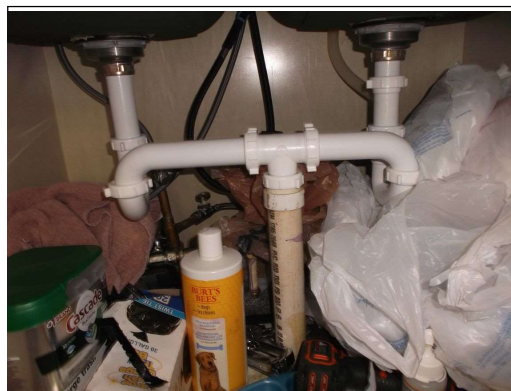
Improper and unsafe drain pipe system
