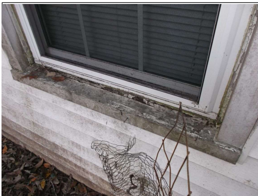
Rot a window seal at left side
