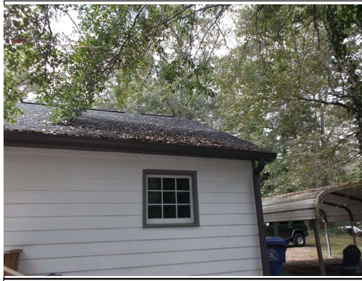
Debris on roof, tree limbs touch roof
