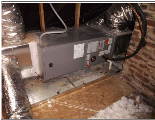
Furnace in attic
