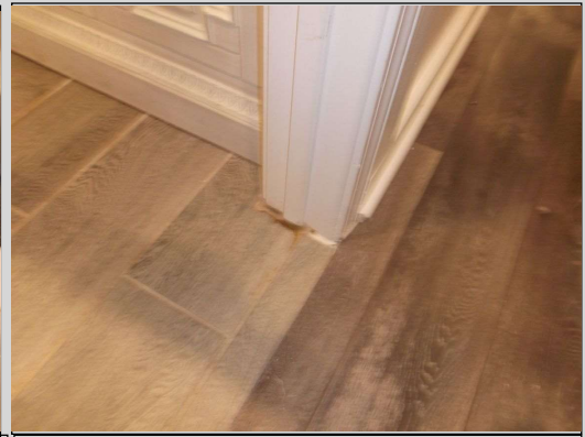
Large gap at door frame and floor
