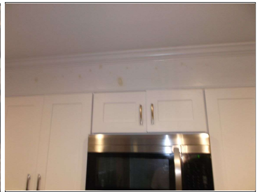
Defective paint above/doors bump
