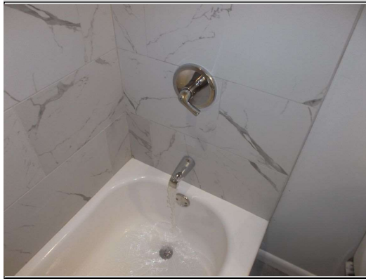
Tub spout and faucet handle loose
