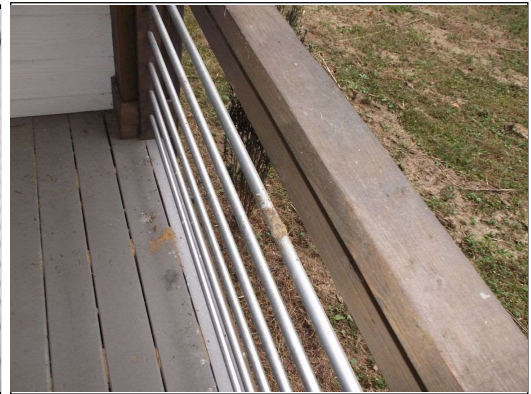
Bees drilling holes in the wood railing
