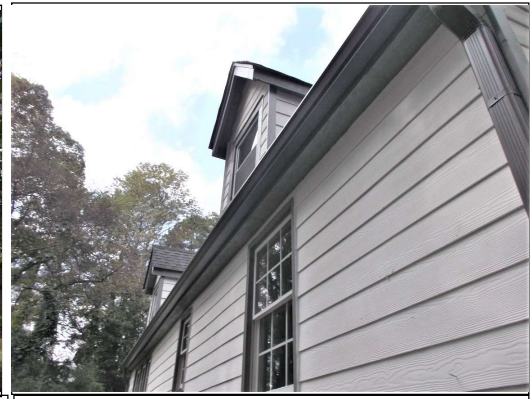
No vents installed at the soffit plywood
