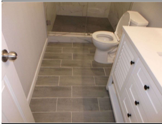
Floor settling near toilet
