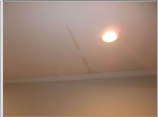
Water stains in den ceiling
