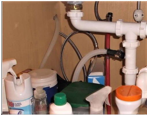
Dishwasher drain pipe not high looped
