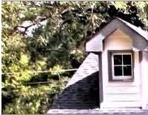
Electrical cables must head under soffit
