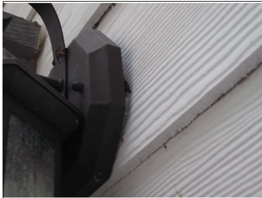
Missing caulk at fixtures on siding
