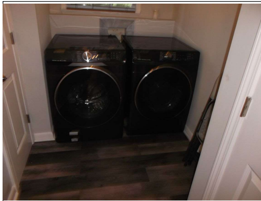
No washer drain pan installed with line
