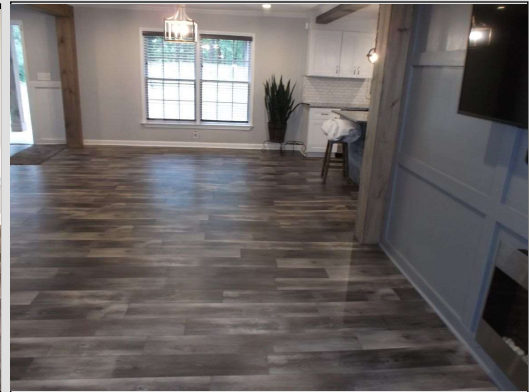
Floor sagging in the center of the room
