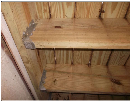
Wood deck missing flashing at house wall
