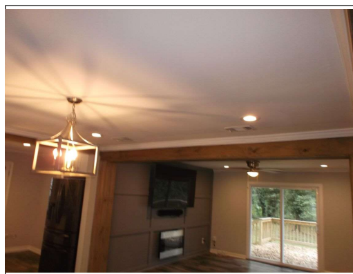
Air vents at center of room
