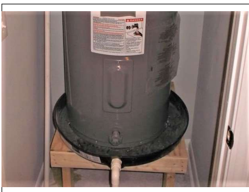
Water heater base poorly built can fail over time
