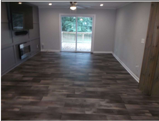
Floor sagging and settling toward S/L door
