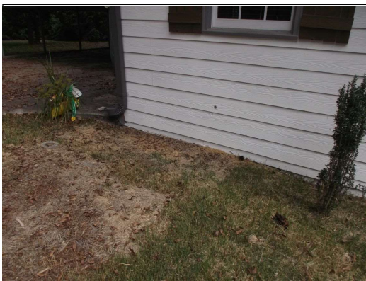
Siding in the soil
