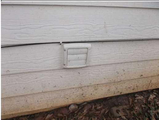
Improper dryer vent terminal (this is for bath)
