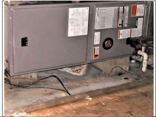
Corrosion in drain pan under furnace
