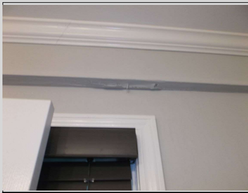
Paint peeling above window
