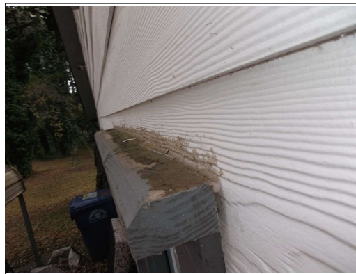
Cannot verify flashing over side door
