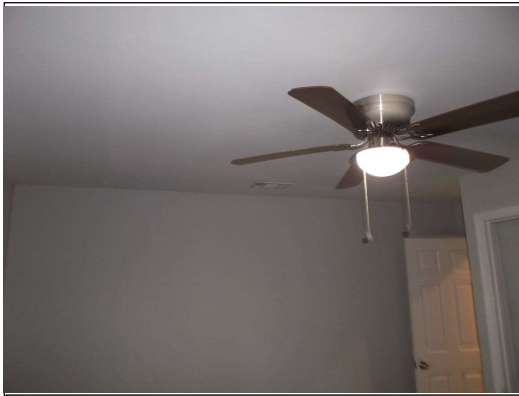
Air vent located near interior wall in bed
