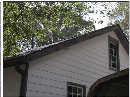
Fascia board is plywood and mold on wood
