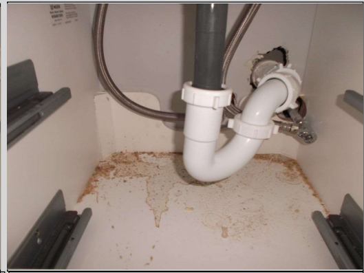
Dry stains on cabinet floor
