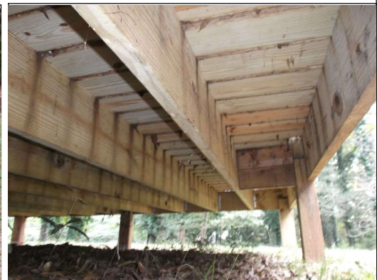
Deck posts are notched but not bolted to rim
