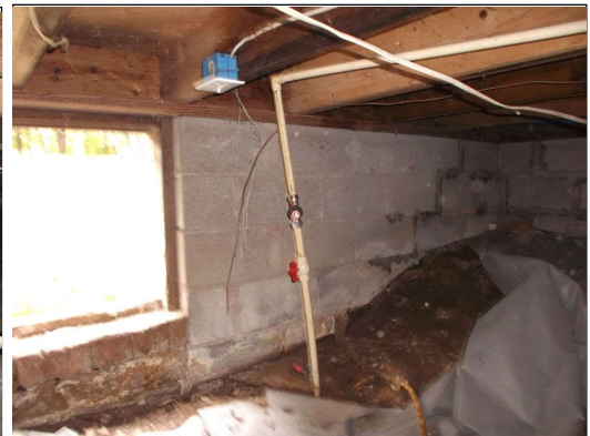
Exposed soil in crawlspace
