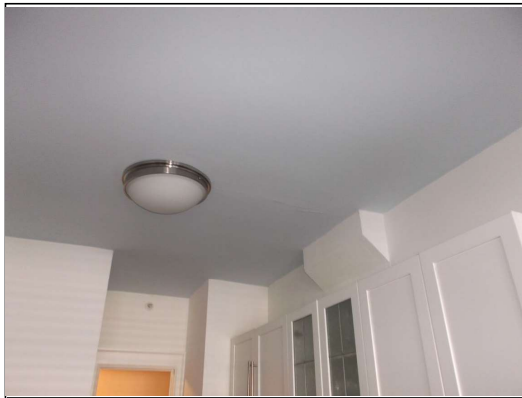
Peeling paint and sagging in kitchen ceiling
