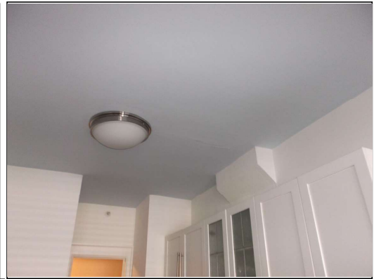
Light not operational
