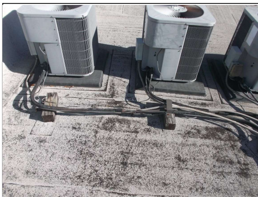
AC unit poorly marked/insulation deteriorate
