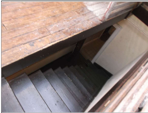
No handrails around attic stairwell & at stairs
