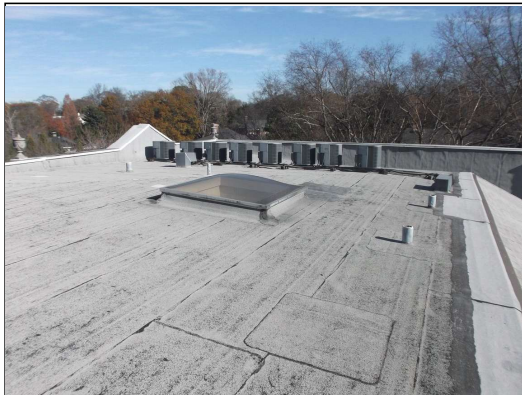
Roof covering worn
