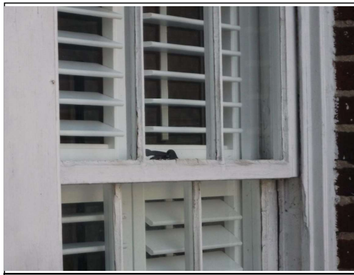
Deteriorating glass putty some window areas
