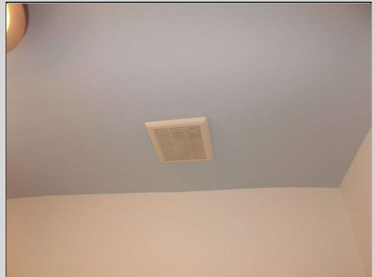
Exhaust fan vibrates and cover dusty
