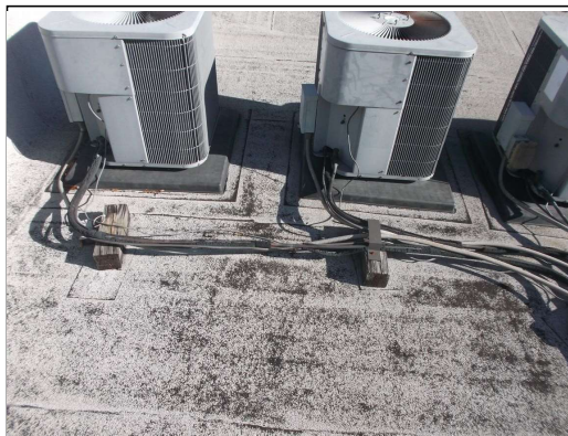
Roof covering deteriorating, asphalt showing
