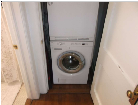
No washer drain pan & pipe to ext. installed
