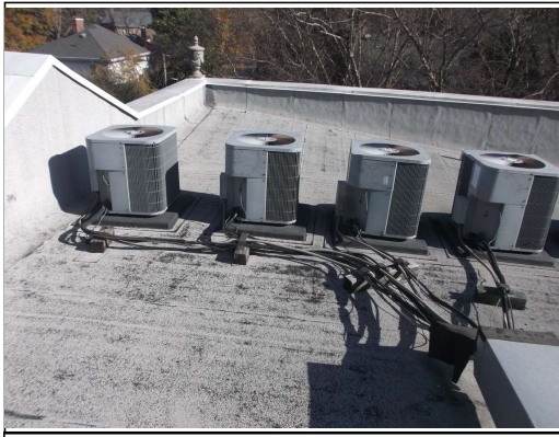
AC units appear not properly serviced
