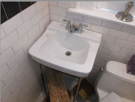
Sink stopper missing
