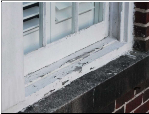
Deteriorating paint at windows
