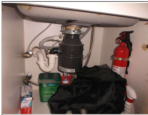
Disposal not operational
