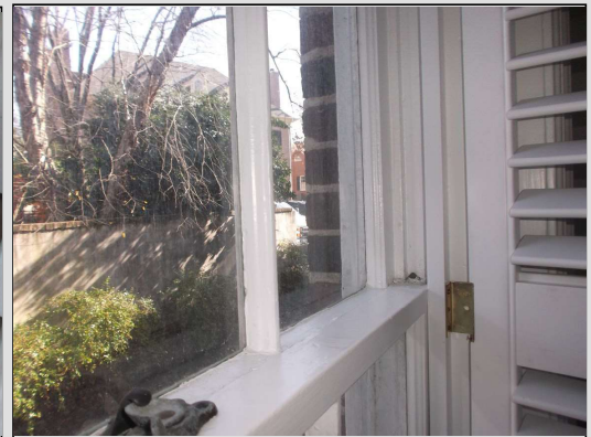
Bedroom windows painted shut, no sash cords
