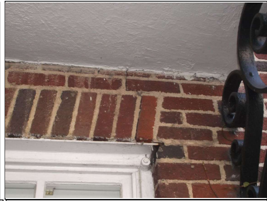
Small crack above right side of the patio door
