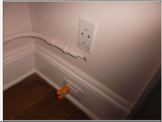
Exposed electrical cable at end of conduit
