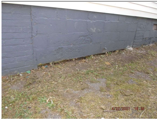
Defective foundation under walls
