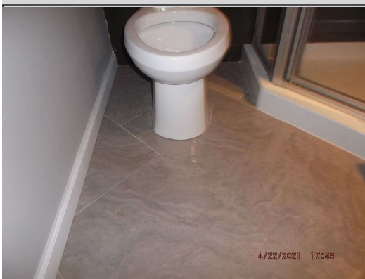
No caulk at toilet on the floor
