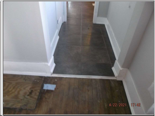
Kitchen floor higher is trip hazard
