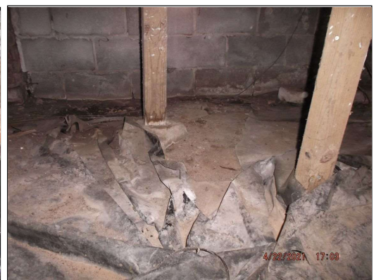
Defective moisture barrier
