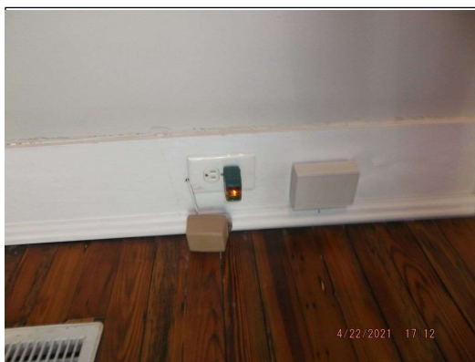
Outlet tested open ground at foyer
