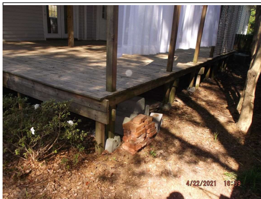
Deck unsafe and debris under deck
