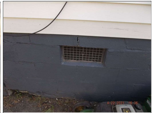
Defective foundation vents
