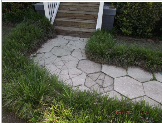
Walk stones broken
