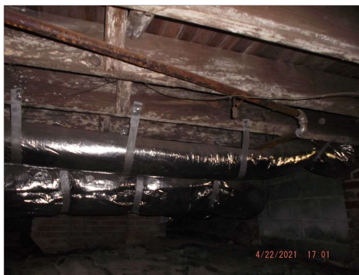
Mold and fungus
