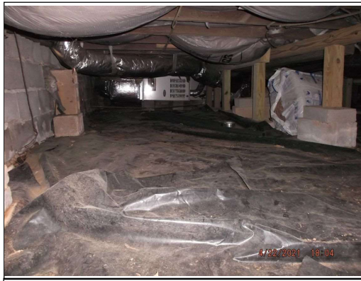
Furnace in crawlspace
