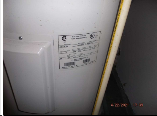
Cannot verify age of water heater
