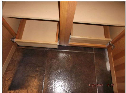
Defective drawer on left
