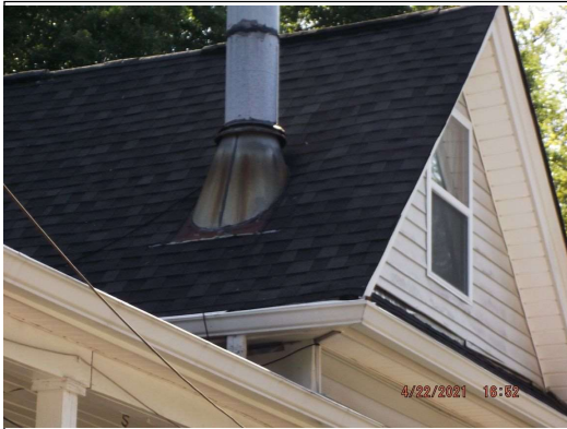
Chimney flashing nailed on top of shingles
