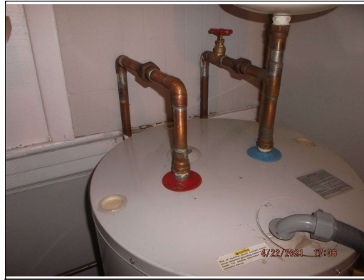
Copper/steel pipe join without dielectric fittin
