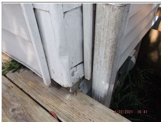
Possible Asbestos siding under vinyl
