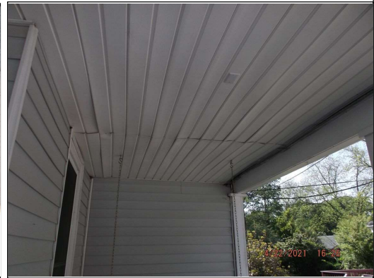
Front porch vinyl defective
