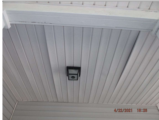
Front porch ceiling coming loose
