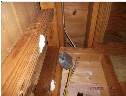
Open junction boxes
