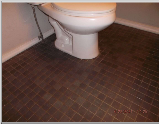
No caulk where toilet rest on the floor
