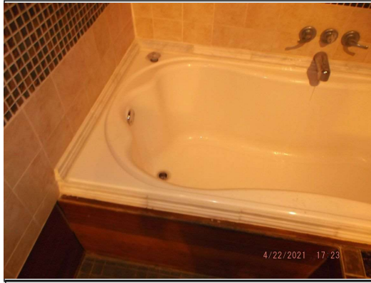
Tub stopper missing
