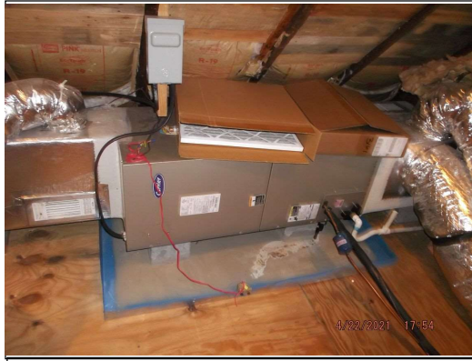
Furnace in attic
