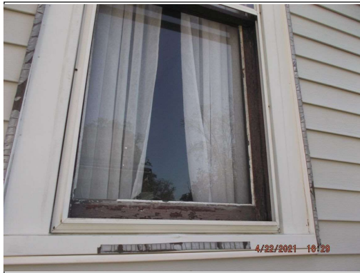
Wood windows need repair or replacements
