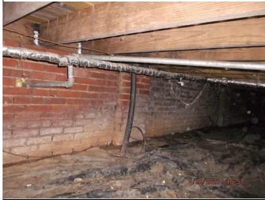
Water pipe used for gas pipe
