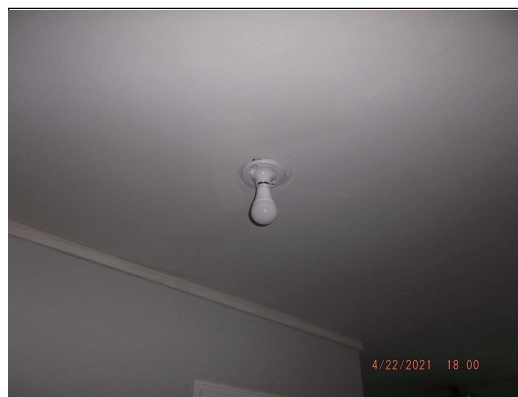
Utility fixtures for light fixtures at areas
