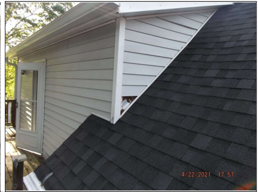
Missing siding panel at 2nd story wall
