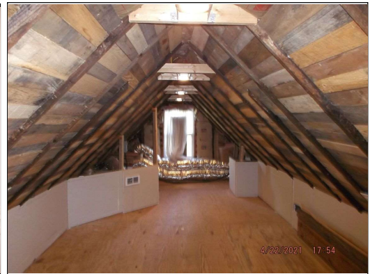
Roof framing sagging/ wrong size rafters
