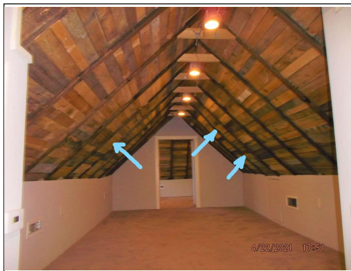
Roof framing sagging/ no braces
