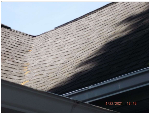
Roof system sagging
