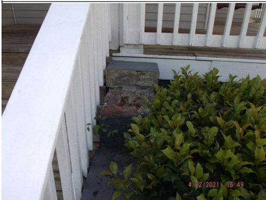
Broken pillar at the front stairs
