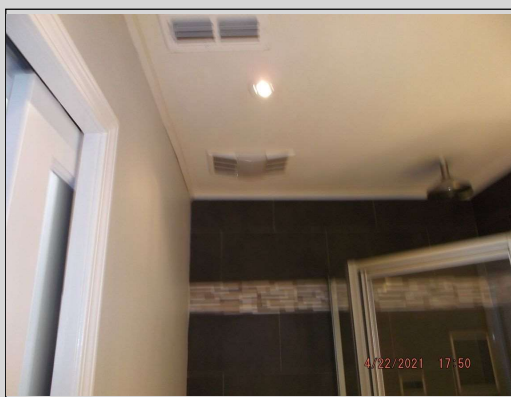
Exhaust fan mechanical noise when operating
