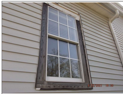
Missing cladding at window side of house
