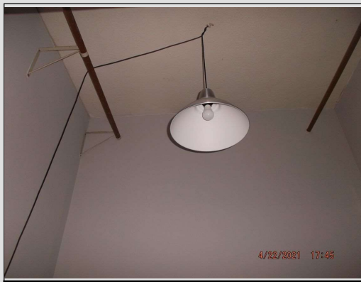
No light switch in bed closet
