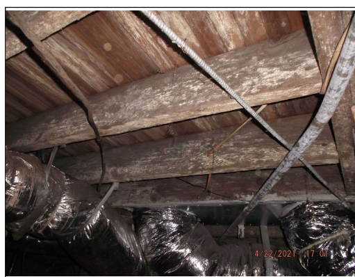
Mold and fungus
