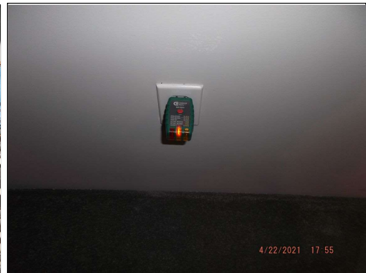
Outlet tested open ground rear room
