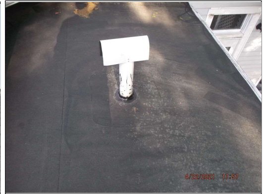
No flashing and boot around vent pipe
