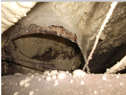
Possible Asbestos tape
