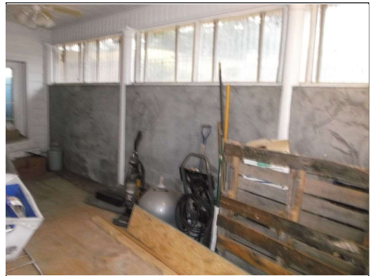
Posts contact concrete.
