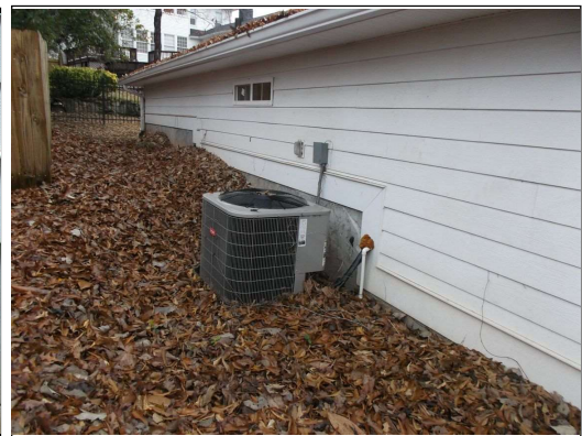
Condensate pipe under debris
