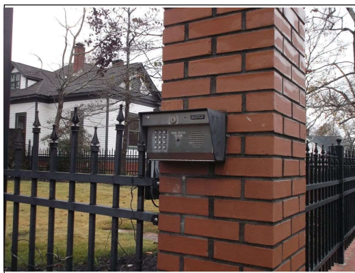
Verify gate and intercom control operate
