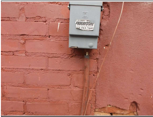
Conduit detached from AC box at house
