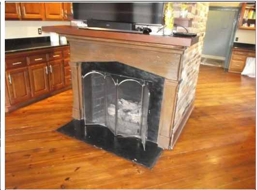
Fireplace damper open, mortar deteriorated
