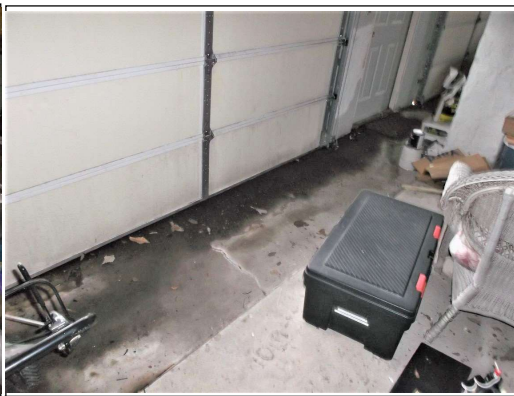
Floor wet at vehicle doors
