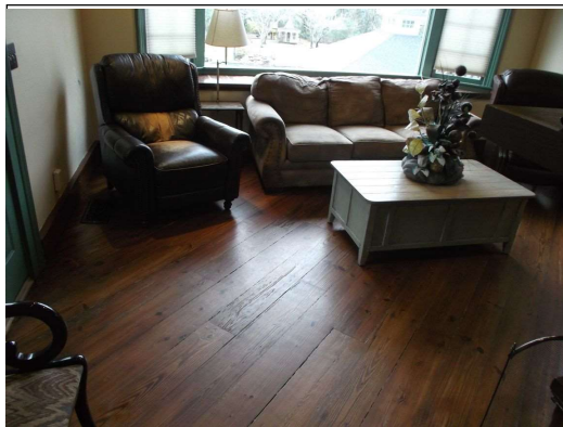
Floor major settling and sloping
