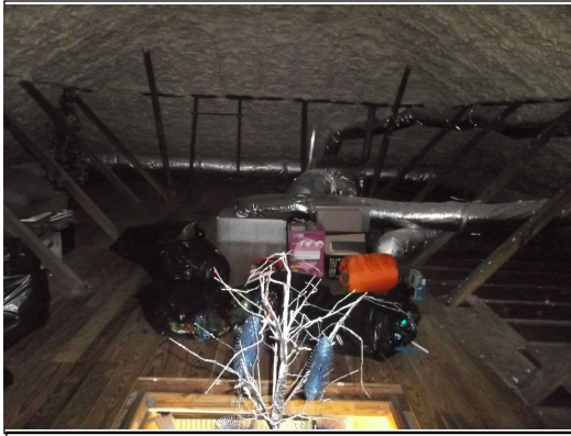
House attic encapsulated with foam insulation
