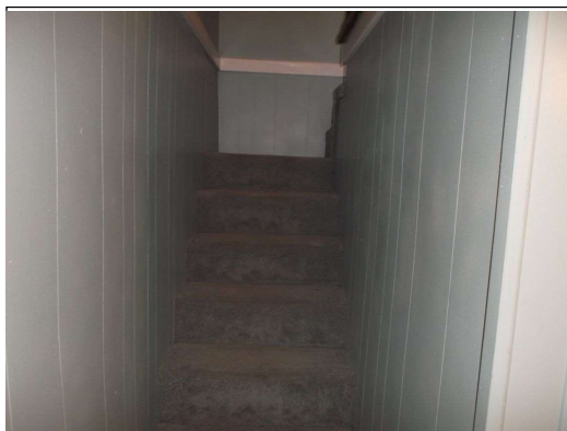
No handrail at basement stairs
