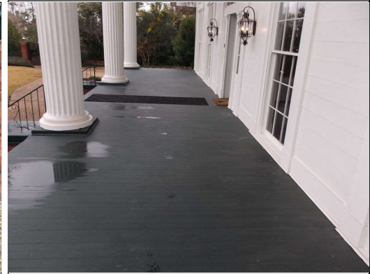
Porch floor has poor slope away
