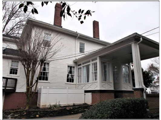
Defective paint some areas
