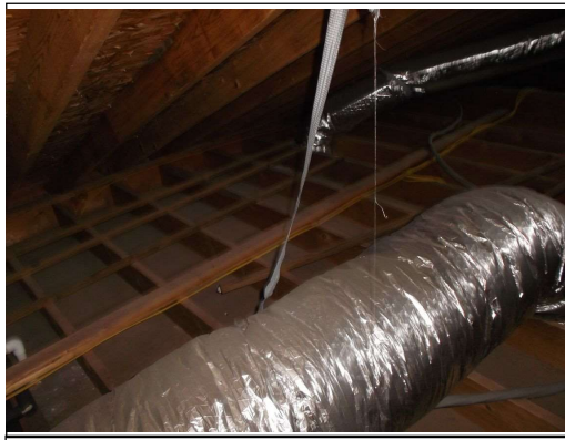
Missing insulation in detached garage attic
