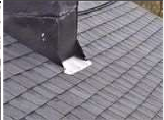
Flashing on top shingles face nailed
