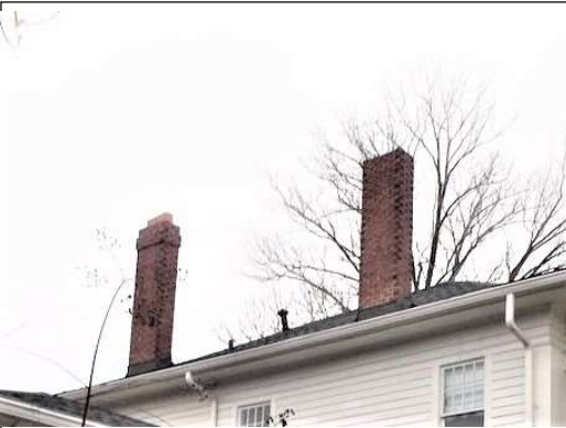
Chimneys missing caps & spark screens
