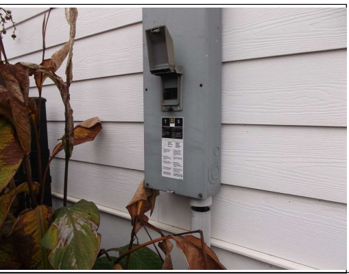
Conduit detached under disconnect panel
