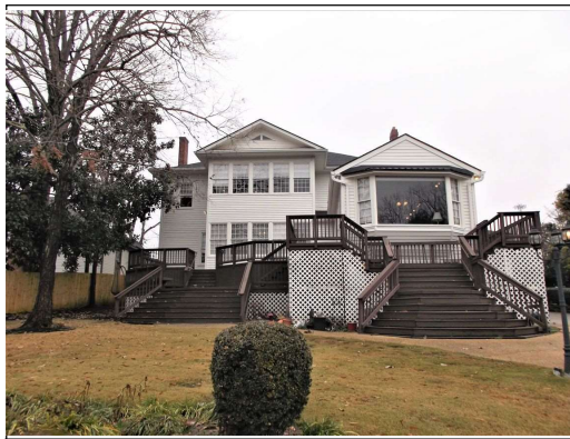
Rear room of kitchen appears to lean
