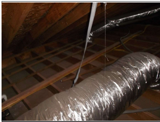
No ceiling insulation
