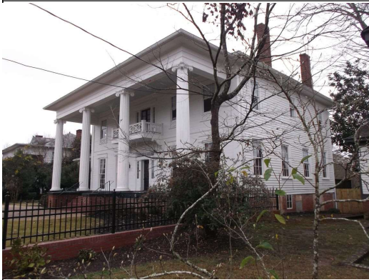
Tree stump/upper porch unsafe
