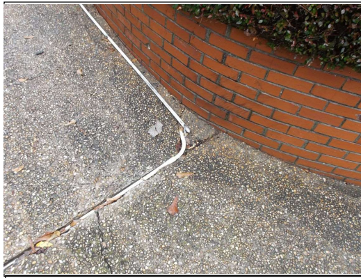
Conduit broken, exposed cable
