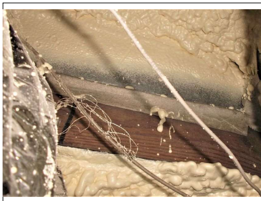
Possible Asbestos tape
