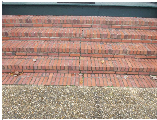
Crack in front steps/step high at porch
