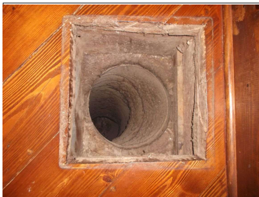
Air ducts very dirty
