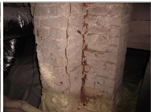
Cracks in brick columns
