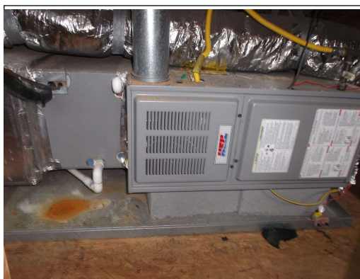
Wrong pipe in furnace, wire in hole, rust in pai
