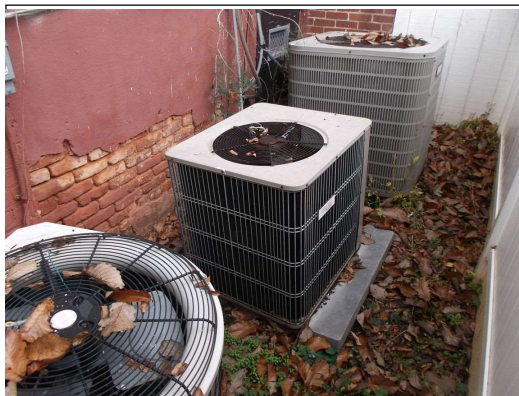
AC units closed in leaning on pads
