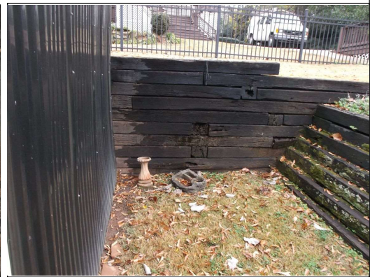
Soil slopes towards pool house floor
