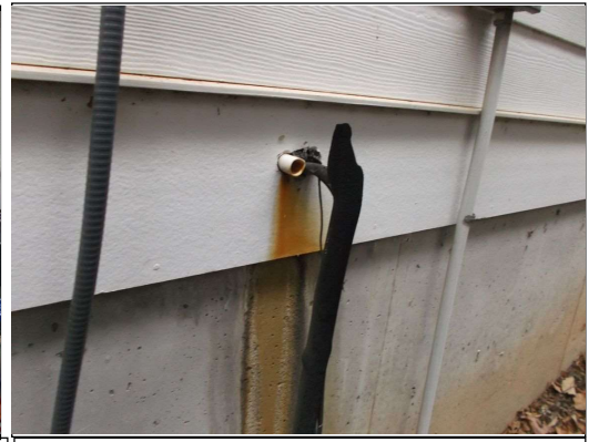
Condensate drain pipe improper
