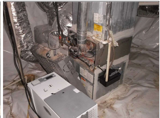
Basement furnace defective
