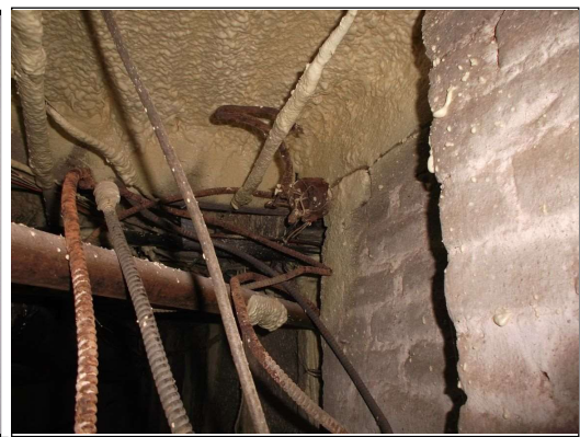
Exposed wire connections in crawlspace?
