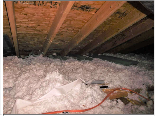
Baffles falling down at the pool house attic
