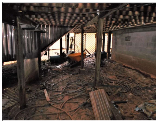
Wood in the soil/improper flashing at house
