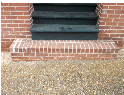
Carport step too high is trip hazard
