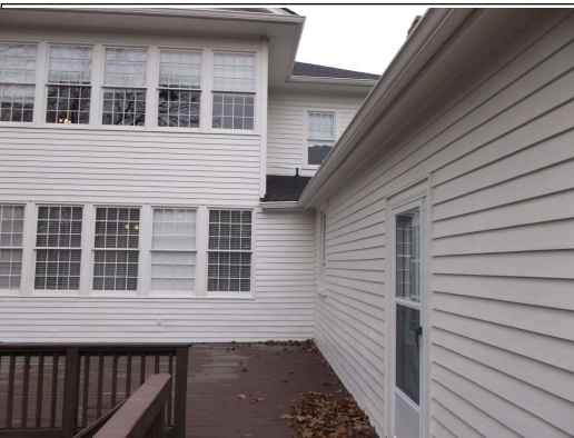
Gutter slopes away and leaking at joint
