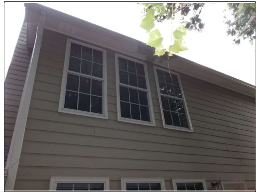
Missing screens at the rear windows
