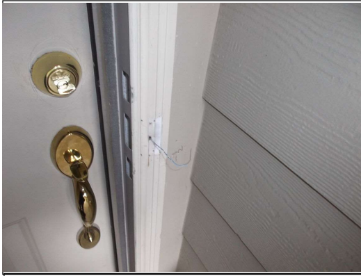
Doorbell button missing
