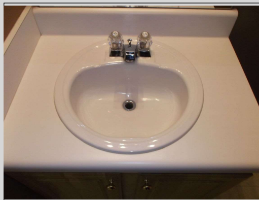
Sink stopper missing
