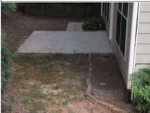
Poor soil away from the foundation
