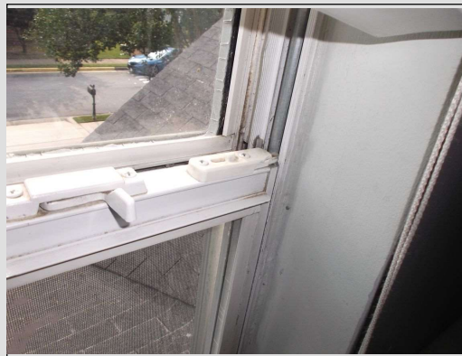
Cracked tilt out latch plastic
