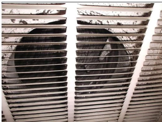
Air ducts dusty
