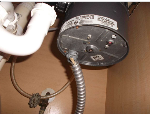
Detached conduit under disposal
