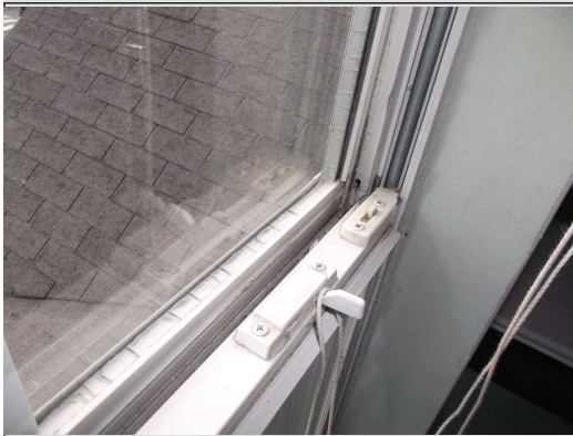
Top glass pushed out of frame
