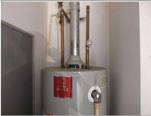
No expansion tank above water heater
