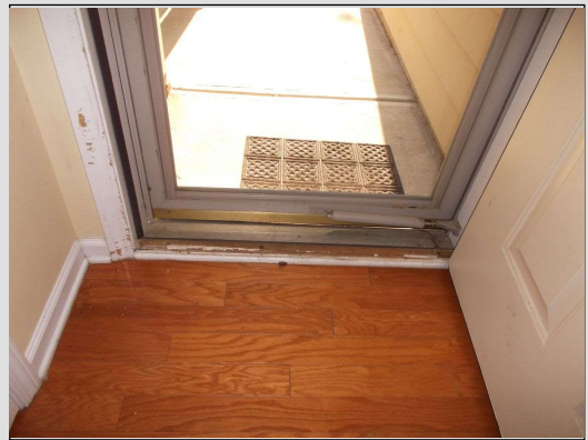
Daylight at the bottom of the storm door
