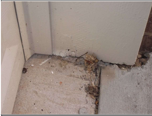
Water damage at the vehicle door frame
