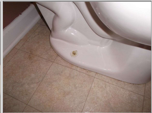
Missing screw and missing caulk at toilet
