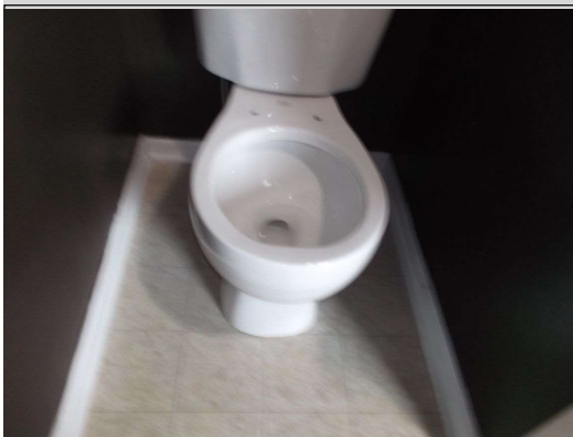
No toilet seat
