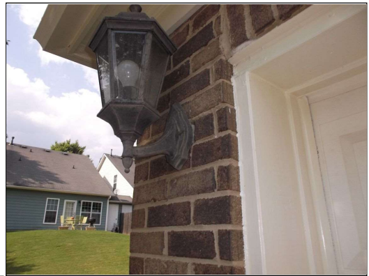
Missing bead of caulk around light on walls
