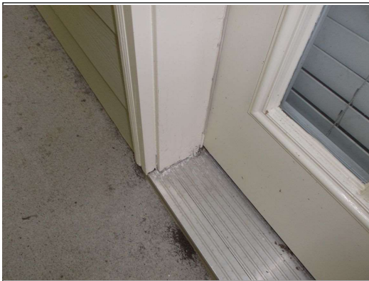
Water damage to rear door frame
