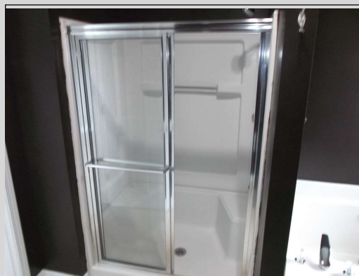
Shower cross bar too low
