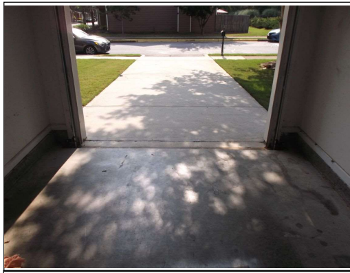
Door not letting up and down properly
