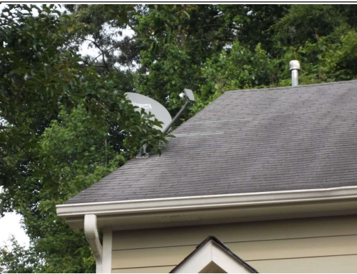
TV dish bolted to roof can cause leaks
