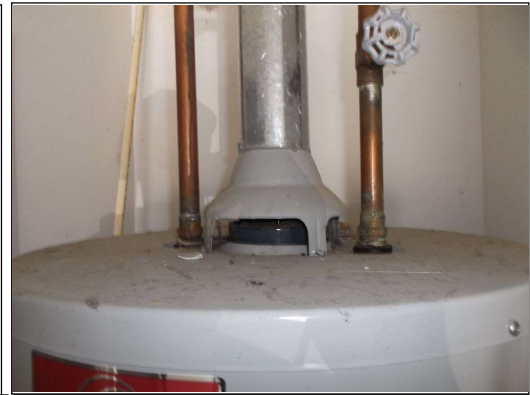
Copper &amp; steel join without dielectric fittings
