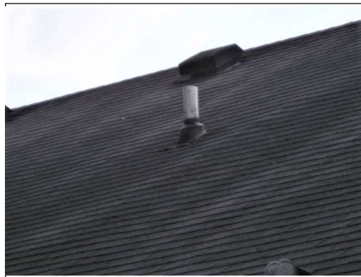
Plastic pipe flashing on top shingles face nailed
