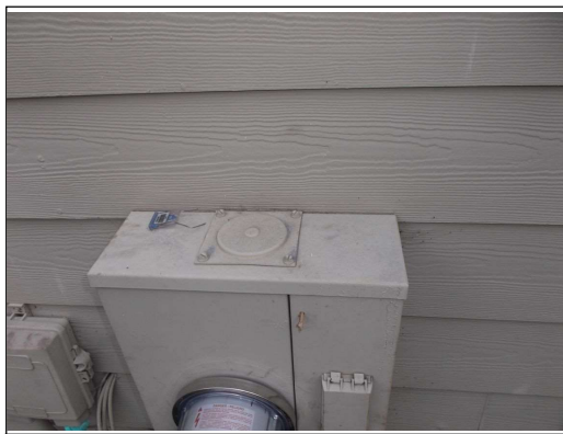
Missing bead of caulk over electrical boxes
