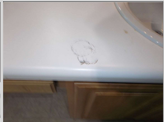
Stains or damage to counter
