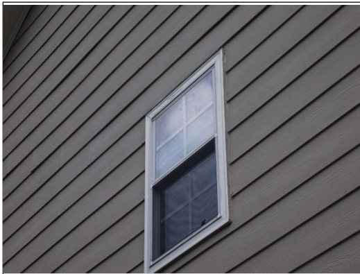
Window fogged at the left side of house
