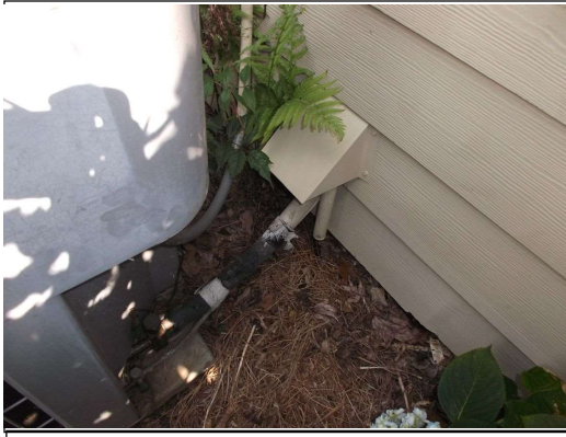
Condensate drain pipe drips at foundation
