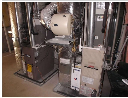
Utility room furnaces one older model
