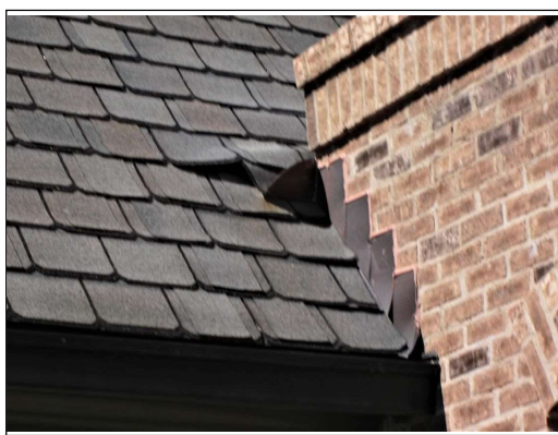
Roof-to-wall flashing lifting at rear of house
