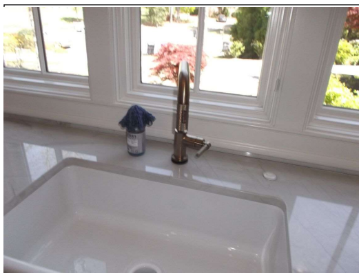
Sink faucet loose at the base
