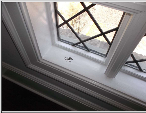
Window seal dry rot, water damage, termite?
