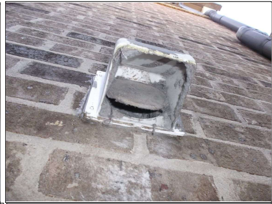
Dryer terminal door stuck open &amp; lint debris
