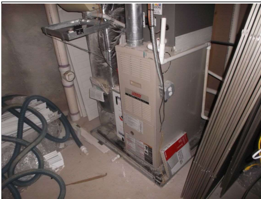
Other utility room furnace older model
