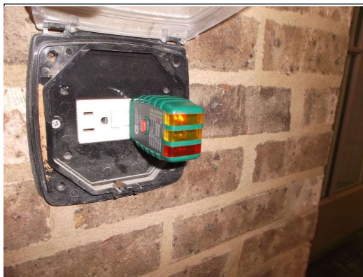
Lower patio ext. outlet tested open ground
