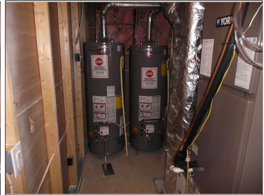
Utility room furnace
