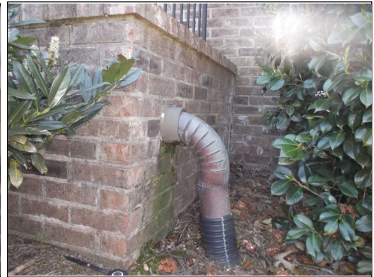
Drain pipe leak at side of front patio
