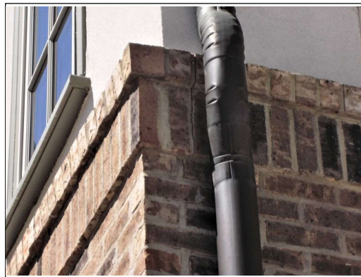
Movement crack at brick at rear brick corner
