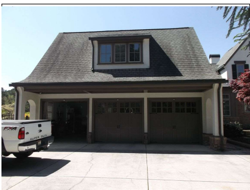
Gutter sagging over vehicle doors
