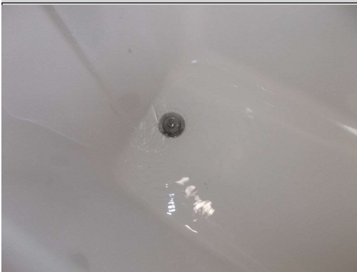
Tub drain outlet has corrosion
