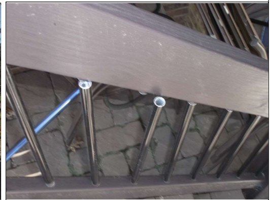
Balusters detaching from stair railing
