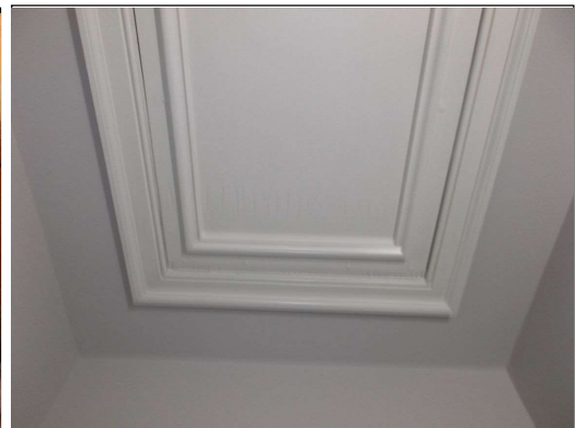
Paint blistered at pulldown attic door
