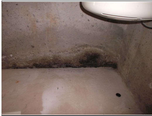
Stains inside the basement wall
