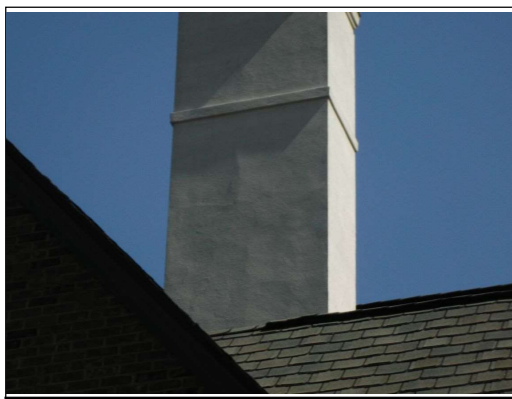
Bulge cracks in chimney stucco
