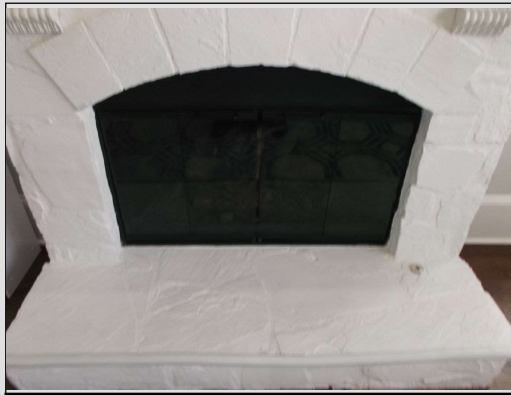
Fireplace doors defective
