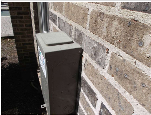
Missing bead of caulk over electrical boxes
