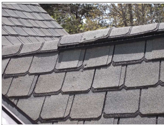
Holes in in roof shingles seen from bed
