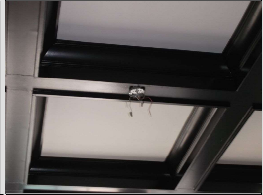
Missing light fixture at parlor
