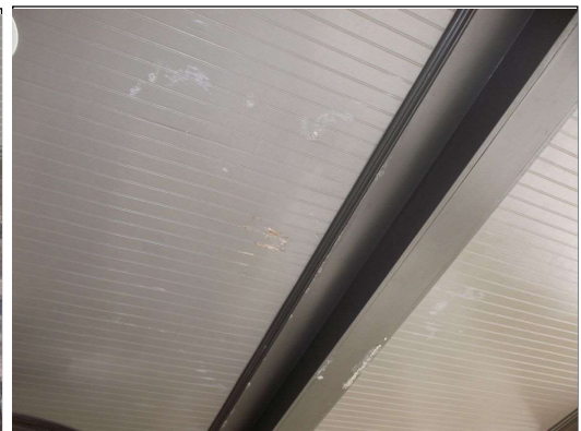
Possible water intrusion at patio ceiling
