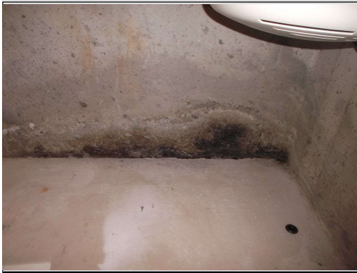
Stains on wall at utility room side of house
