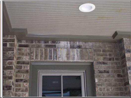
Calcium deposits on basement patio brick
