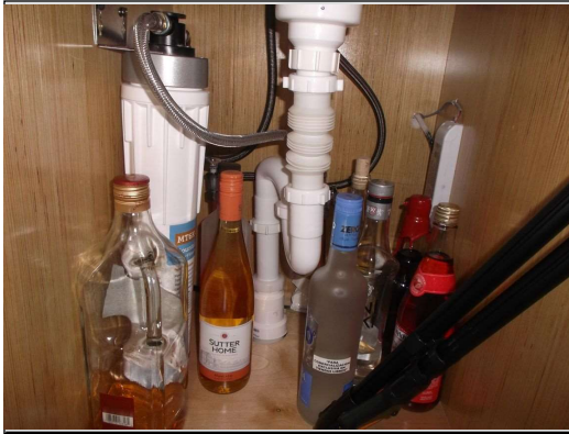
S-Trap under bar sink
