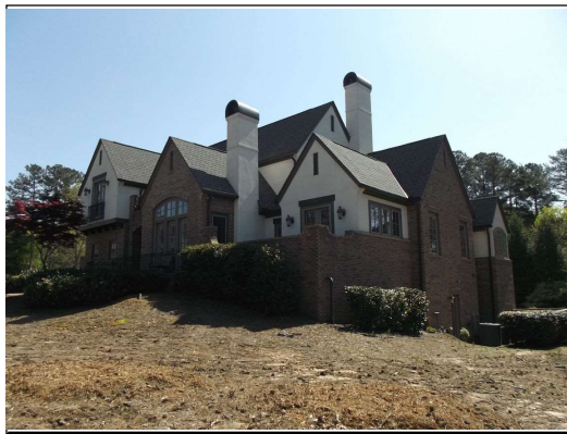
Front chimney leans to the left
