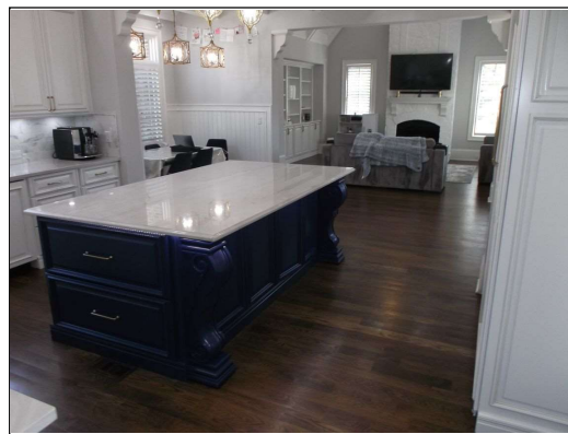
Kitchen floor settling at island
