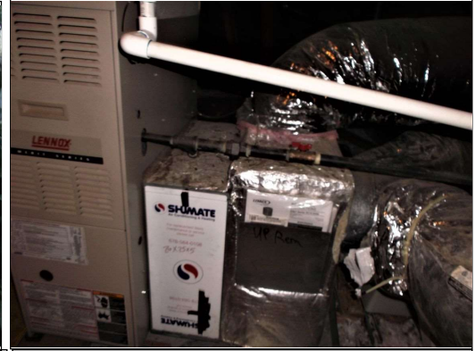
Improper sediment trap @ gas pipe to furnace
