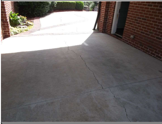
Moderate crack in driveway
