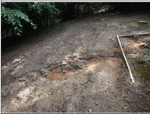
Missing ground cover &amp; soil erosion rear yard
