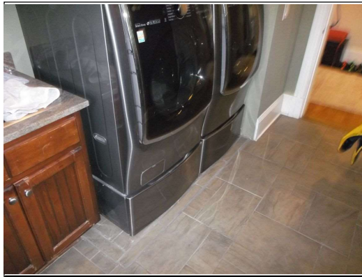
No washer drain pan installed
