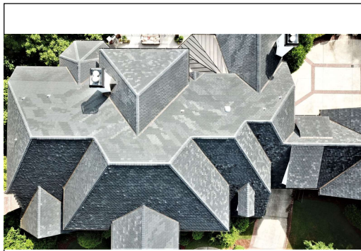
Defective shingles throughout roof system
