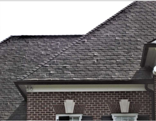
Shingles near end of use
