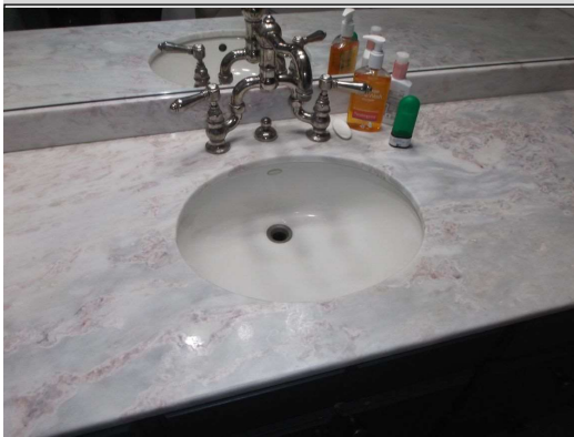
Sink stopper missing
