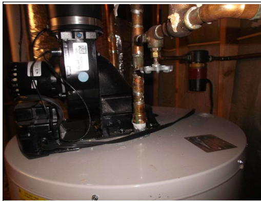
Copper &amp; steel pipe join above water
