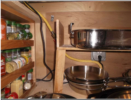
Cannot see a gas regulator valve in cabinet
