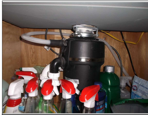
Dishwasher drain pipe not high looped up
