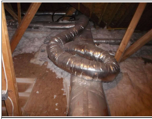
Air duct too long, too many turns
