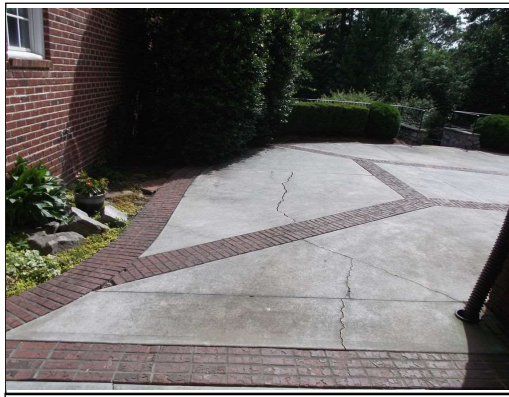
Driveway has moderate crack/slope to house
