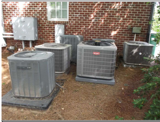
6 AC units on the right side of garage
