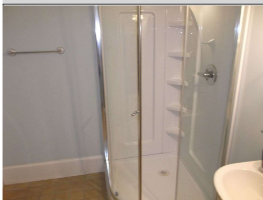
Shower door defective opening and closing
