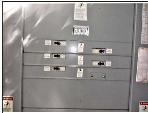
Five 200 watt breakers in main panel
