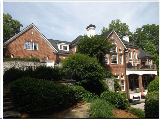
Shingles on rear roof lifting and curling
