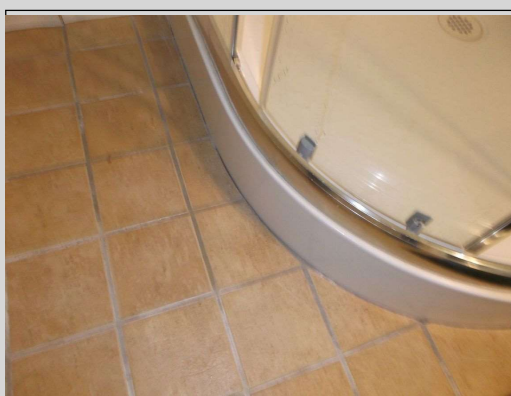
Missing caulk at the shower base and tile
