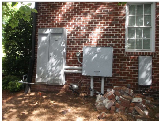
Main panels side of garage 5x200 watt breake
