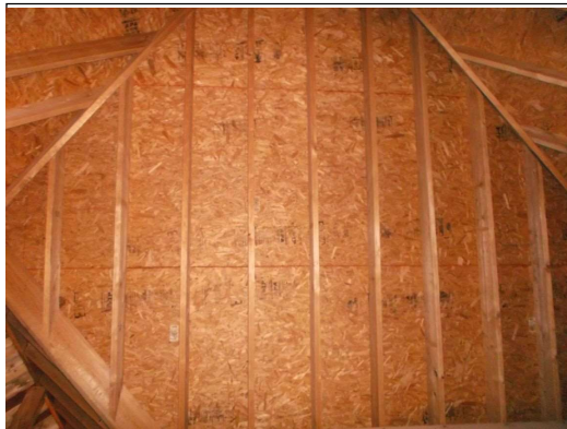
Missing ply board spacer clips between panel
