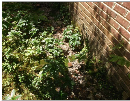
Soil erosion at the rear of the house no gutter
