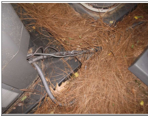
Refrigerant line insulation missing
