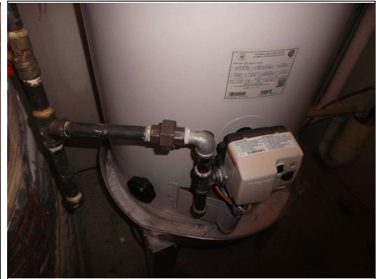
Water pipe elbow in gas pipe @ W/H
