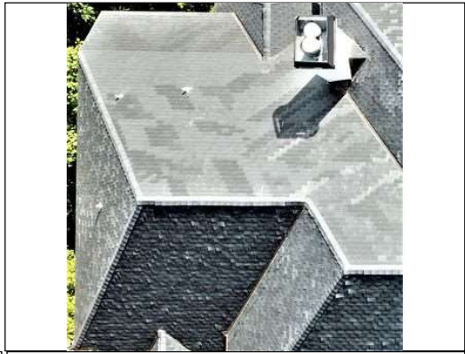
Missing gutter left side and rear left of house
