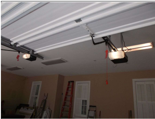
Lights not illuminating garage/globe missing
