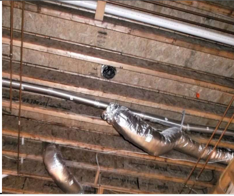
Air duct disconnected in basement ceiling
