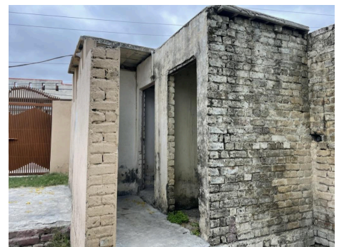
Toilet block needs renovation and enlargement
