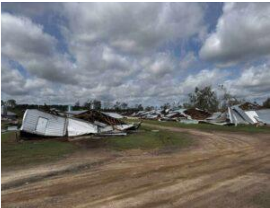
Collapsed poultry houses in Coffee County
