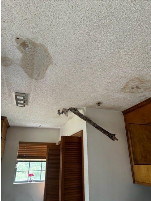
Tree branch coming out of a ceiling in an Augusta home
