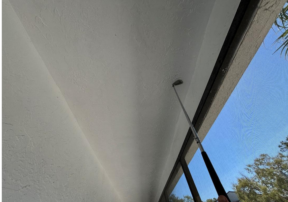
Figure 11: Apparent delamination at soffit, Unit 204. Building 4.
