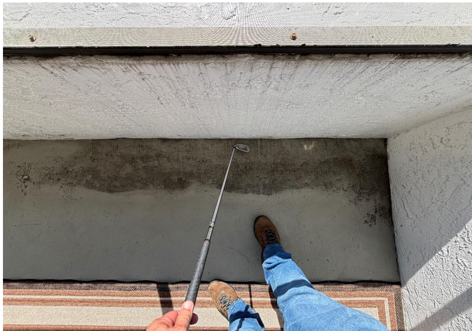
Figure 2: Localized apparent delamination at balcony slab, Unit 209 Building 2.
