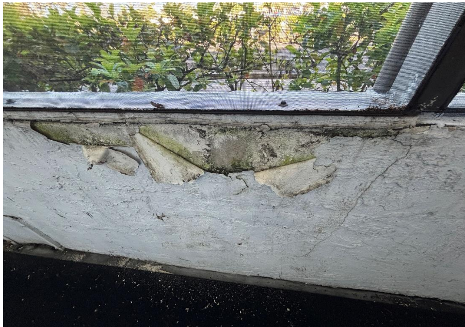
Figure 4: Moisture-related deterioration at balcony knee wall (typical condition) - Building 2.
