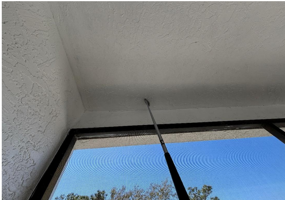
Figure 12: Apparent delamination at soffit, Unit 208. Building 4
