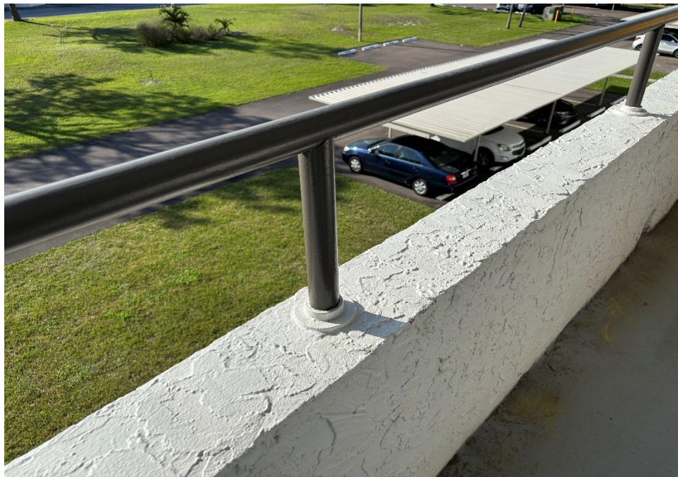
Figure 6: Balcony guardrail and connection condition, with no visible signs of distress or deterioration – Building 2.
