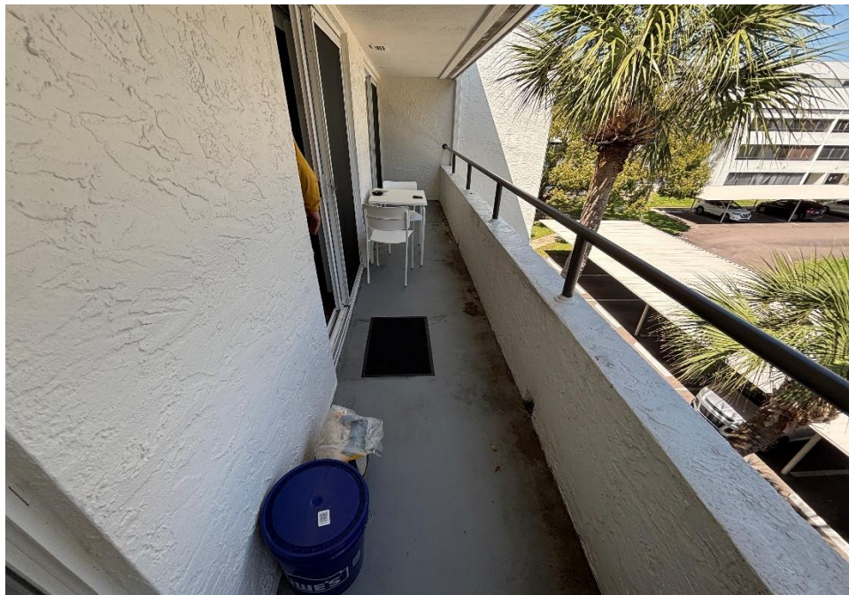
Figure 14: Typical balcony and guardrail condition showing no visible signs of distress or deterioration – Building 4.
