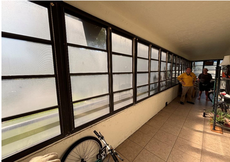
Figure 7: Typical balcony condition with tile finish, limiting direct observation of the underlying structural slab – Building 2.
