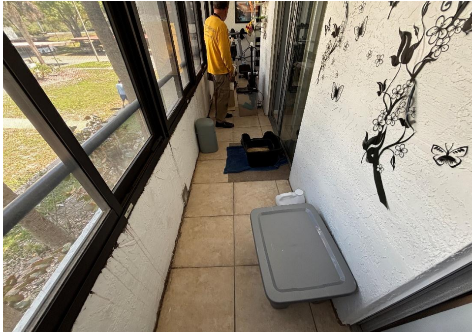
Figure 15: Typical balcony condition with tile finish, limiting direct observation of the underlying structural slab – Building 4.
