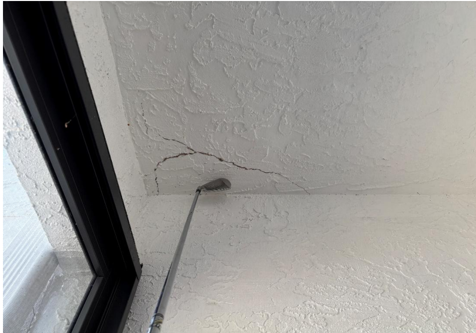
Figure 13: Minor hairline cracking observed at ceiling, consistent with typical age-related conditions – Building 4.
