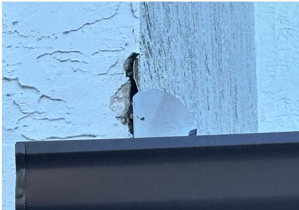
Figure 16: Localized surface damage with material loss at wall corner at west entrance – Building 2.
