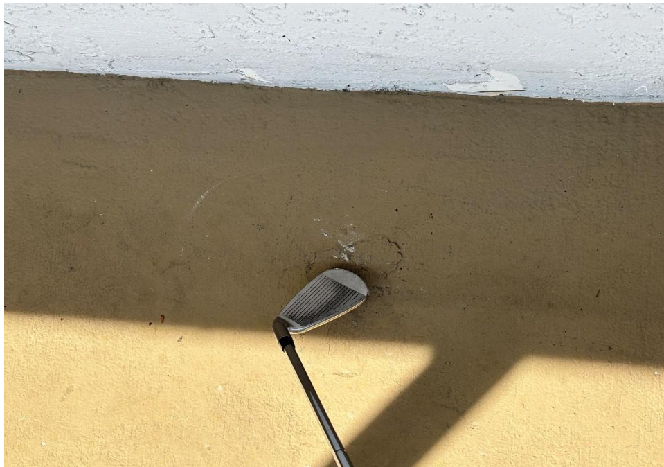
Figure 10: Localized apparent spall at balcony slab, Unit 301 Building 4.
