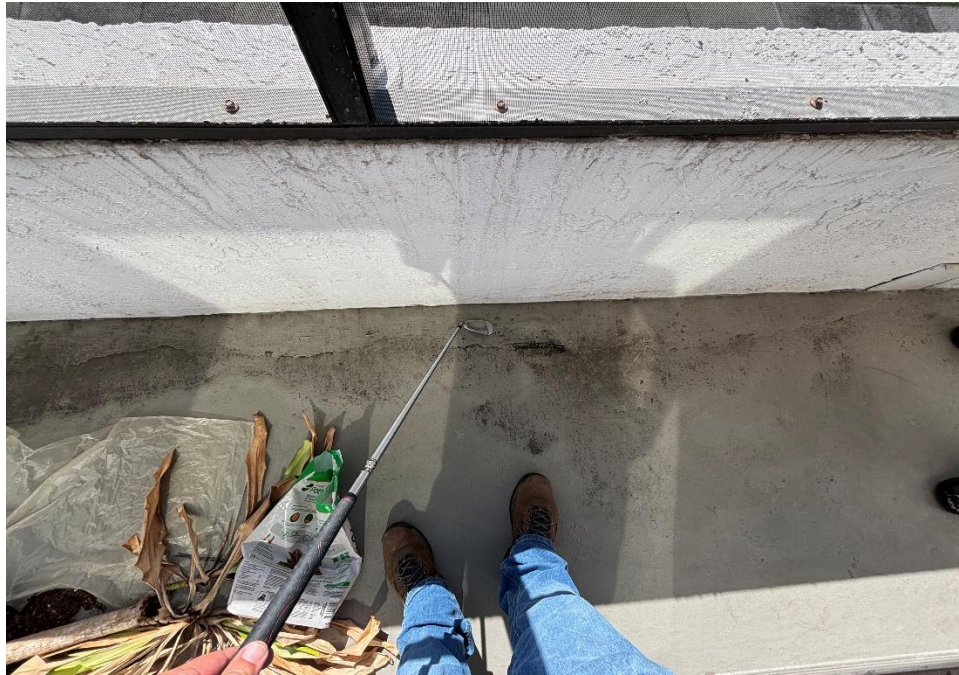
Figure 3: Localized apparent delamination at balcony slab, Unit 209 Building 2.
