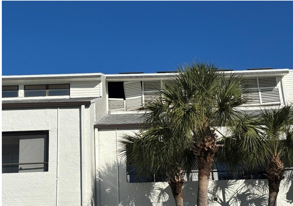
Figure 17: Displaced or missing louver panel at attic ventilation opening, east elevation – Building 2.
