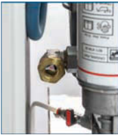
Oil Level Check
