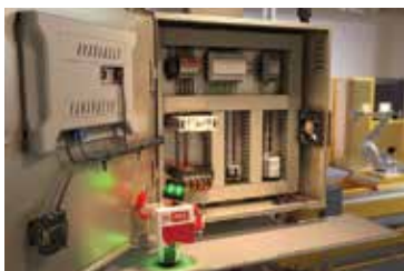
AUTOMATION AND CONTROL
