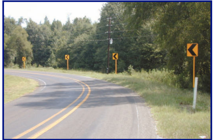
Chevron signs with retroreflective strips on sign posts installed along a curve. Source: FHWA
