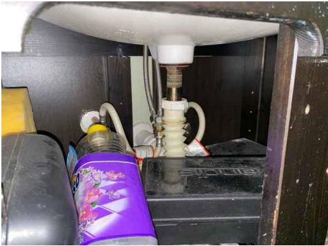
Bathroom (both water lines appear connected)
