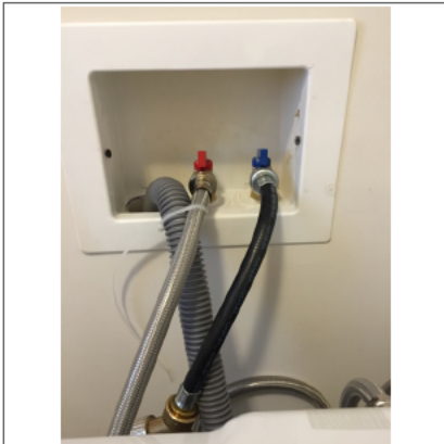
Rubber hose on cold water line
