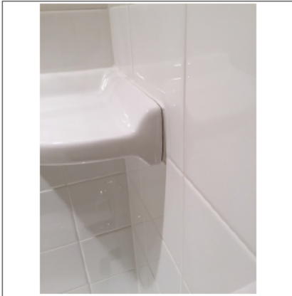
Soap shelf needs grout
