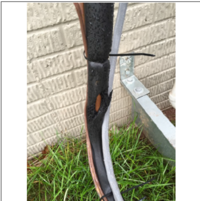
Damaged insulation on outside refrigerant line
