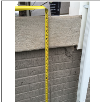
Porch height 41". Needs guard rail.
