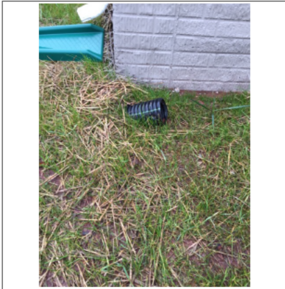
Foundation drains go uphill at ends
