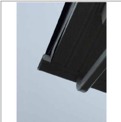
Fascia damaged over porch corner
