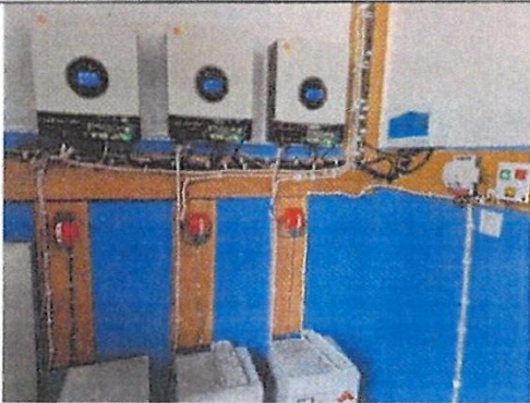
With solar batteries and inverters in place. Light shown!
