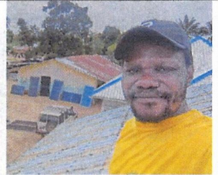
Pierre began solar panel installation on an older building, the new roof being too steep.
